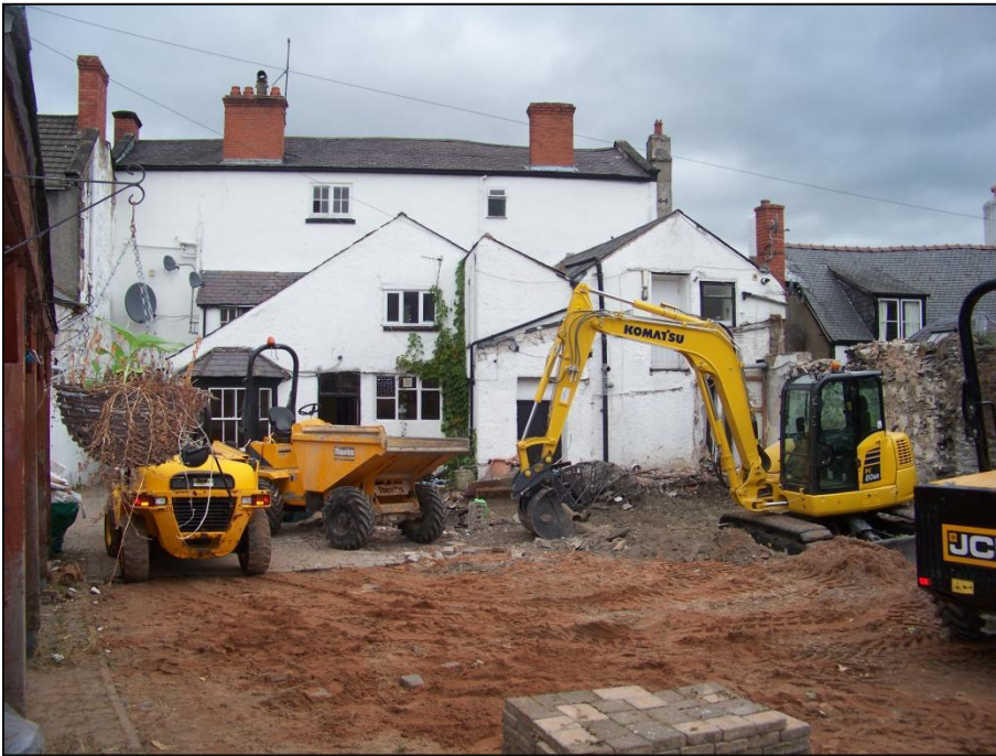
Plate 2: Looking NNE across the yard towards the rear elevation of the hotel following demolition of the kitchen. 15.08.18
