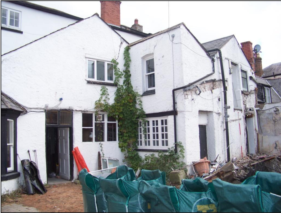
Plate 1: Looking NE towards the rear elevation of the hotel following demolition of the kitchen. 15.08.18
