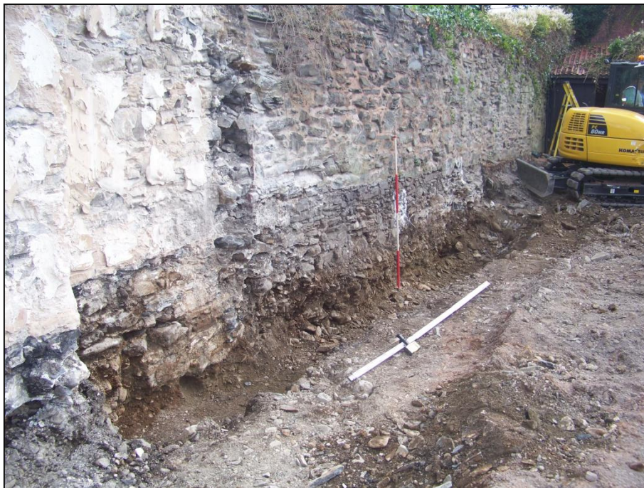
Plate 9: Eastern boundary wall foundations, following excavation and wall scar 4m south of hotel. 2m scale bar
