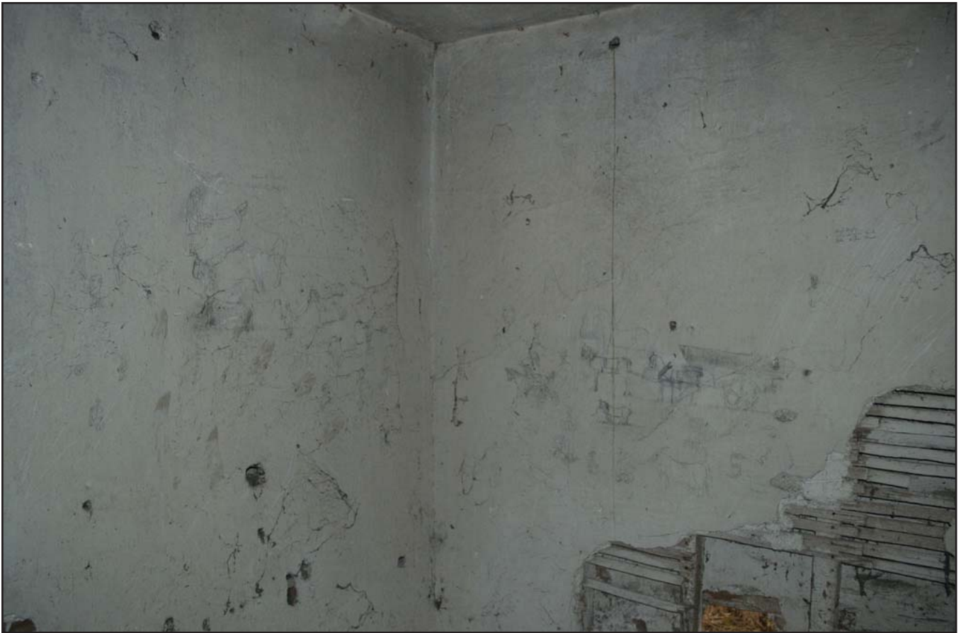
Plate 53: Graffiti on low quality lathe and plaster forming internal room upstairs. F03 Store (archive reference: G2479_090).
