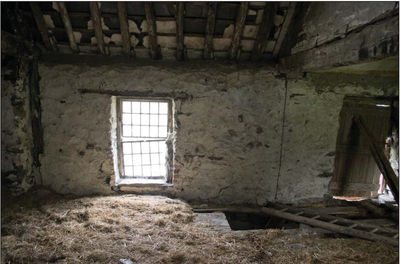
Plate 40: Central portion of SE internal elevation. Access point in floor F01 Hayloft (archive reference: G2479_077).
