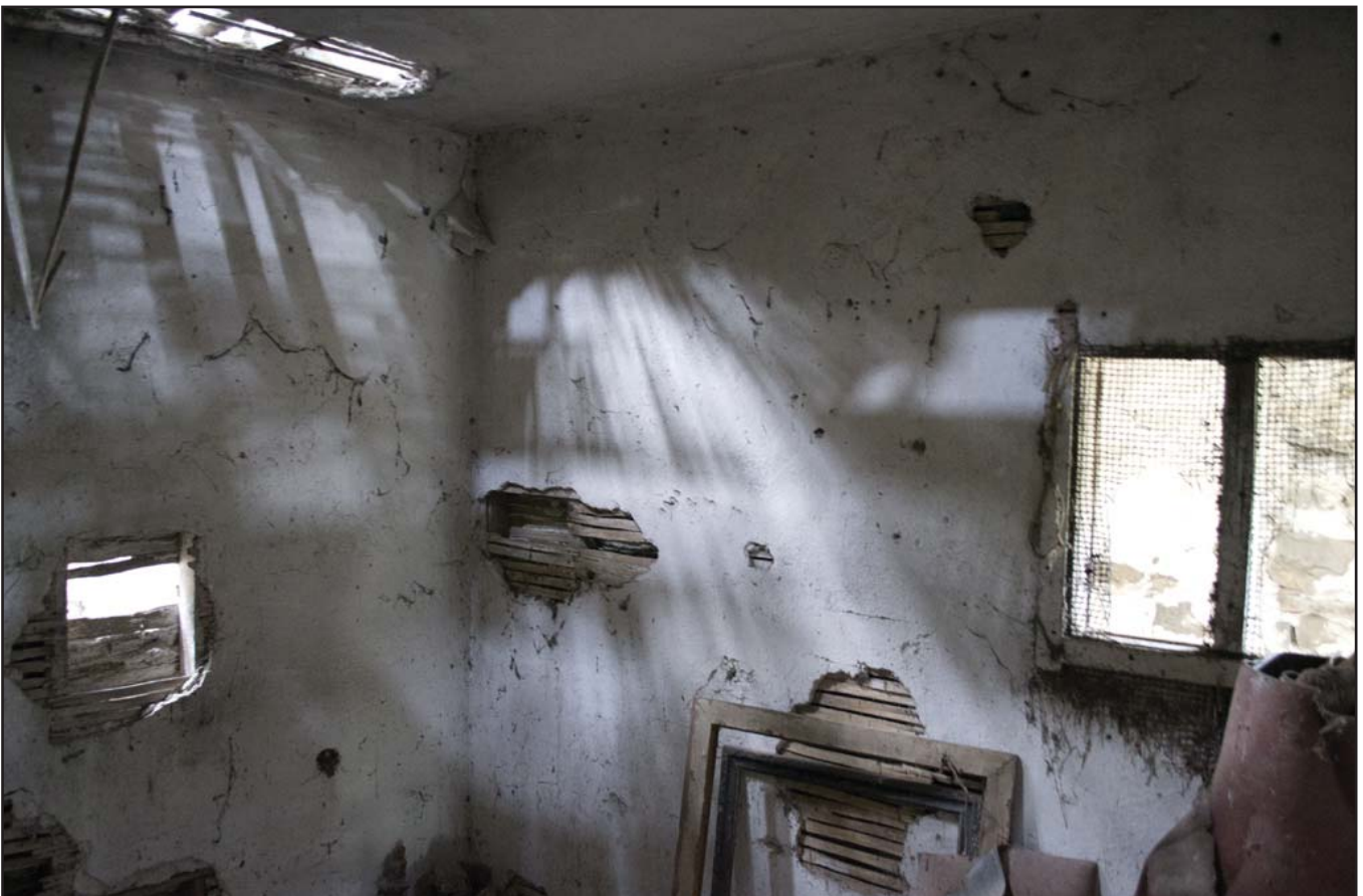
Plate 52: Low quality lathe and plaster forming internal room upstairs. F03 Store (archive reference: G2479_089).
