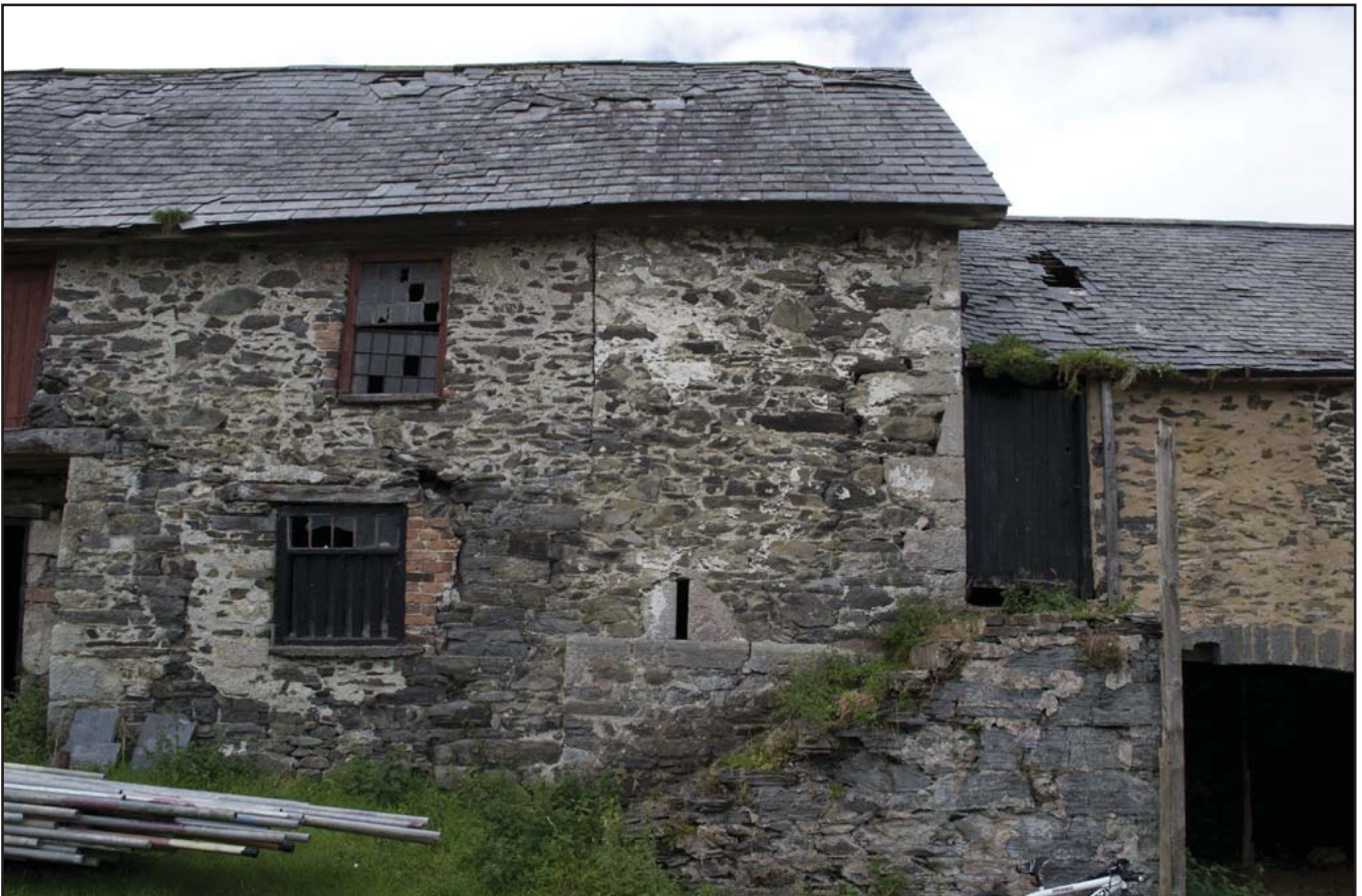
Plate 8: NE end of G01/F01 showing vertical crack and slit window (archive reference: G2479_030).
