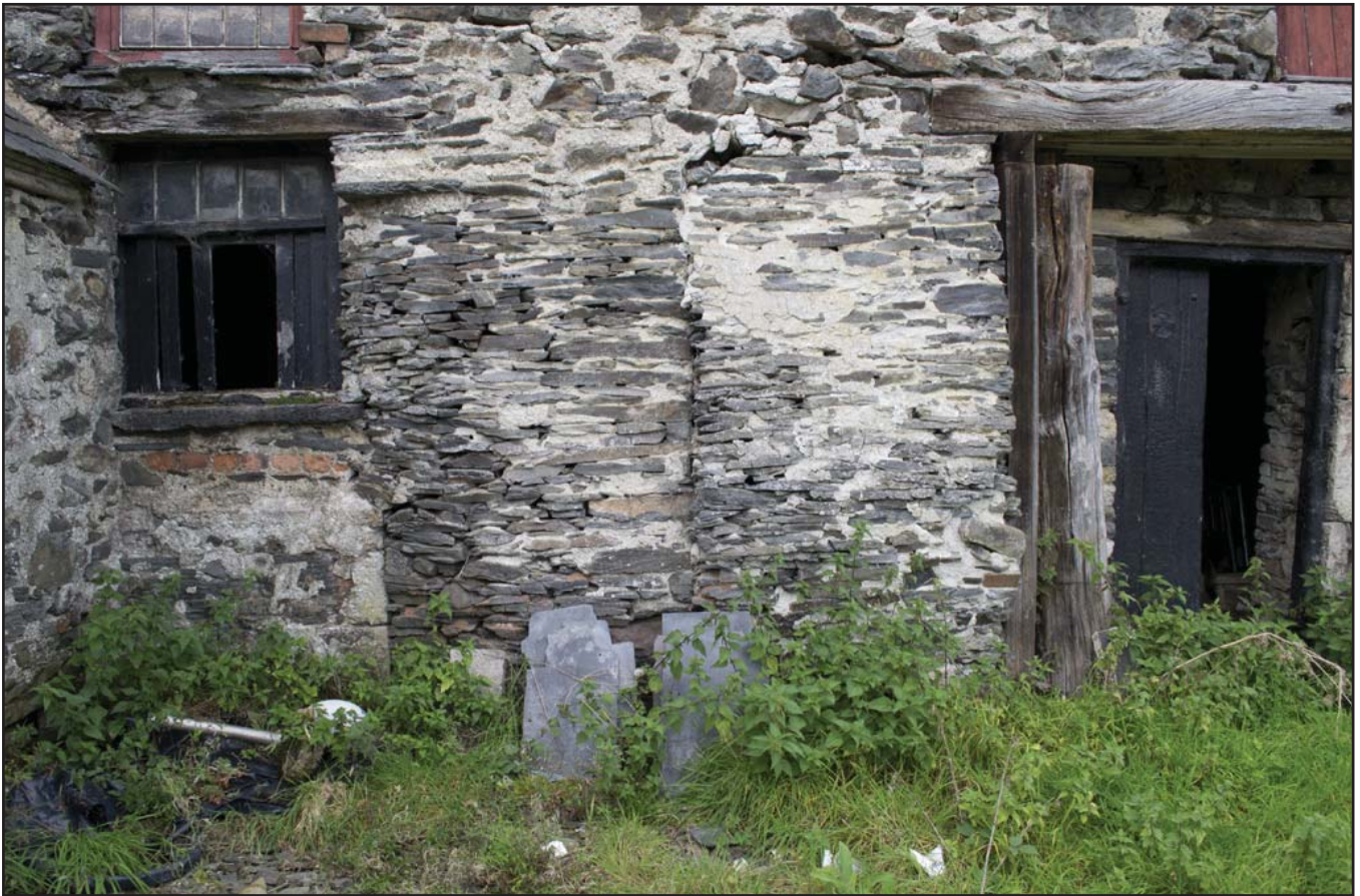
Plate 11: Collapsing repair between central door of G01 and Outbuilding G02 (archive reference: G2479_036).
