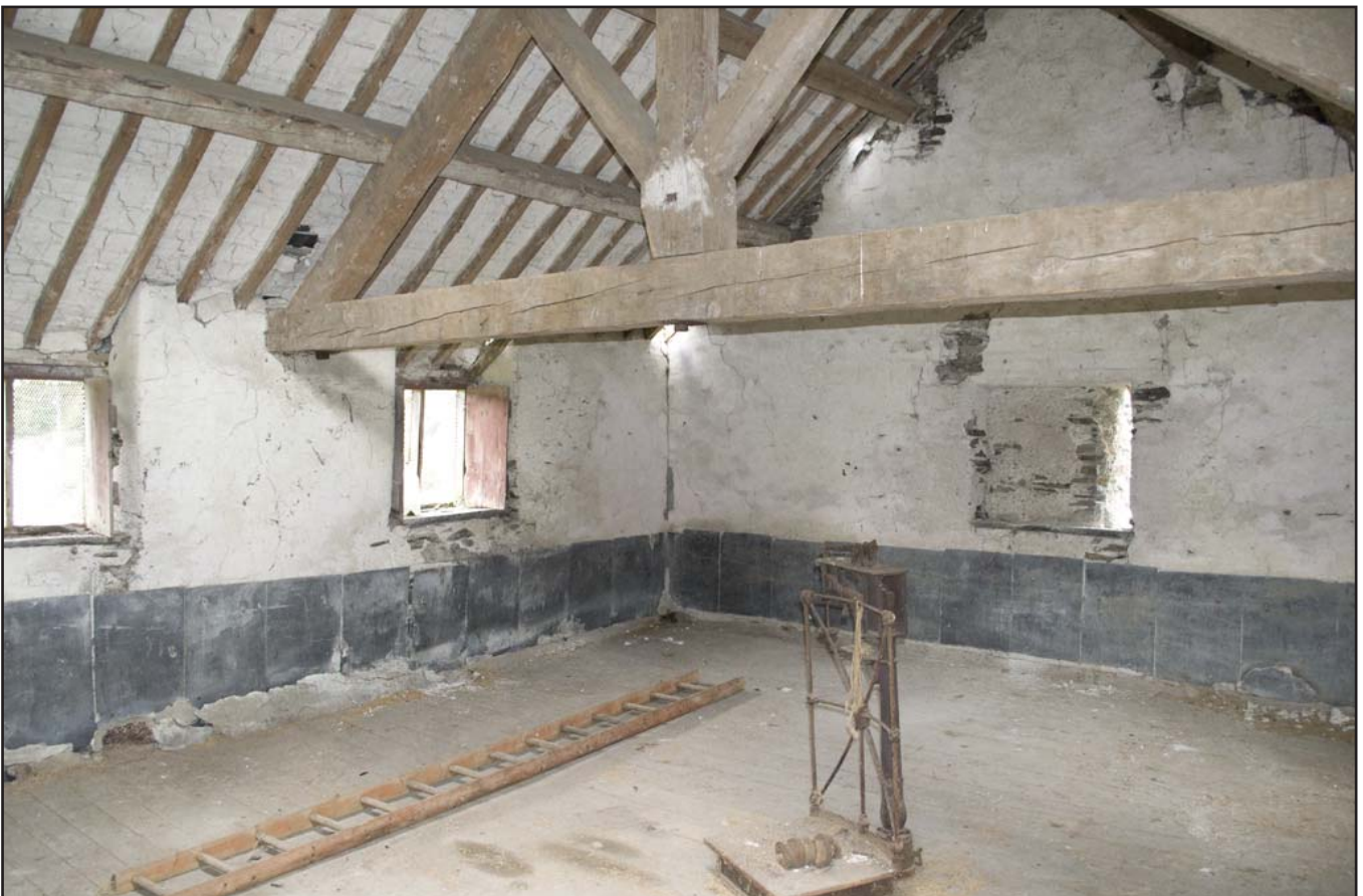
Plate 62: NE/NW elevation of Grain Store F04 - upper floor - (internal) (archive reference: G2479_021).
