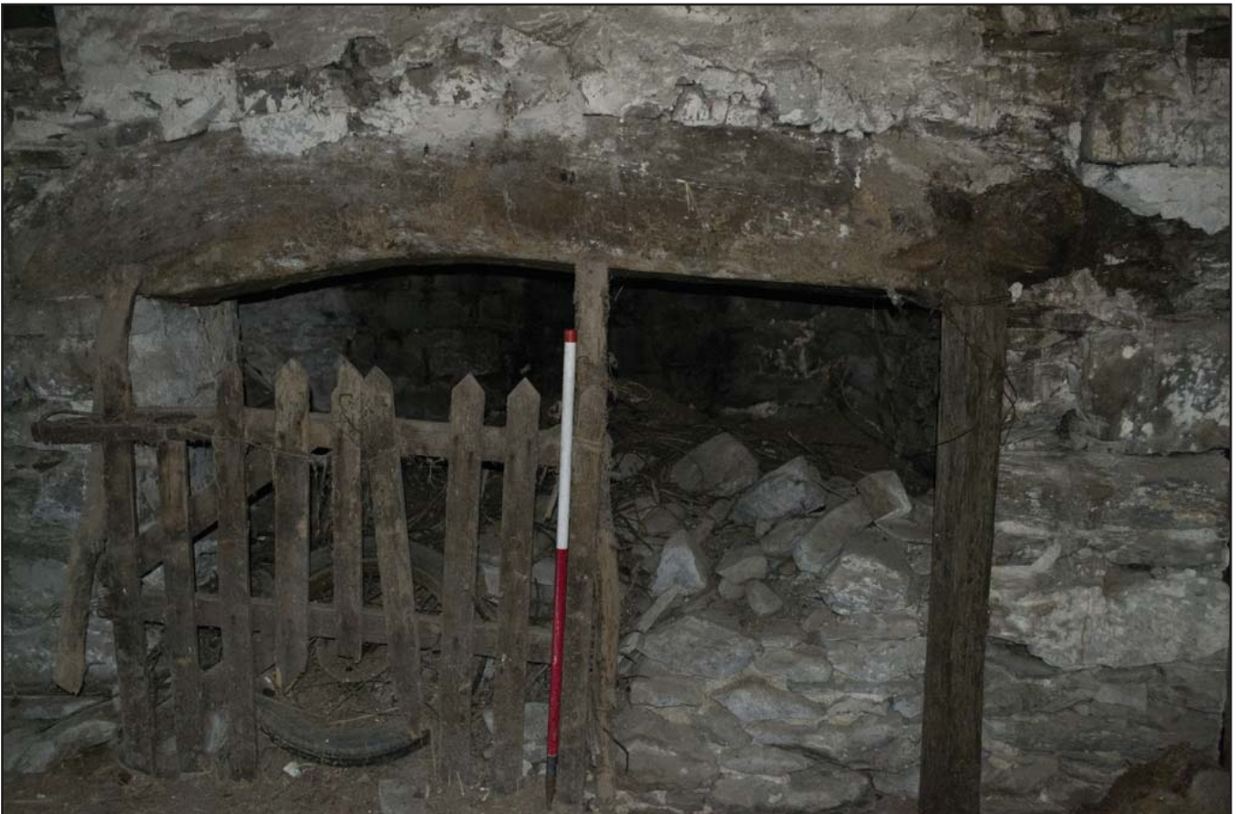
Plate 28: Chimney breast in end of building showing timber lintel above, reduction in width and built in oven on left of photo (G01); scale: 1x1m (archive reference: G2479_066).
