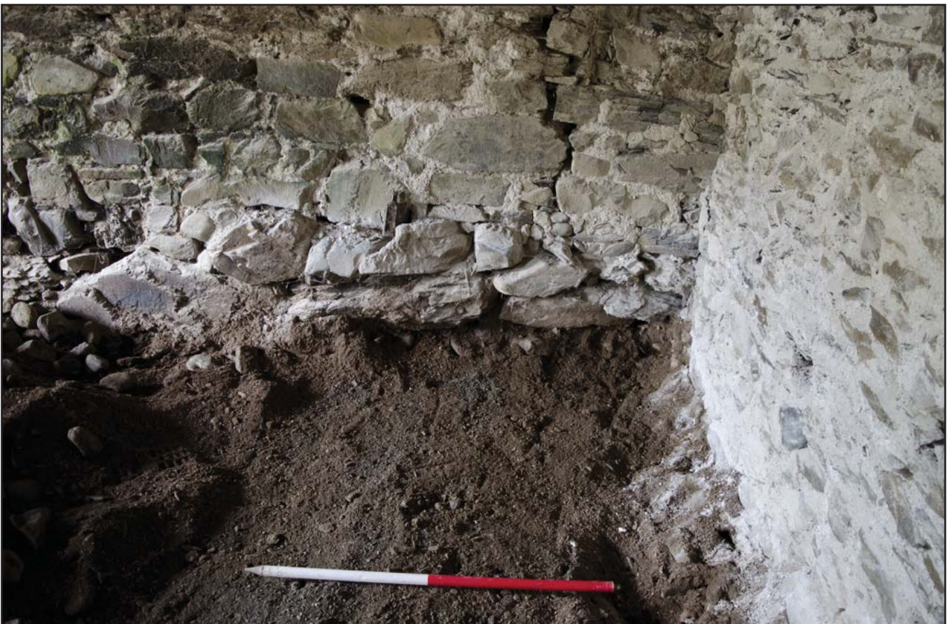
Plate 68: Cobbles lifted on S side of G04 Cart Shed showing depth of bedding gravel; scale: 1x1m (archive reference: G2479_201).
