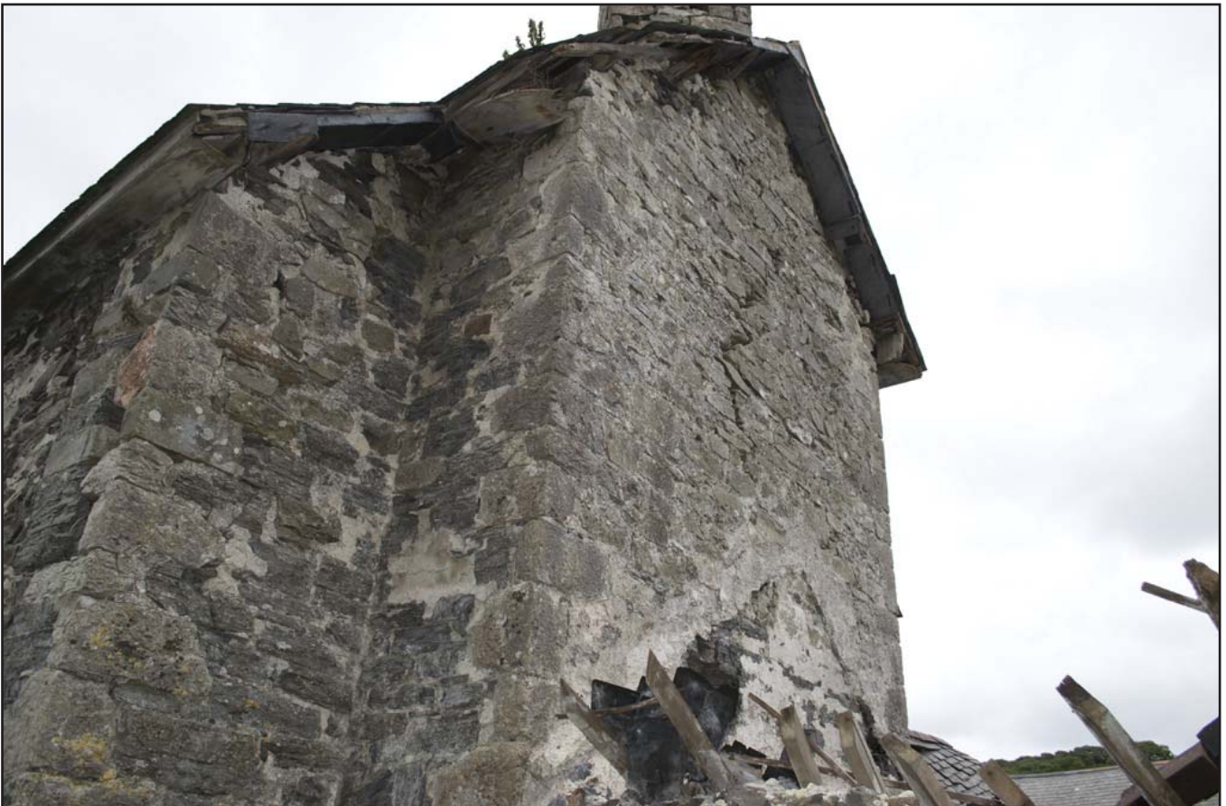
Plate 4: Chimney breast of G01/F01 showing scar of Outbuilding G02 and vertical crack in breast; (archive reference: G2479_046).
