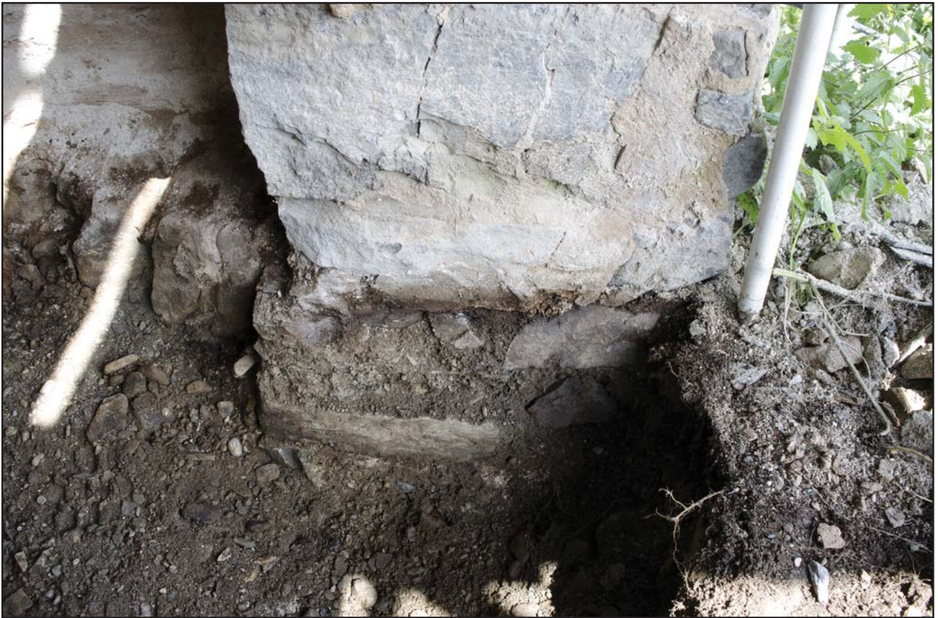
Plate 69: Cobbles lifted on N side of G04 Cart Shed showing base of wall of G04 Cart Shed; scale: 1x1m (archive reference: G2479_209).
