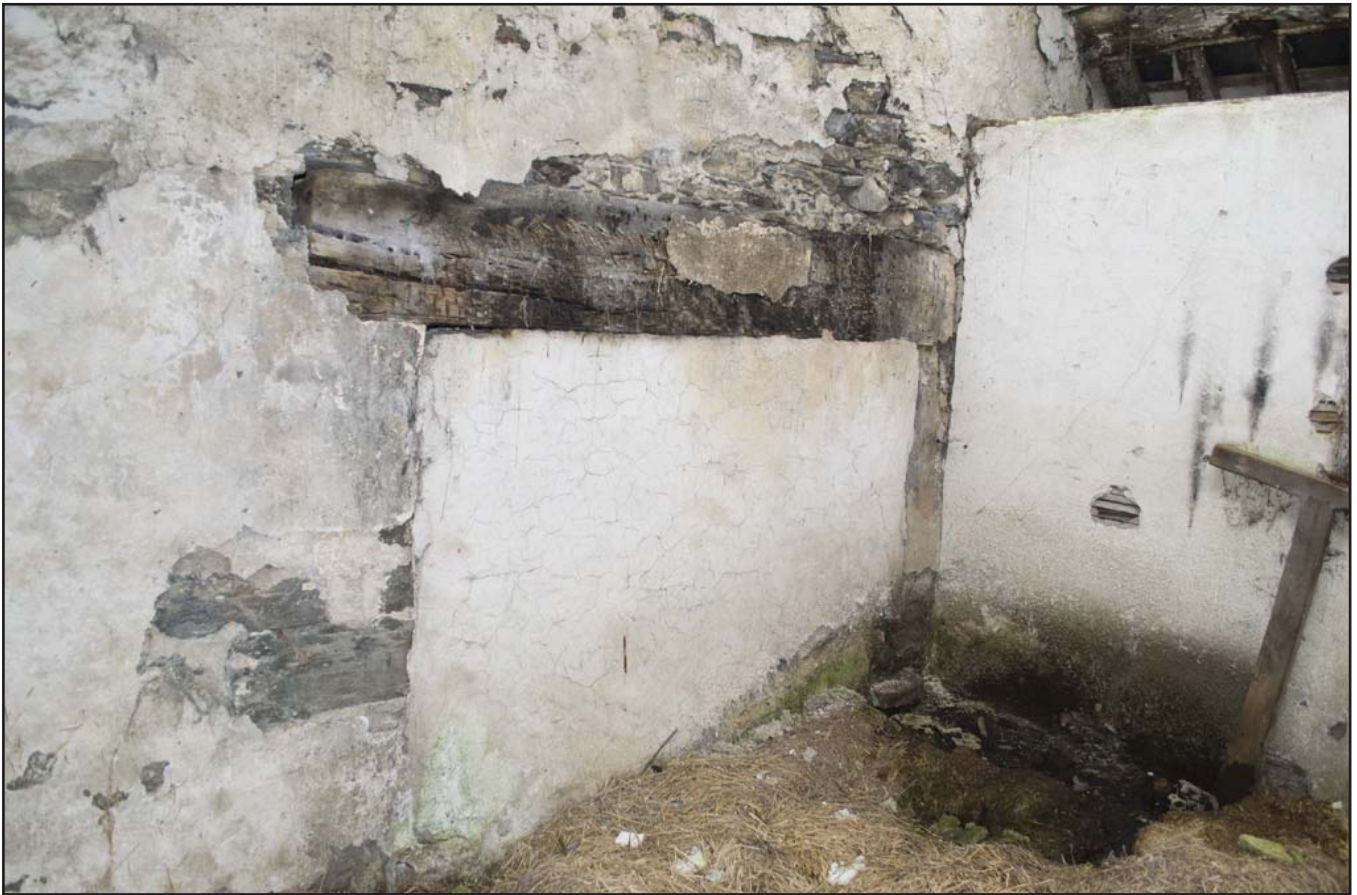
Plate 51: Blocked fireplace with internal still in place, low quality plaster. F02 Store (archive reference: G2479_093).
