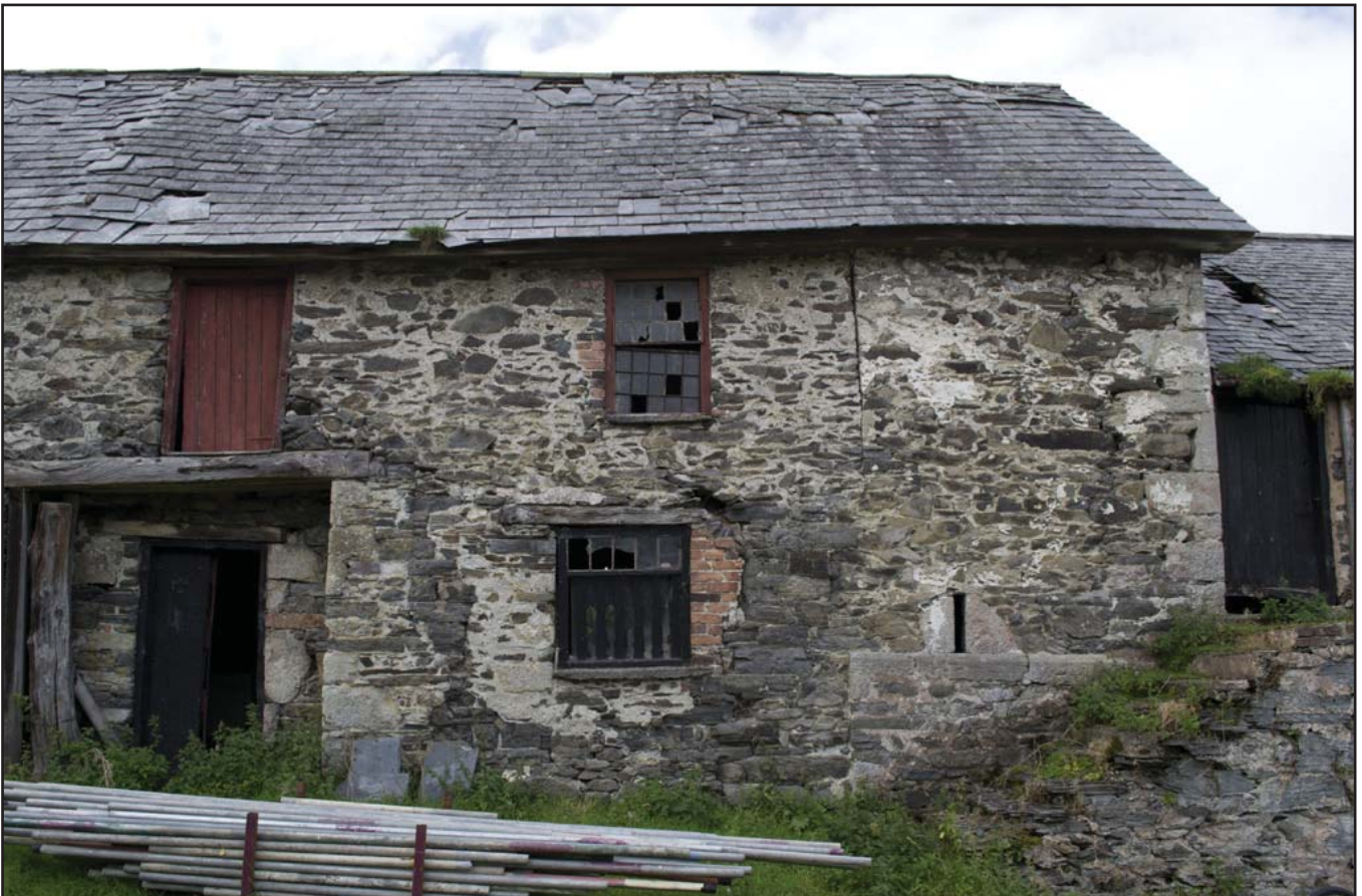
Plate 6: NE end of G01/F01 showing structural failings around ground floor window (archive reference: G2479_031).
