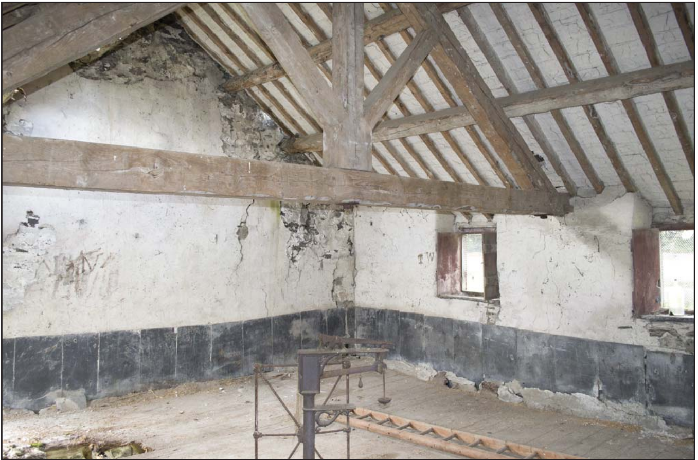
Plate 59: NW/SW elevation of Grain Store F04 - upper floor (internal) (archive reference: G2479_015).
