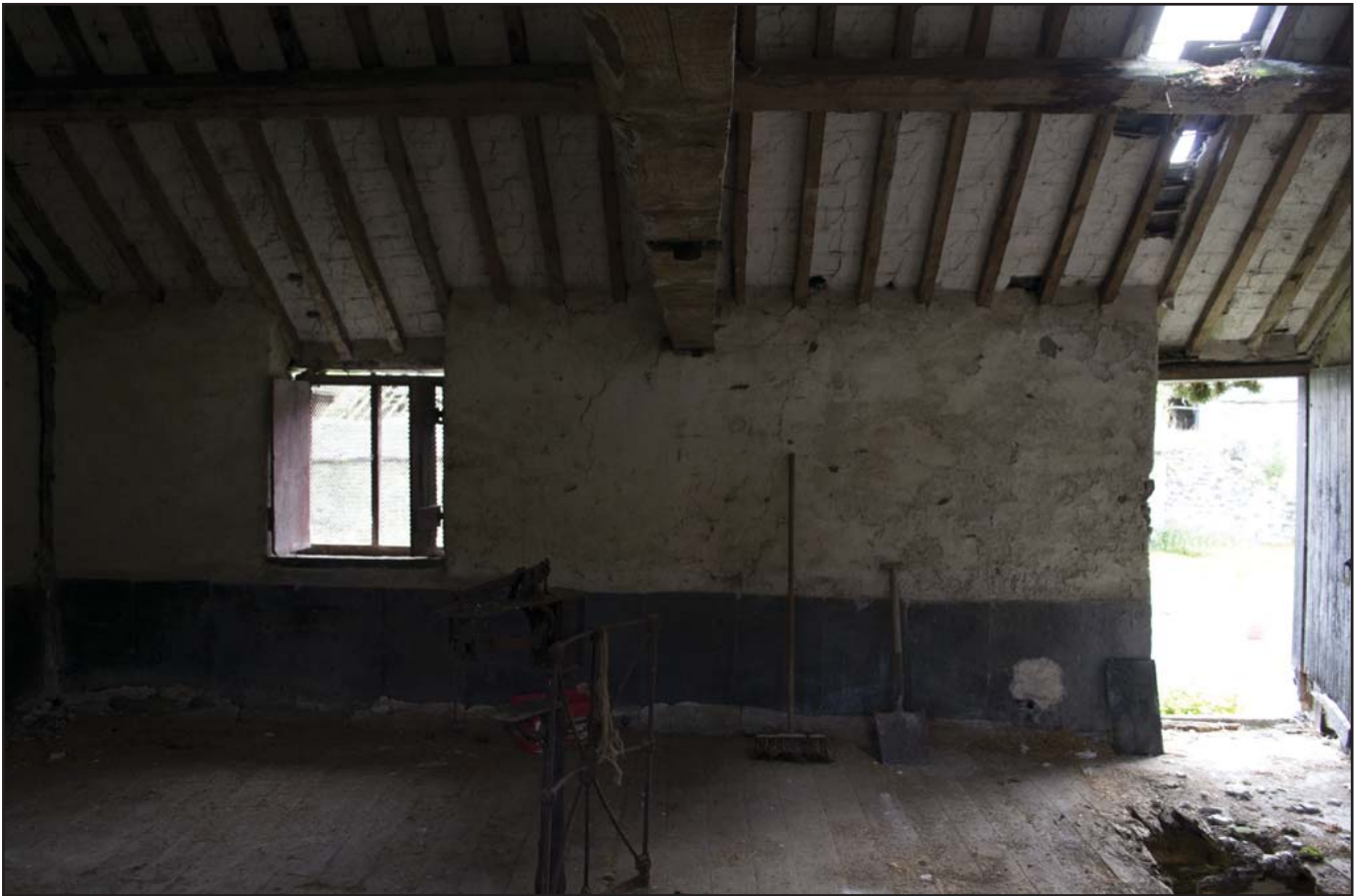
Plate 57: SE elevation of Grain Store F04 - upper floor - (internal) (archive reference: G2479_018).
