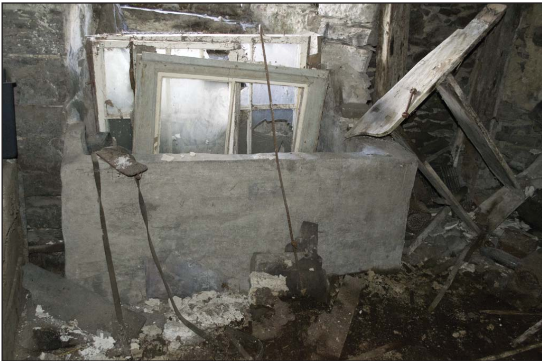
Plate 22: Rendered feed storage area built into window opening in G01 (archive reference: G2479_059).
