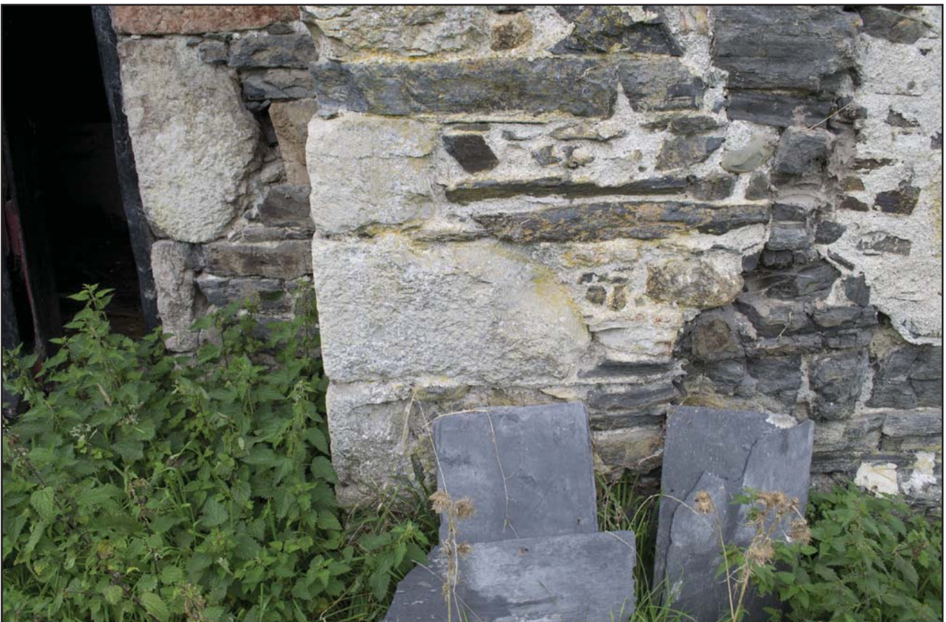
Plate 10: Limestone quoins visible in both inner and outer faces (G01) (archive reference: G2479_034).
