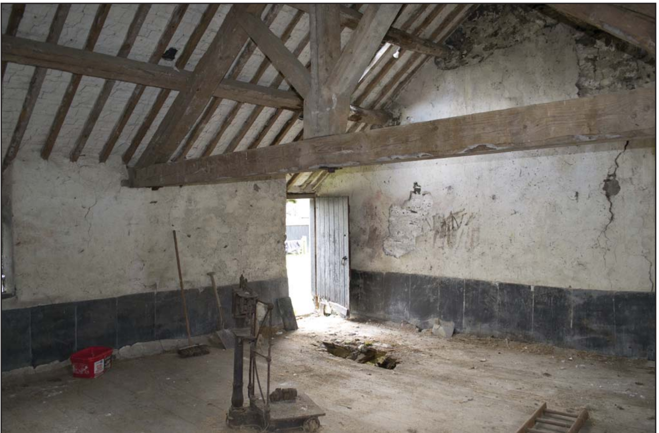
Plate 60: SW/SE elevation of Grain Store F04 - upper floor- (internal) (archive reference: G2479_017).
