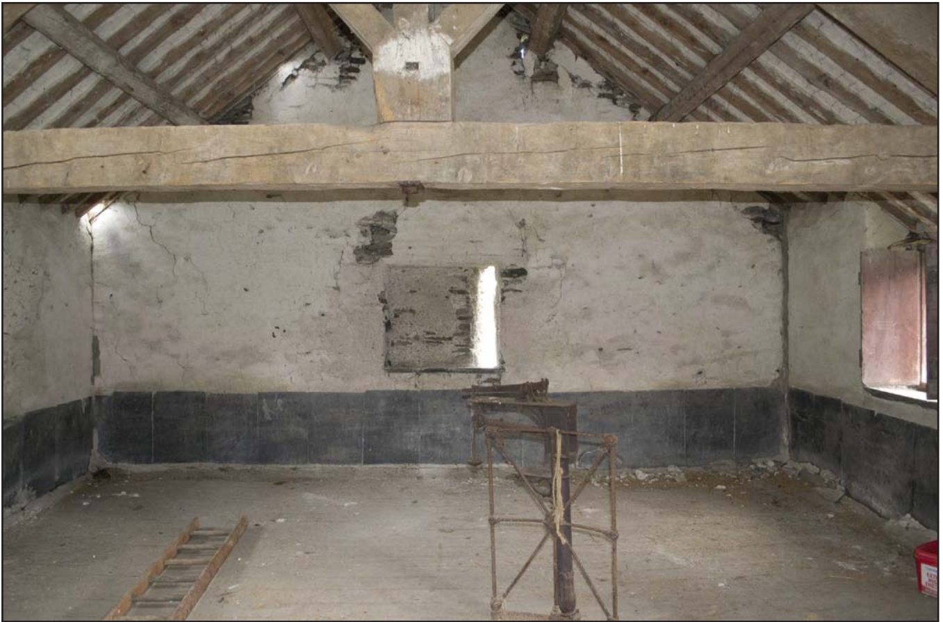
Plate 61: NE elevation of Grain Store F04 - upper floor - (internal) (archive reference: G2479_020).
