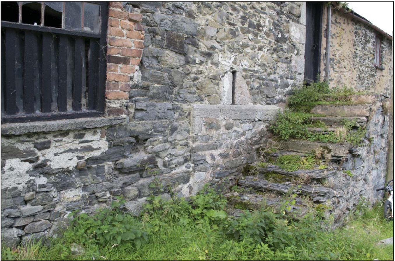
Plate 9: Relationship of external stairs, string course and structural failure (G01) (archive reference: G2479_033).
