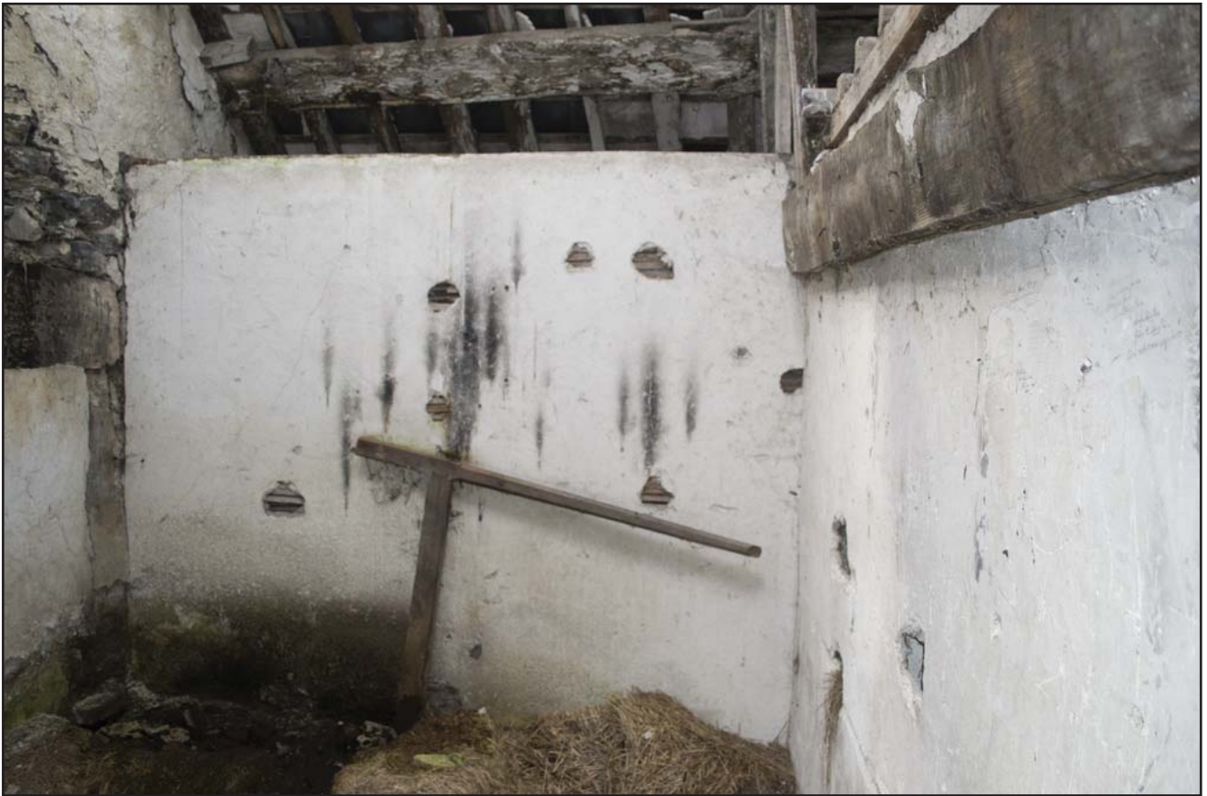
Plate 49: Low quality lathe and plaster wall forming corridor down NW side of building F02 Store (archive reference: G2479_092).
