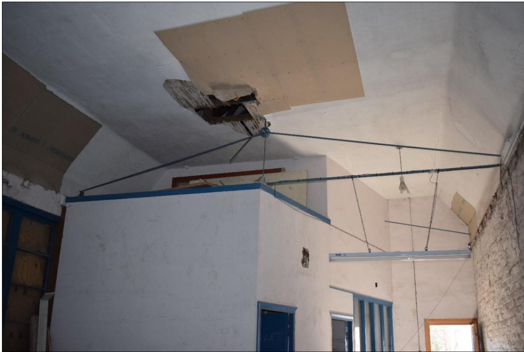
Fig. 7 The interior of the original building showing the iron bracing and later partitions. Photo CPAT 4634-0006
