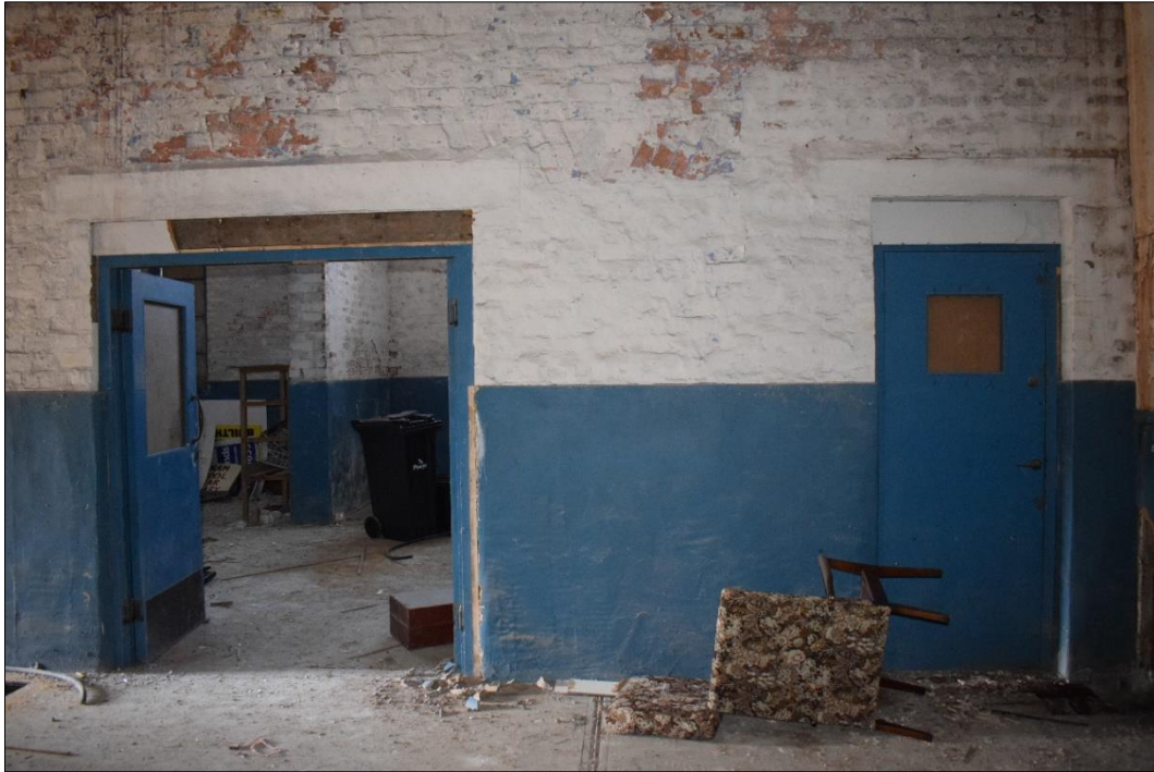
Fig. 5 The south wall of the original building showing the modern inserted doorways, with the voussoir of the blocked opening just visible between. Photo CPAT 4634-0019
