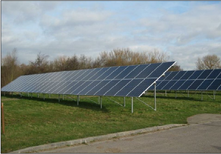
Typical solar array
