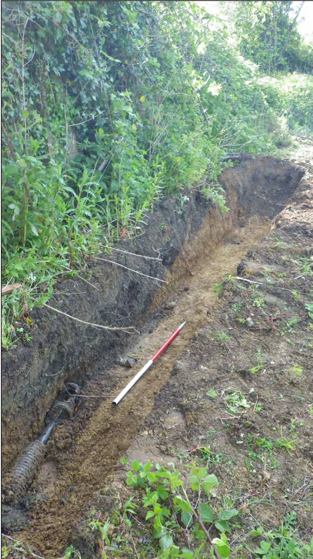
Plate 13: RWH2013_113 Excavated trench showing cut for modern pipe and subsoil, looking west.
