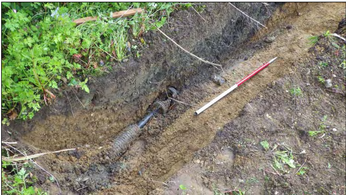
Plate 12: RWH2013_112 Southeastern end of the trench showing the modern pipe running across the side of it, looking west.
