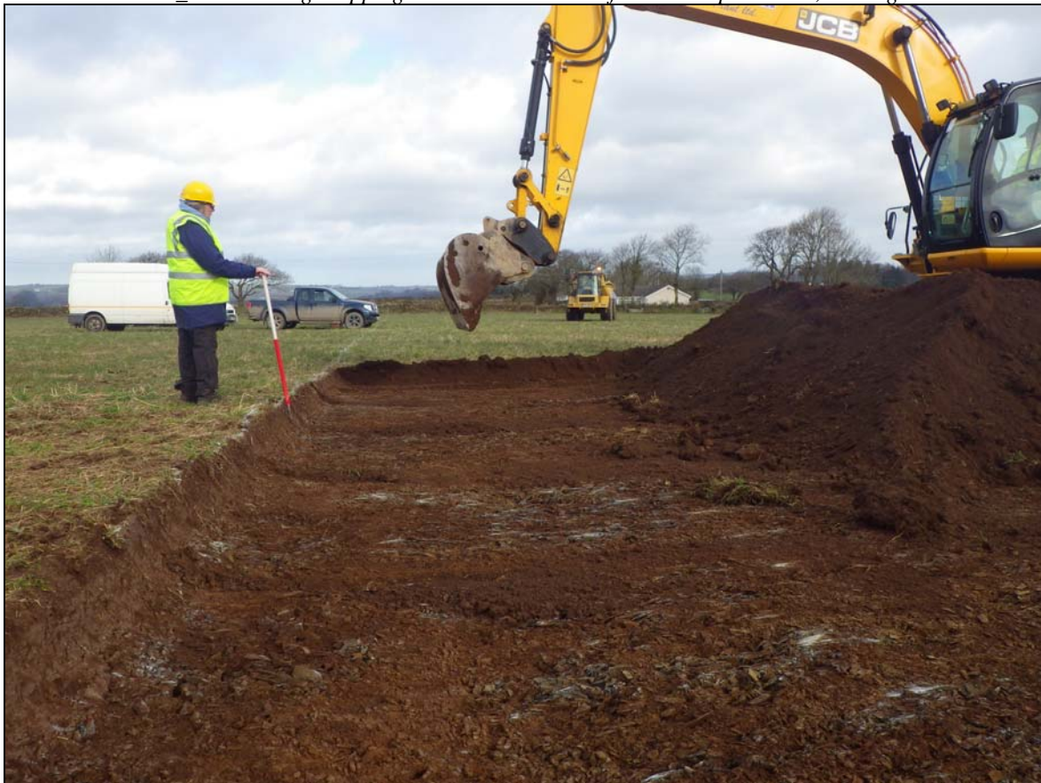
Plate 2: TNB2015_102: Stripping the development area, looking north northwest, bedrock visible in places
