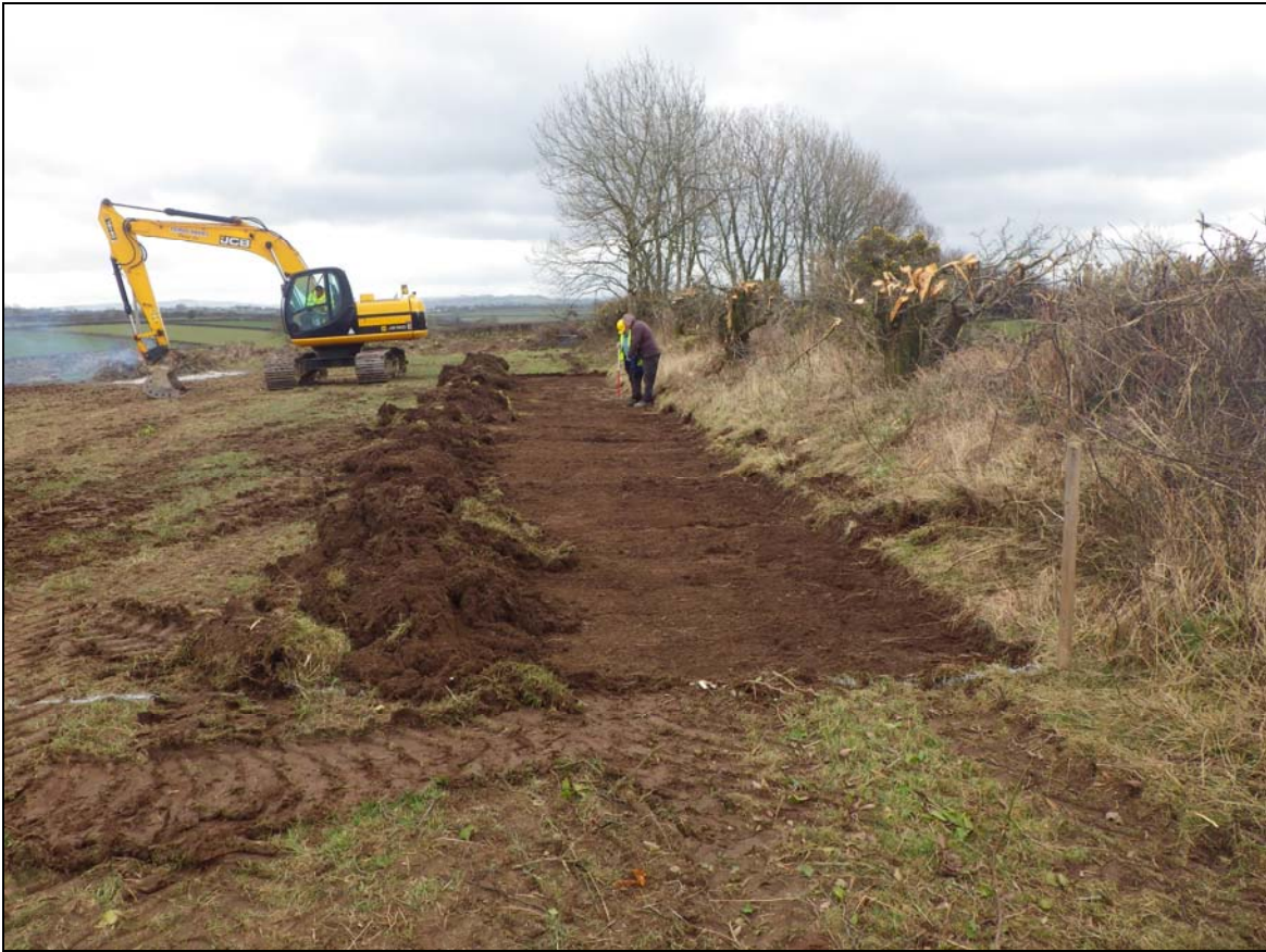
Plate 1: TNB2015_101: Starting stripping at the southern end of the development site, looking east
