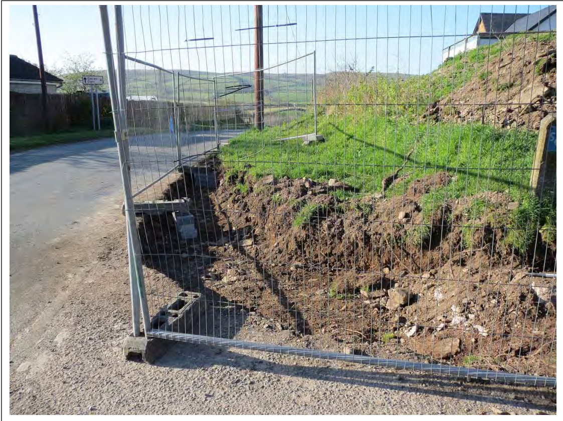
Plate 5. General shot of the excavation at the north-east corner of the site, showing stone rubble (24) below the topsoil (20). Looking South.
