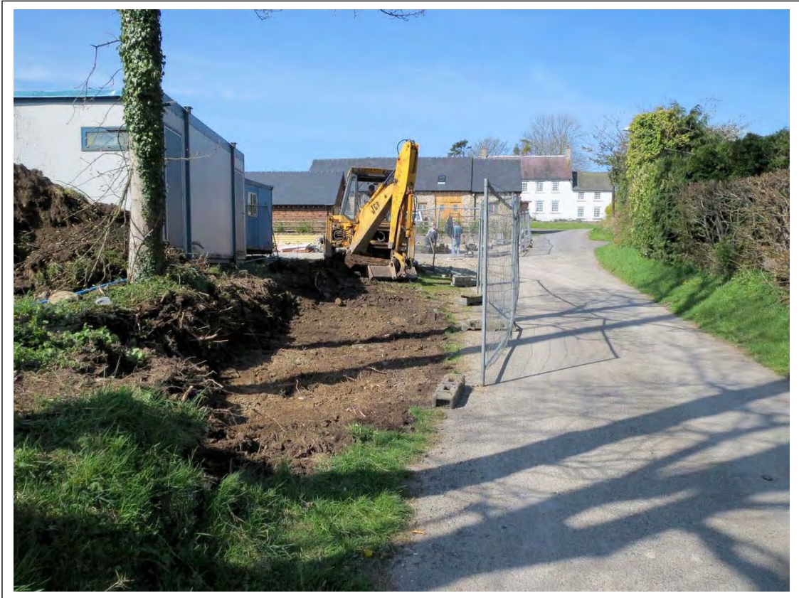
Plate 1. Working shot of the machine excavation, stripping topsoil (20) along the northern perimeter of the development site. Cruck Barn (built in stone) and Castle Farm (rendered and whitewashed) are shown in the background. Looking West.
