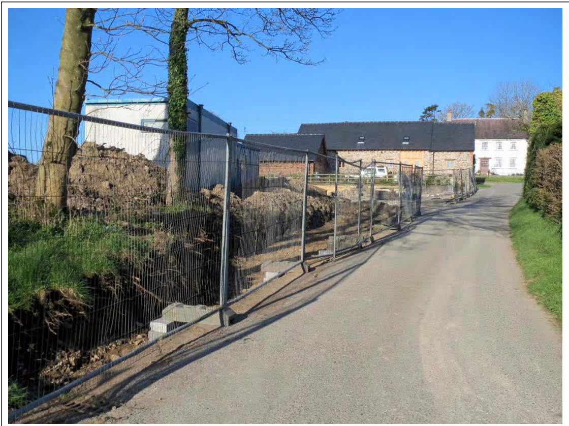
Plate 4. General shot of the excavation along the northern site boundary following the soil strip. Looking West-South-West.
