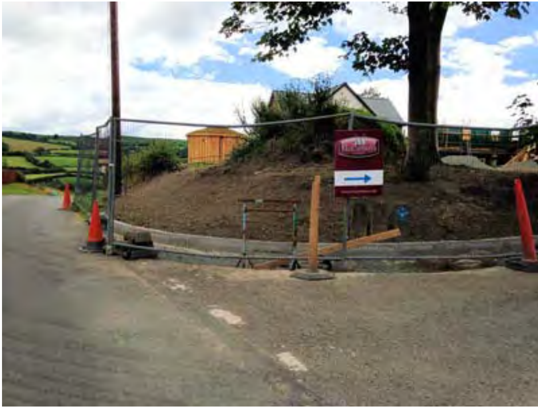
Plate 21. View of the new road kerb at the north-east corner of the site. The remains of the stone-built structure identified in this area have been left in situ below the reinstated bank. Looking South-South-West.
