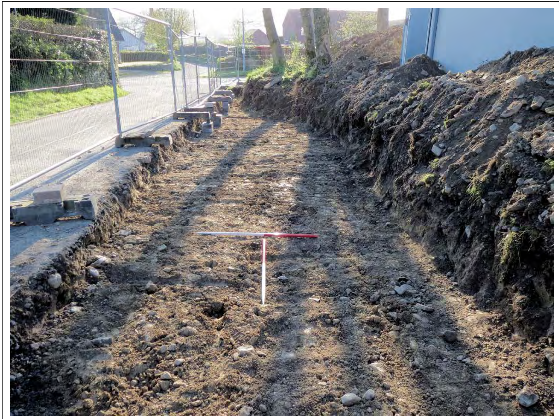
Plate 8. Post-excitation shot of the soil strip down to the silt subsoil (29) along the northern site boundary. Scales: 2 x 1m. Looking East.
