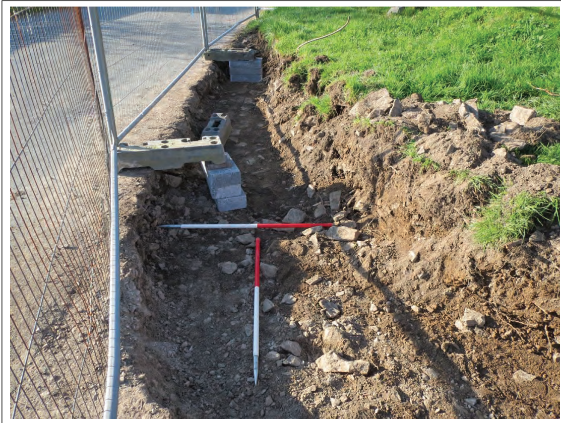
Plate 11. Post-excitation shot of the soil strip on the road junction at the north-east corner of the site, showing stone rubble (24) derived from the historic collapse or demolition of a post-medieval building (marked on the tithe map). Scales: 2 x 1m. Looking South.
