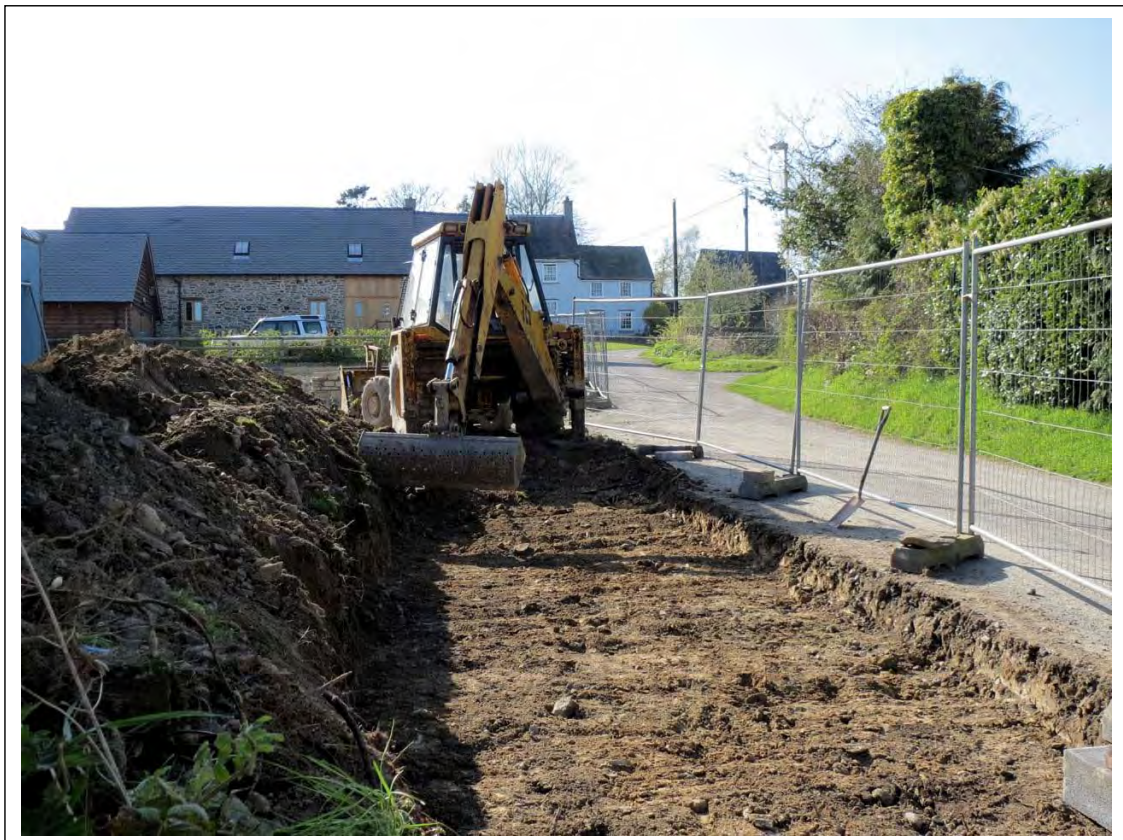
Plate 2. Working shot of the soil strip down to natural subsoil, a light grey-brown silt (29). Looking West.
