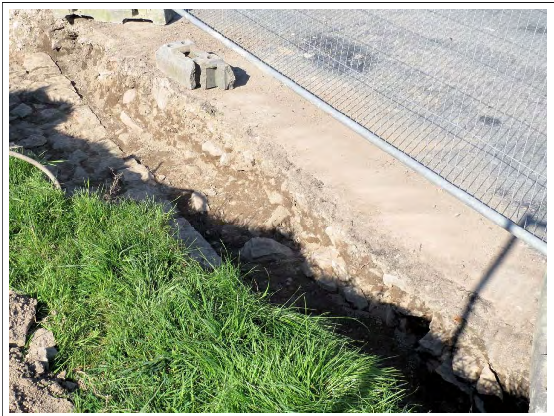
Plate 18. Oblique view of the road construction along the eastern site boundary, showing a layer of compacted stone (28) below the tarmac (21). Looking North-North-East.
