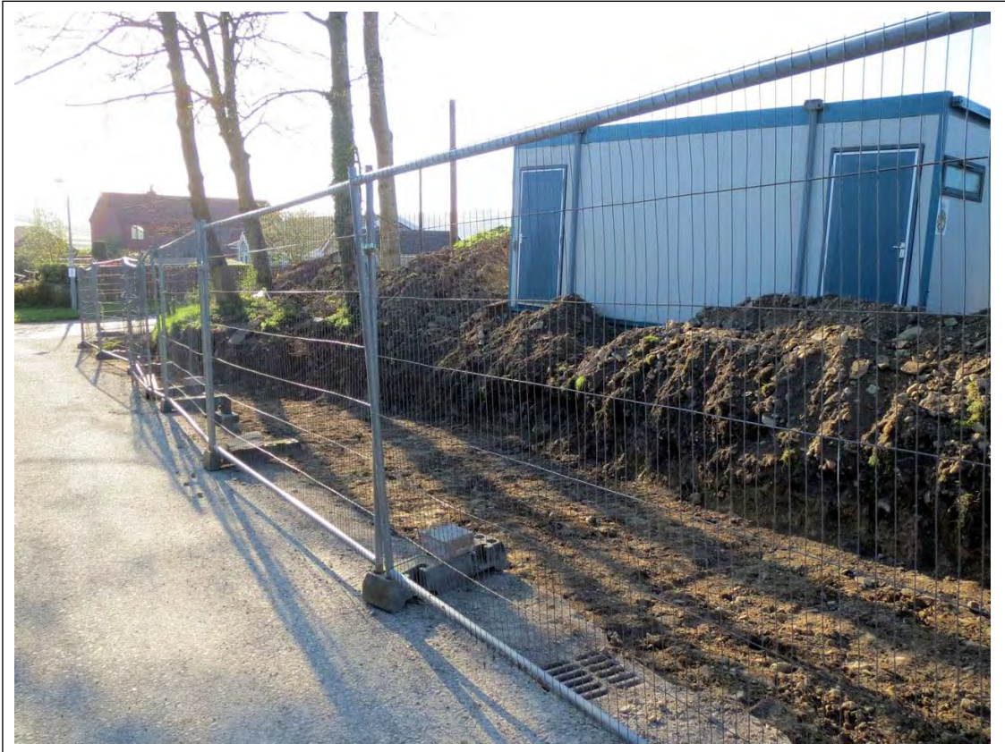
Plate 3. General shot of the excavation along the northern site boundary following the soil strip. Looking East-South-East.
