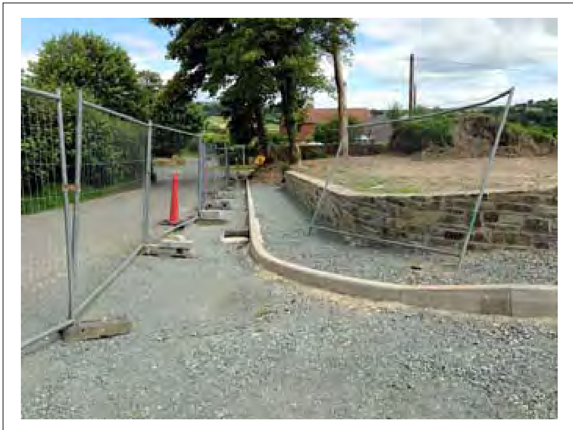
Plate 20. View of the new access, pavements and road kerb for the widened roadway to the north of the development site. Looking East.
