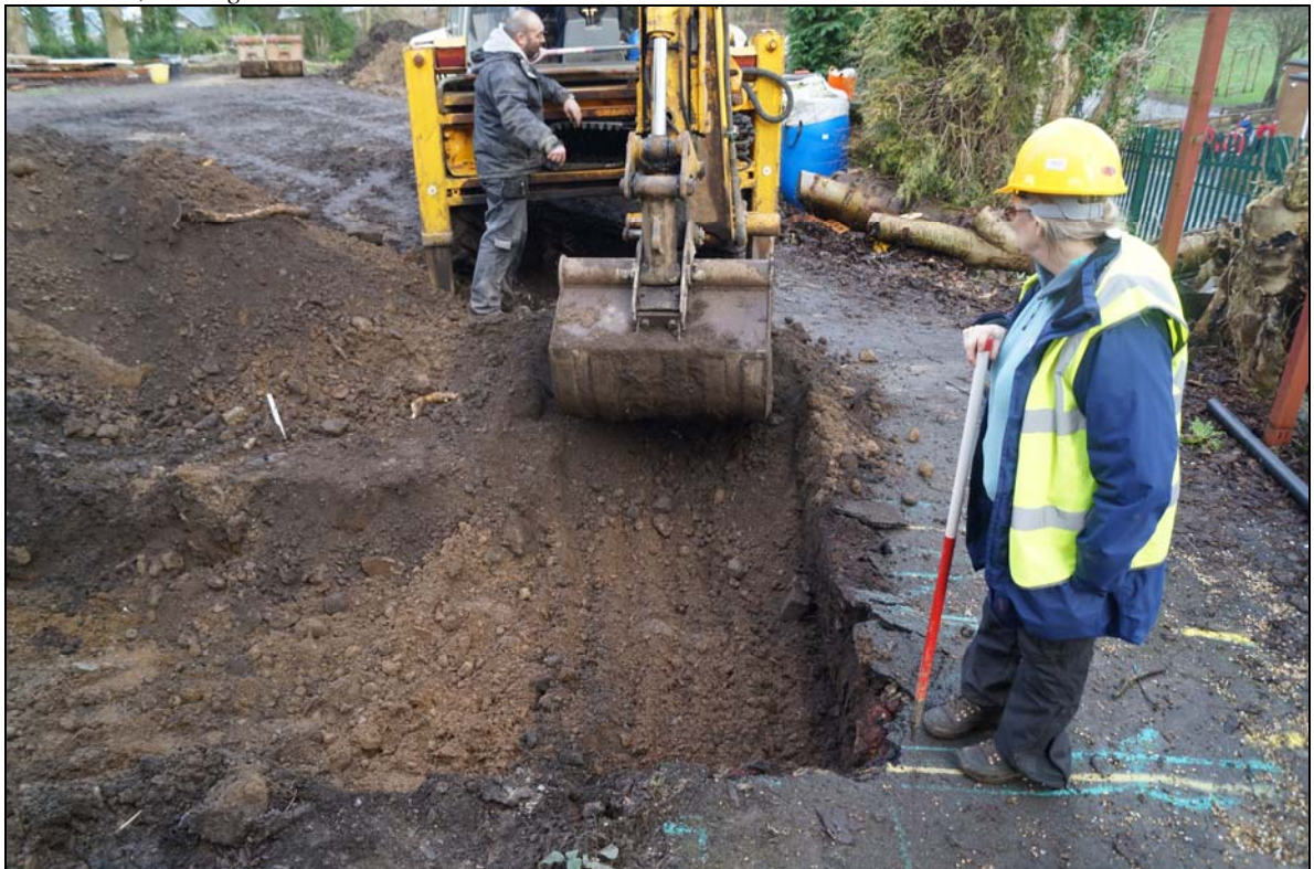
Plate 8 : PBL2016_108: Excavation of southern foundation trench, through context 001 and into natural subsoil 005, looking north northeast.
