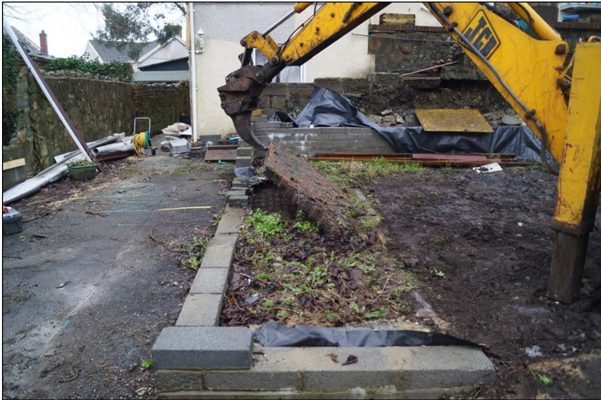
Plate 5: PBL2016_105: Removal of late 20 th century/early 21 st century footings, looking south southwest.
