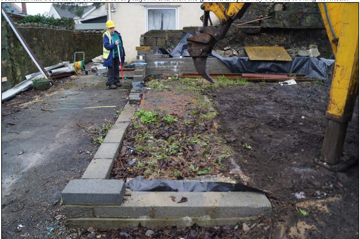
Plate 4: PBL2016_104: Removal of late 20 th century/ early 21 st century footings, looking south southwest.
