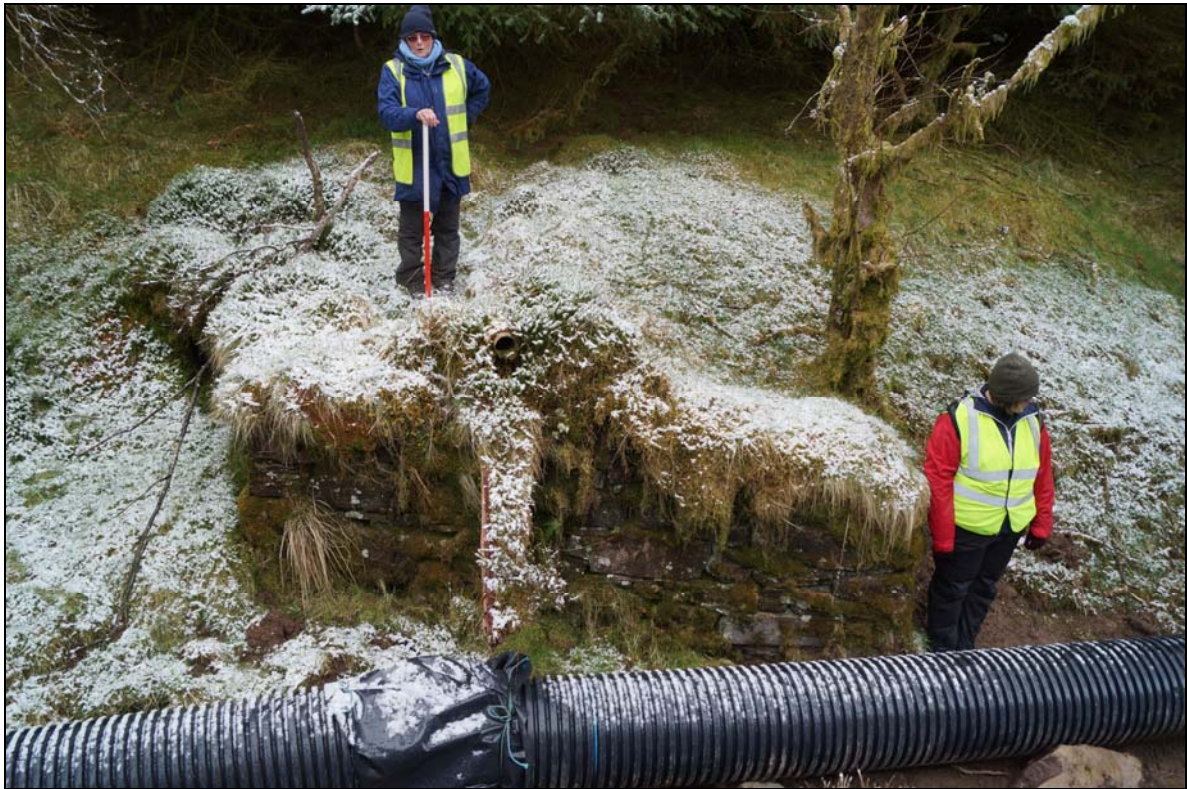
Plate 1: CNE2016_101, The remains of the stone built bridge with the central section collapsed and the abutments overgrown, looking south southwest.
