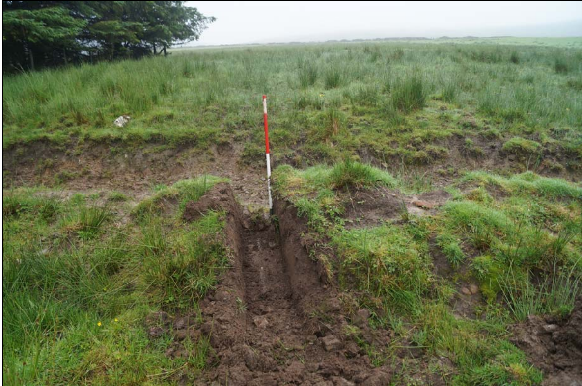
Plate 6: CNE2016_112. Looking east, at the narrow cable trench across the bank. It had been thought that the tramway embankment had been clipped redigging the ditch to the east but in fact the bank here seems to be a modern product of digging the ditch and the tramway embankment had already been lost or was never an embankment here.
