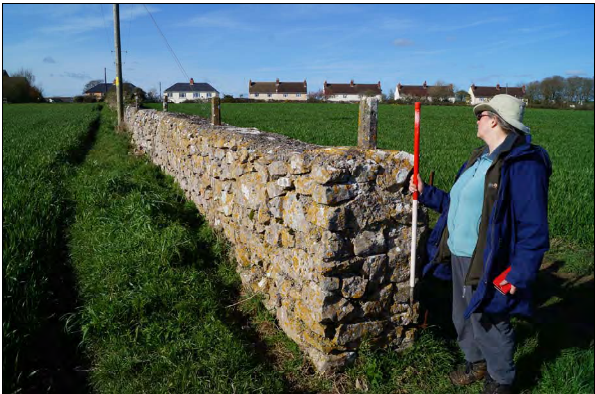
Plate 2: A view looking north at the gap in boundary wall ID Number 39, with concrete posts set within it.
