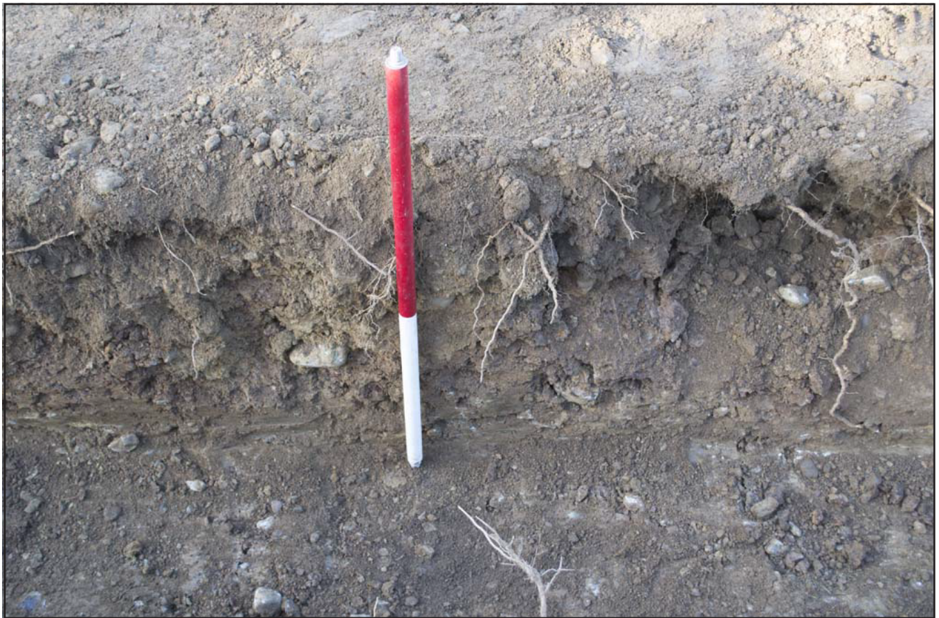
Plate 03: NE facing section of electricity cable trench; scale: 1x1m (archive reference: G22629_013).
