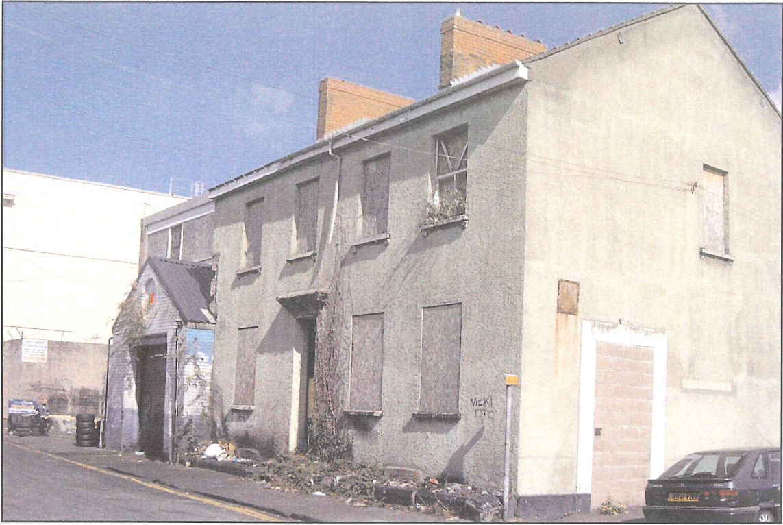
Plate 3 Mid 19th century building on the corner of John Street and East Market Street
