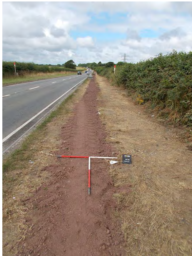
Photo 2: View west along the backfilled cable trench alongside the A40. 1m scales.
