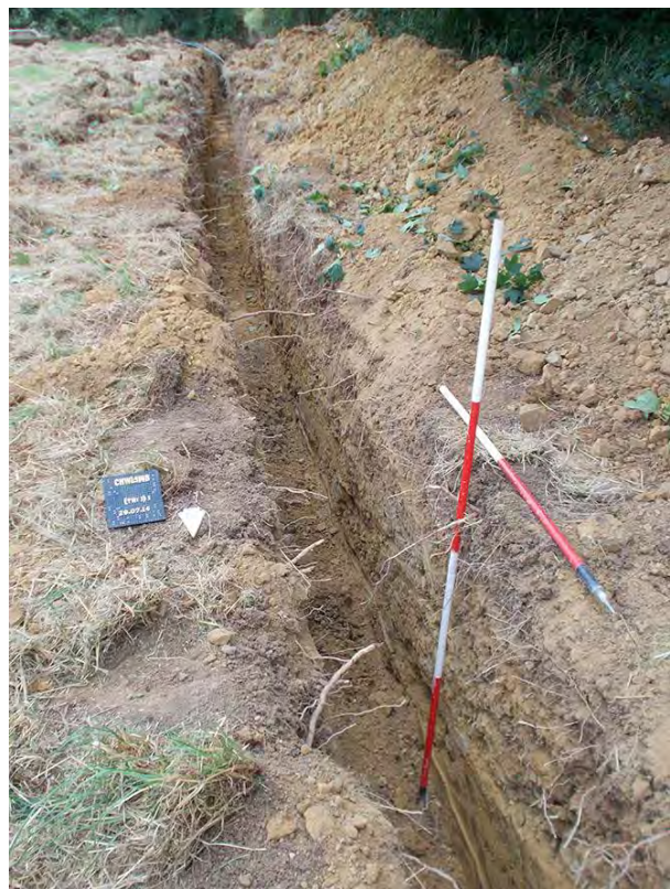
Photo 10: Looking south along a section of the cable trench just to the north of the line of the gas pipeline. 2m & 1m scale.
