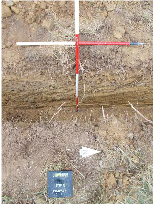
Photo 9: Looking west at a section of the cable trench just to the north of the line of the gas pipeline, showing deposits 105 and 106 (Section 4). 2m & 1m scale.
