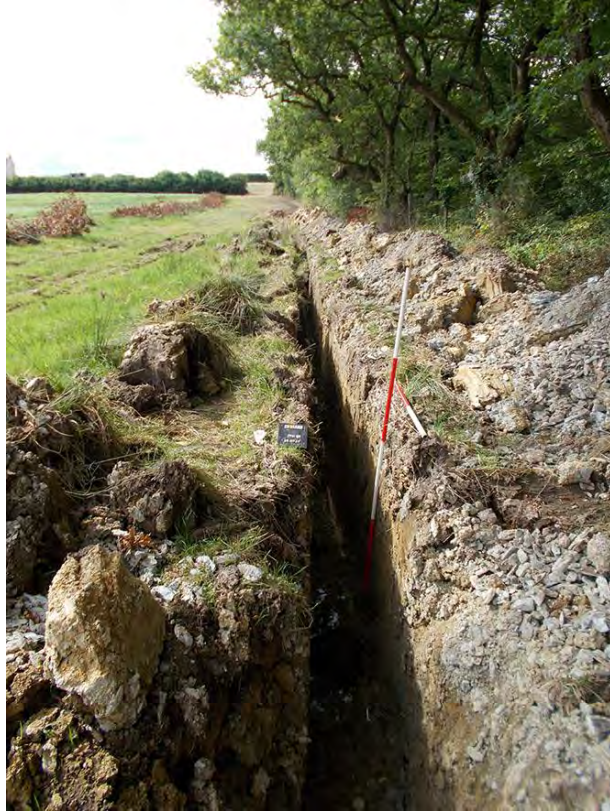
Photo 5: Looking south along a section of the cable trench as it approaches the northernmost stream, showing deposits 113 and 114. Strong sunlight prevented a meaningful photograph of the section (Section 3). 2m & 1m scale.
