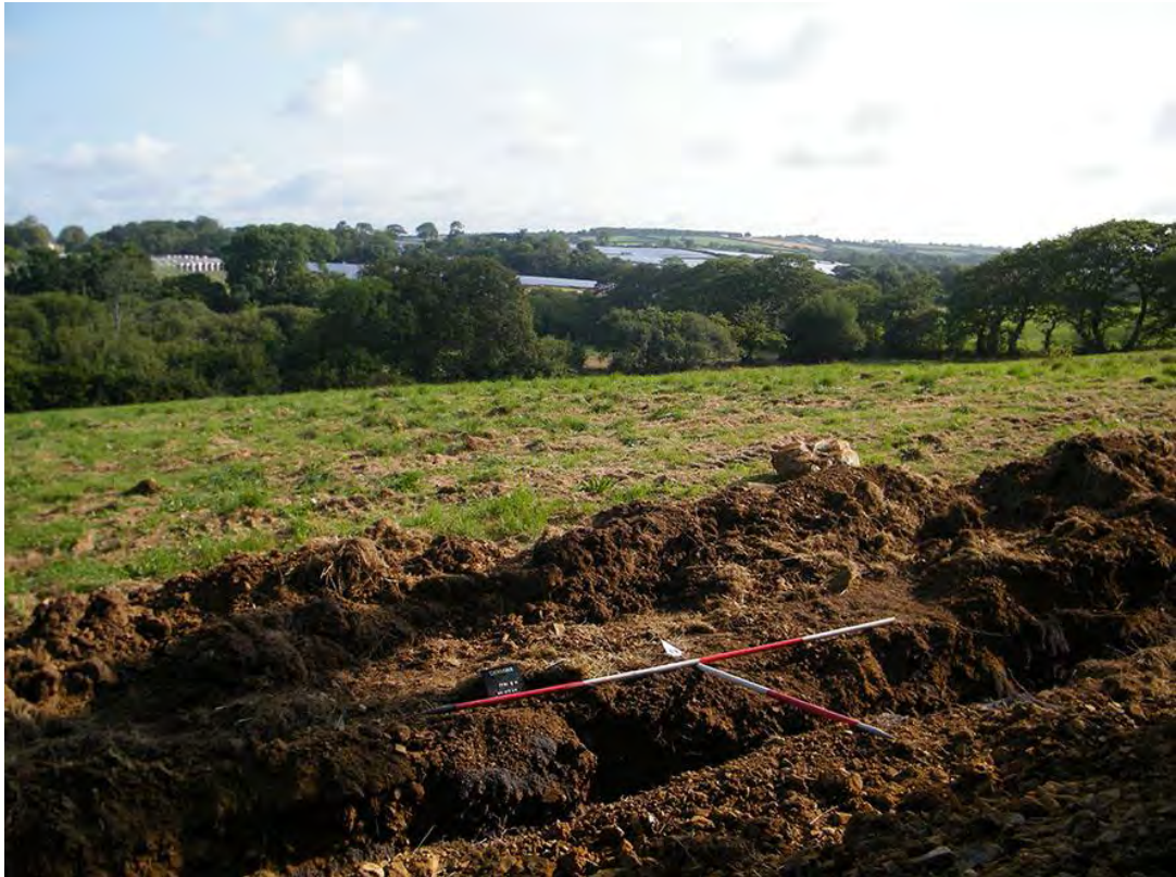
Photo 1: General view across the cable trench looking NNE with the solar farm in the background.
