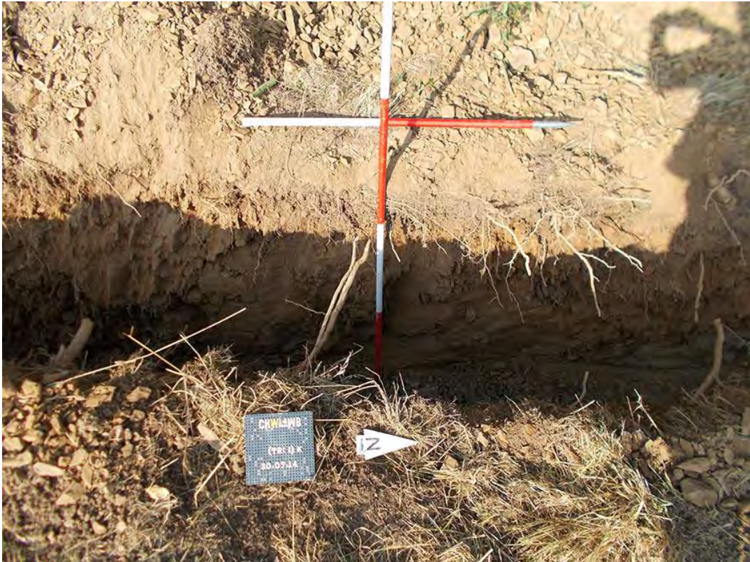
Photo 11: Looking west at a section of the cable trench between the gas pipeline and Fenton Brook, showing deposits 103 and 104 (Section 5). 2m & 1m scale.
