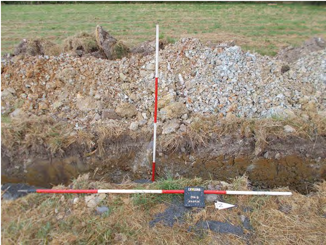
Photo 6: Looking west at a section of the cable trench between the northernmost stream and the line of the gas pipe, showing deposits 100, 101 and 102. 2m scales.
