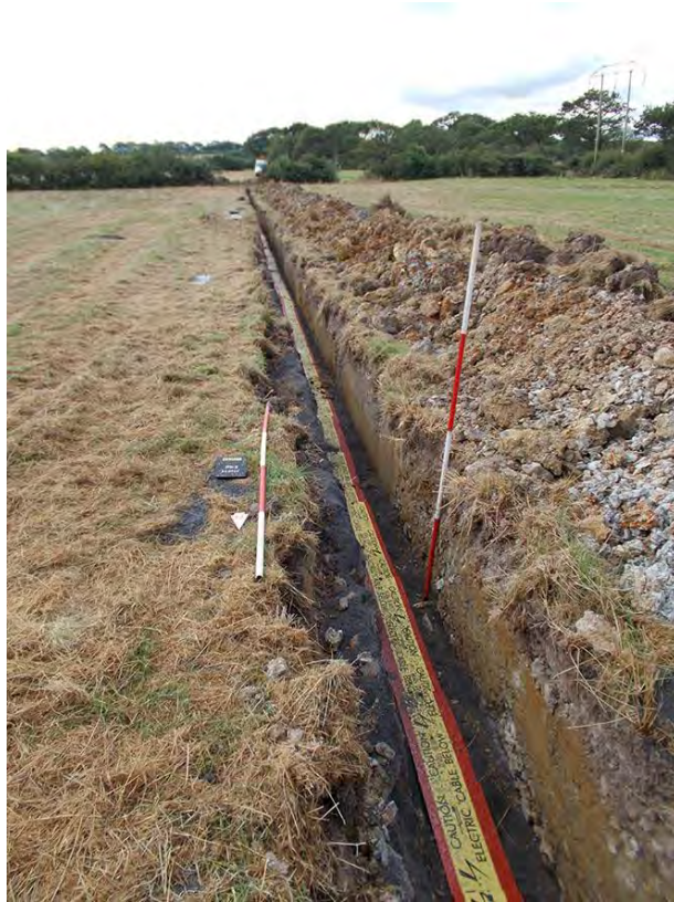
Photo 7: Looking south along a section of the cable trench between the northernmost stream and the line of the gas pipe, showing deposits 100, 101 and 102. 2m scales.
