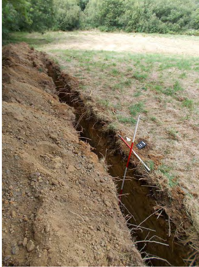
Photo 13: Looking northeast along a section of the cable trench just to the south of Fenton Brook (the wooded area to the rear), showing deposits 107 and 108. 2m & 1m scale.
