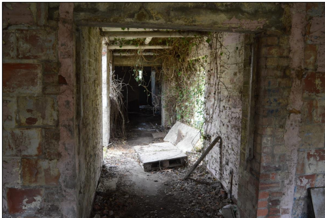
Fig. 10 The covered access way between Buildings 1 and 2, from the south. Photo CPAT 4486-0097
