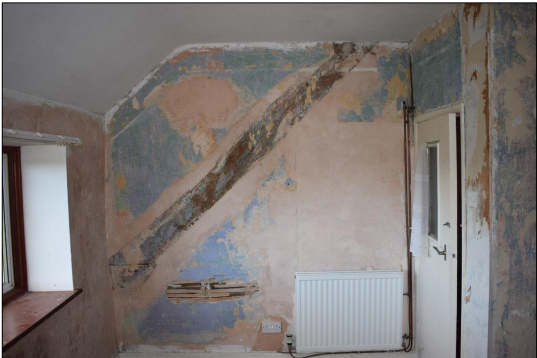
Fig. 10: The north-west end of the roof truss visible on the first floor in room F1, with slots for the purlins of the original roof. The projecting horizontal stub of the sawn-off horizontal beam can be seen to lower left. CPAT 4599-0020
