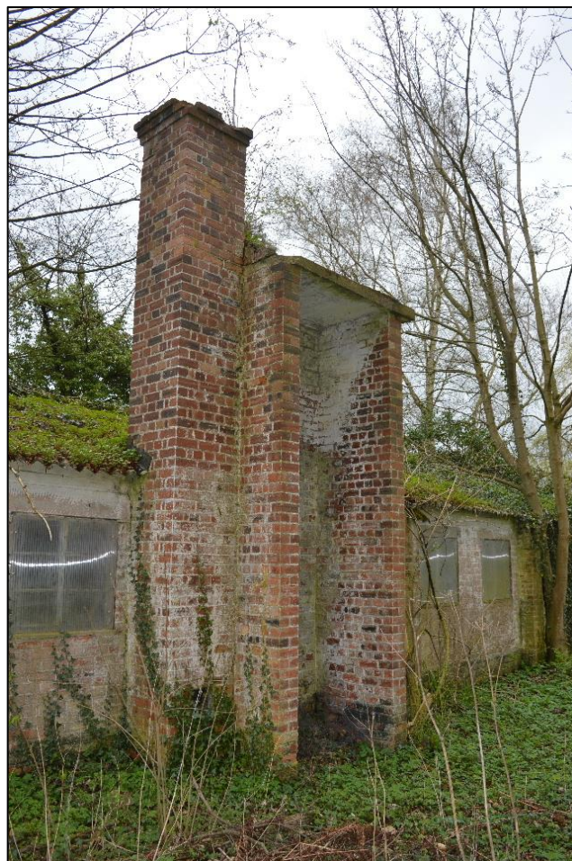
Fig. 12 The chimney stack and water tank support, viewed from the south. Photo CPAT 4486-0066
