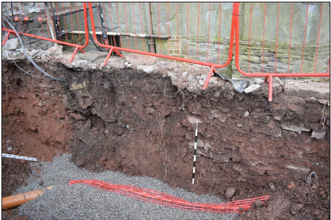
Fig. 9 View from the west of the foundations for the boundary wall between the museum and the council offices. Photo CPAT 4323-0026
