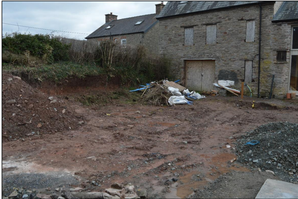
Fig. 3 View from the north-west across the site towards the farmhouse Photo. CPAT 4605-0008
