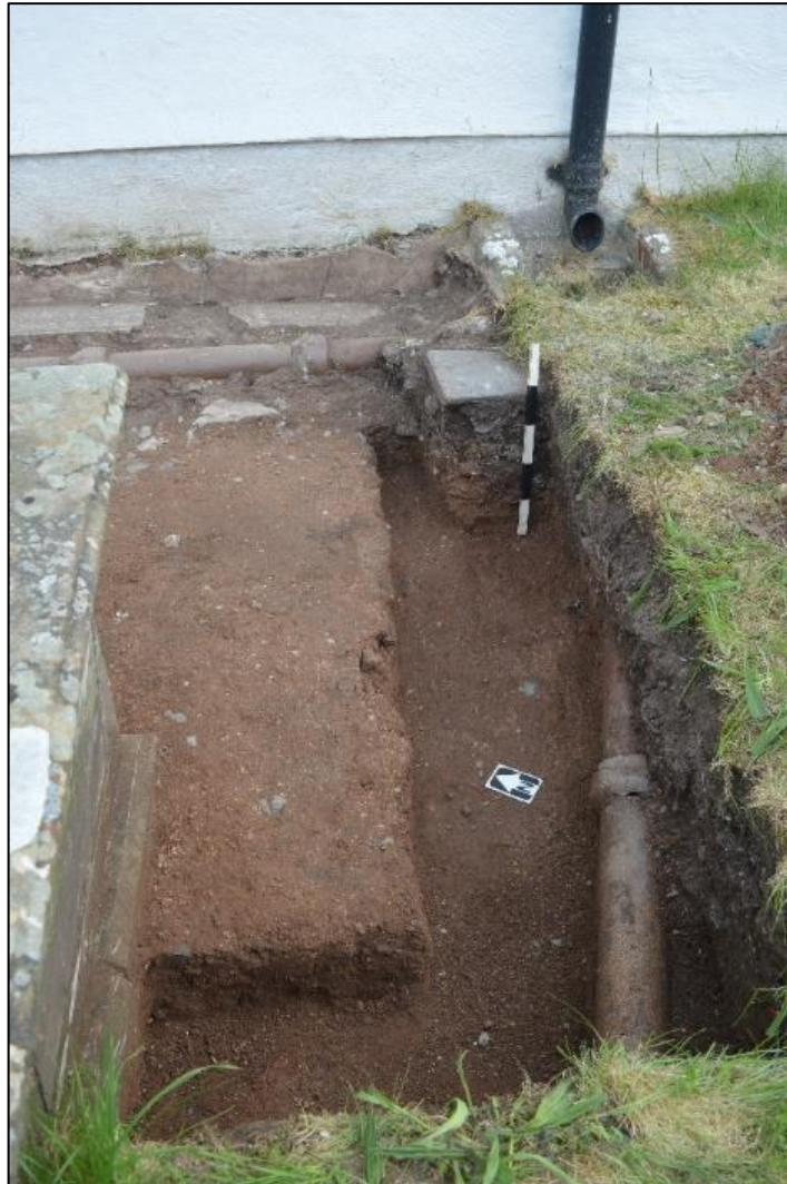
Fig. 11. View of the west wall showing the location of the south-east footings and drainage (03). Viewed from the west. Photo CPAT 4507-0013
