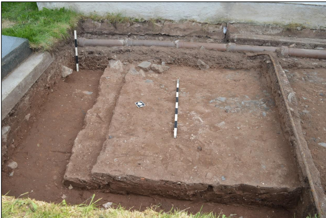
Fig. 7. Excavated ring beam footings, deposit 04 in-situ . Electrical cable (13) to the right. Viewed from the west. Photo CPAT 4507-0003
