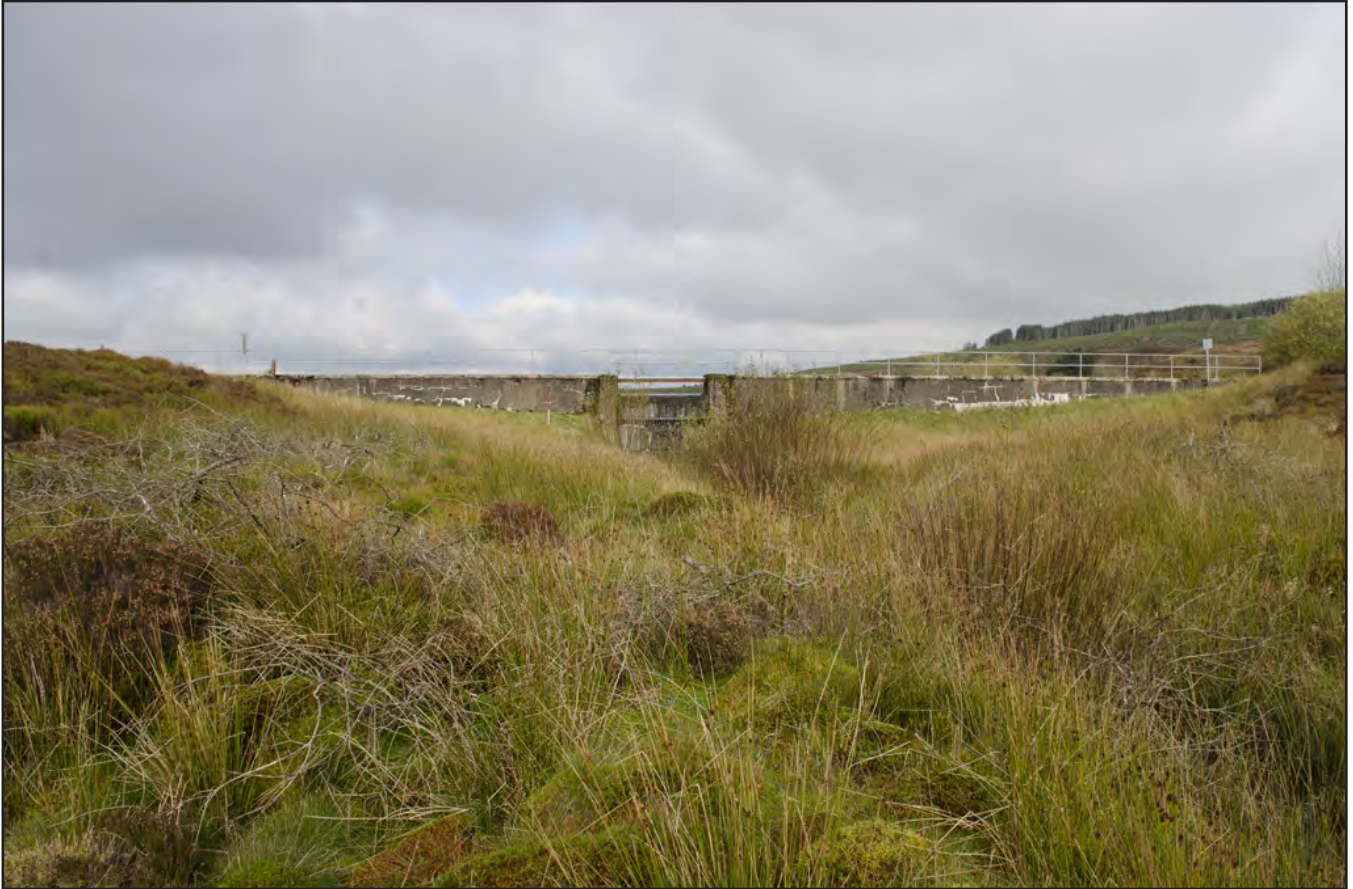
Plate 1: General view of dam with central weir; scale: 1x1m (archive reference: G2580_001).
