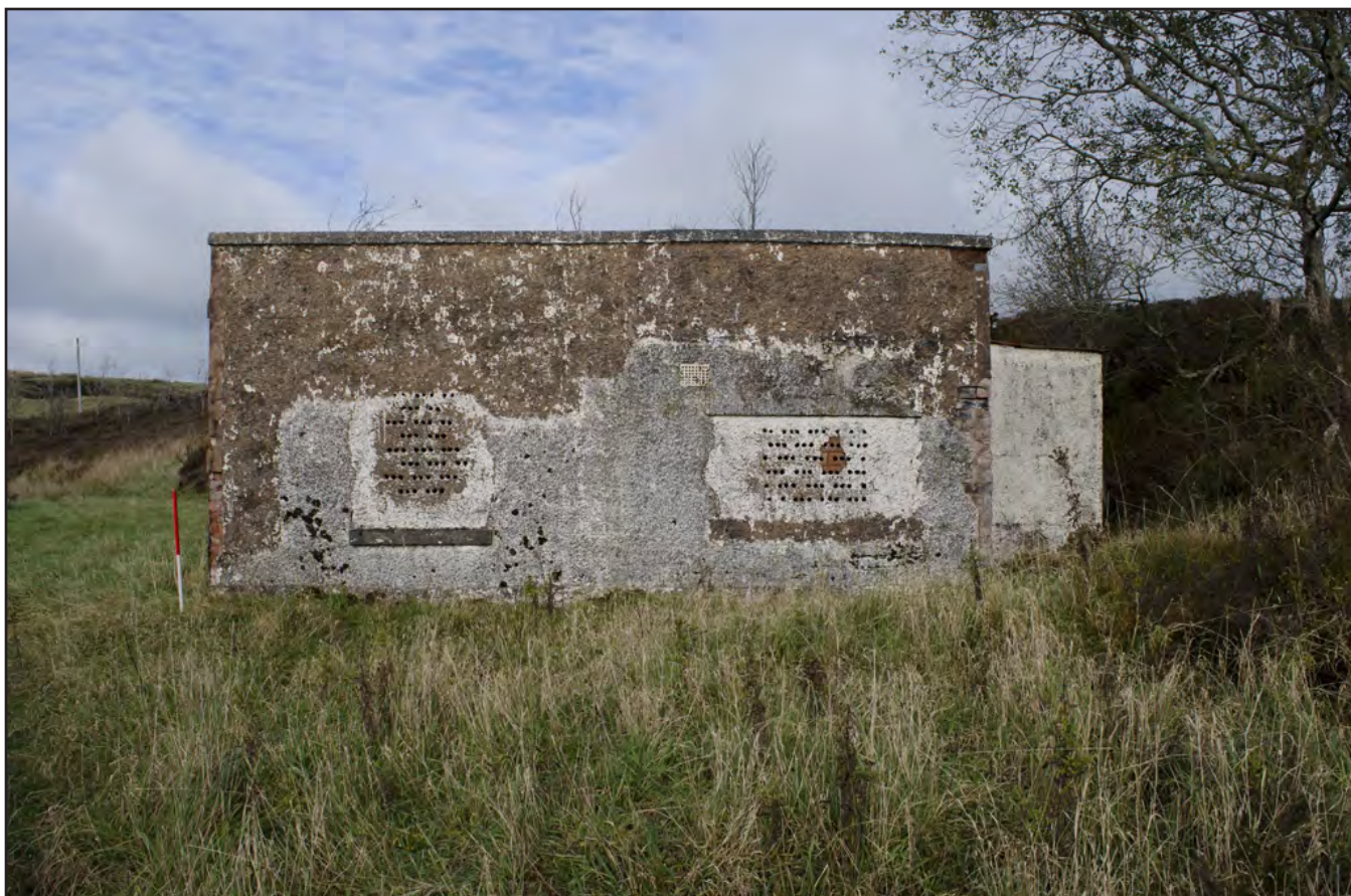
Plate 14: View of blocked up windows on the brick and concrete building; scale: 1x1m (archive reference: G2580_018).
