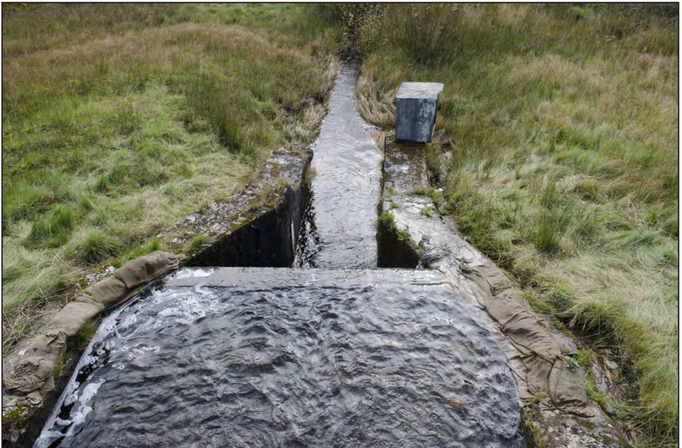
Plate 4: Weir structure from the dam wall; scale: not used (archive reference: G2580_004).
