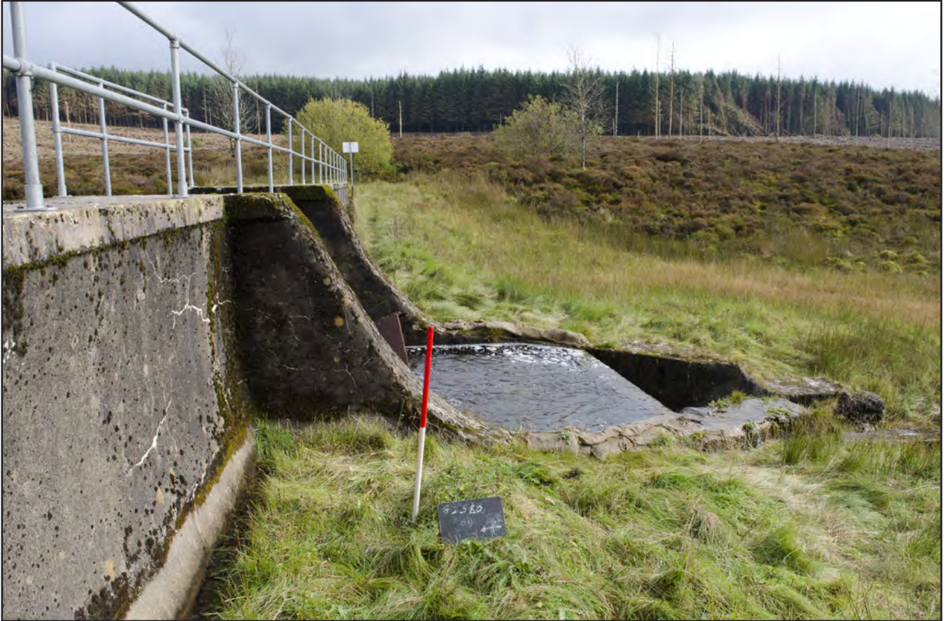
Plate 3: View of concrete walls of weir and dam; scale: 1x1m (archive reference: G2580_003).
