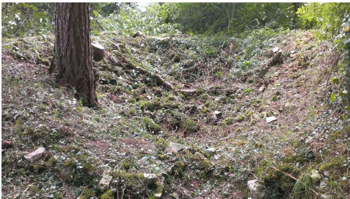
Fig. 7. View of the structure looking west before excavation, showing the extent of collapse.
