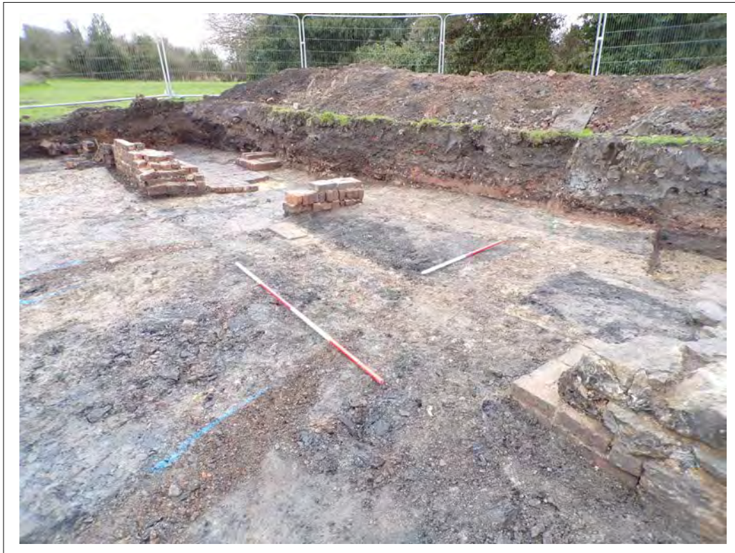
Plate 31. View of clearly defined robbed wall lines. Looking south. Scales 1m & 2m
