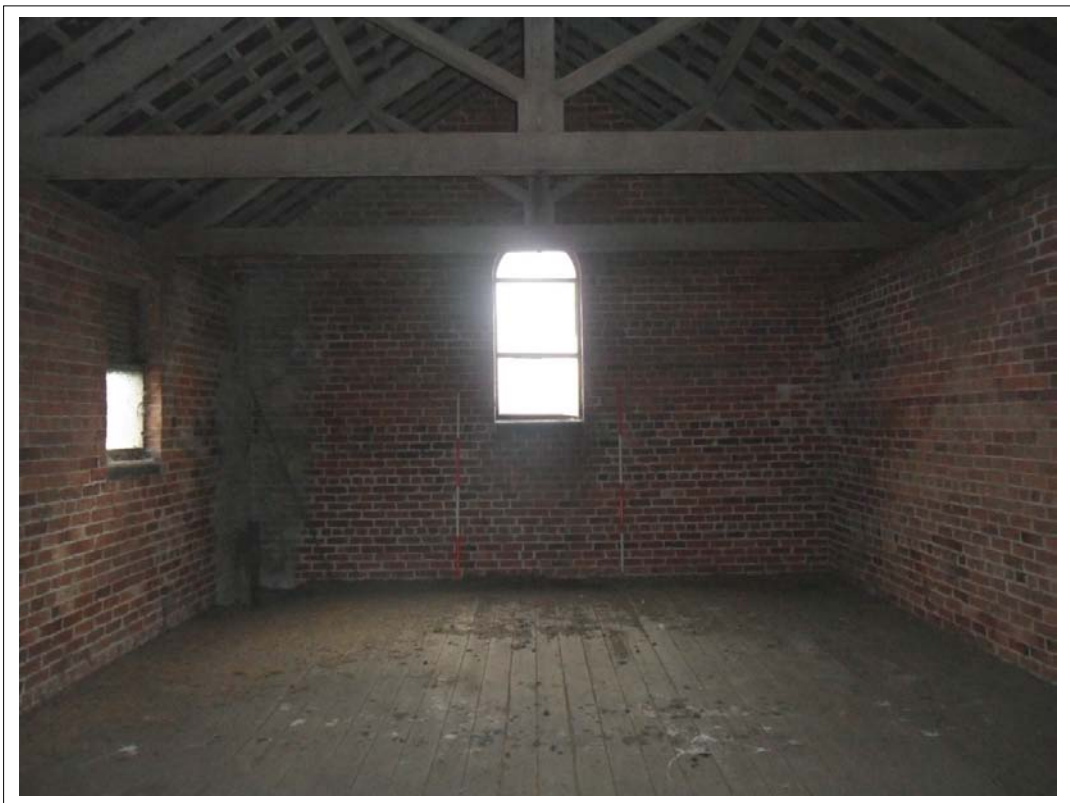
Plate 150: View south east of end of open space on upper floor Note ladder access bottom left, Scales 2x2m
