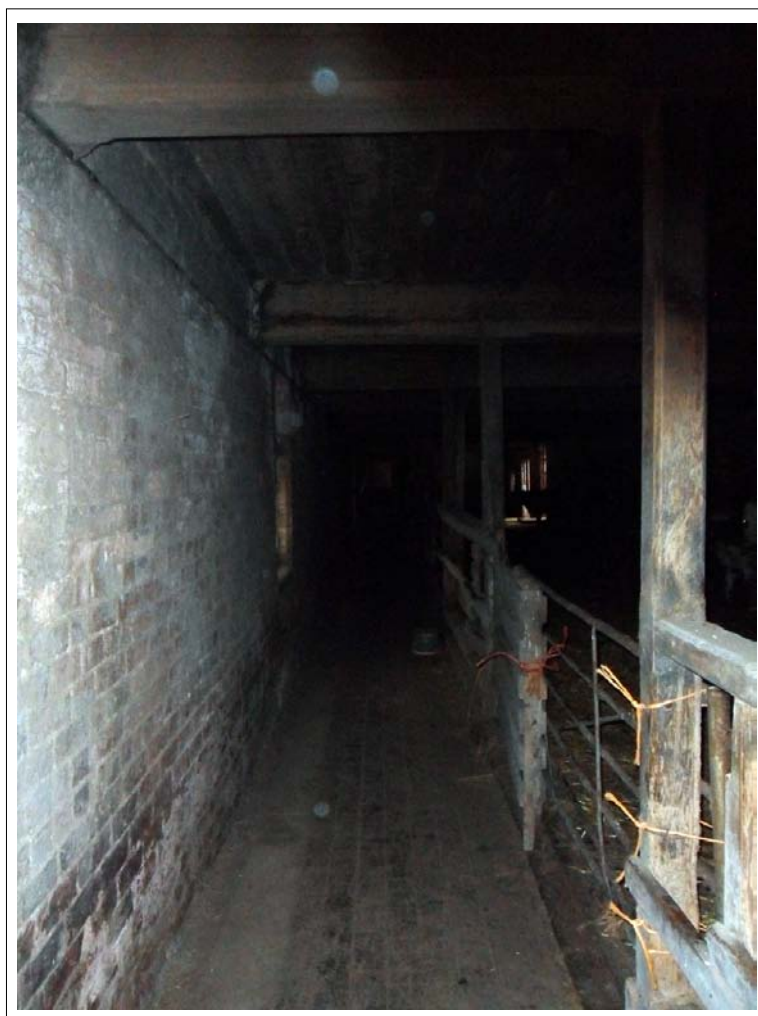
Plate 100: View down corridor running north west to south east along animal pens.
