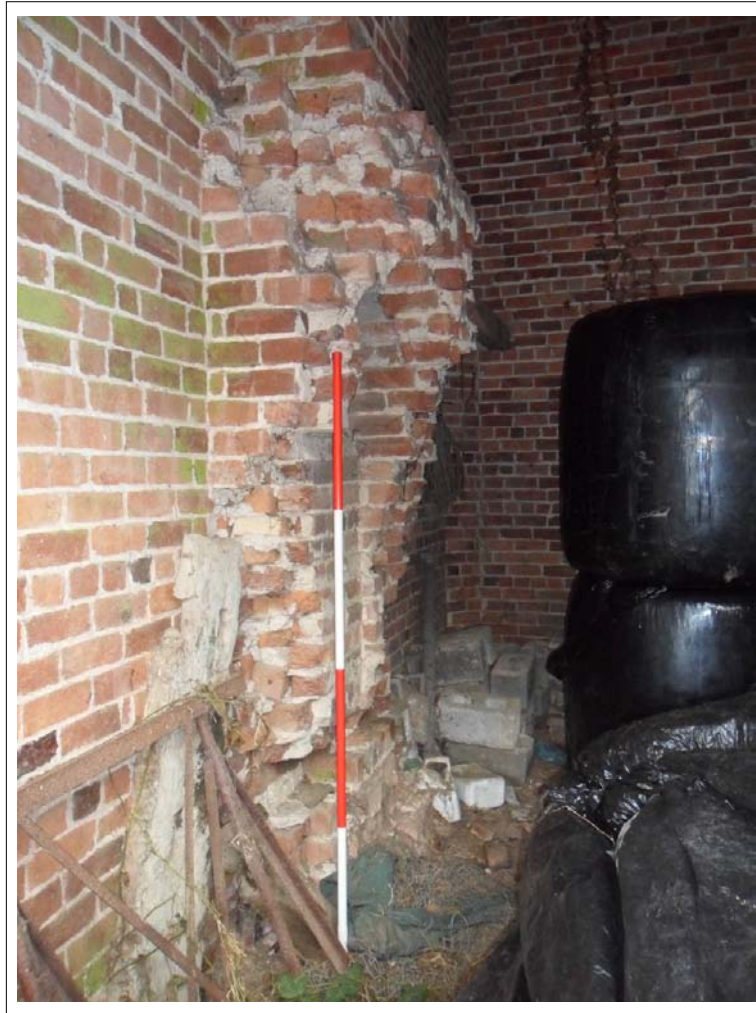
Plate 75: View of damaged/removed fireplace within groundfloor room, north western edge of complex Scale 1x2m
