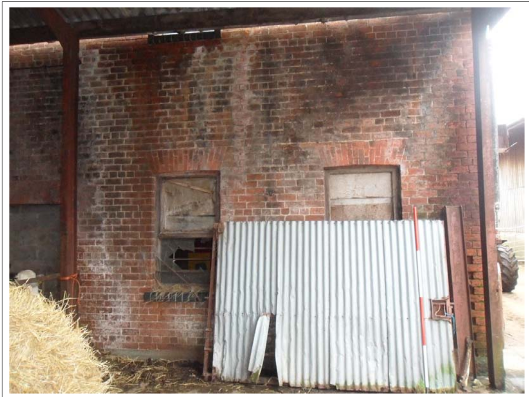
Plate 31: View of windows in north west wall of animal range 3 Scale 1x2m, Looking south east
