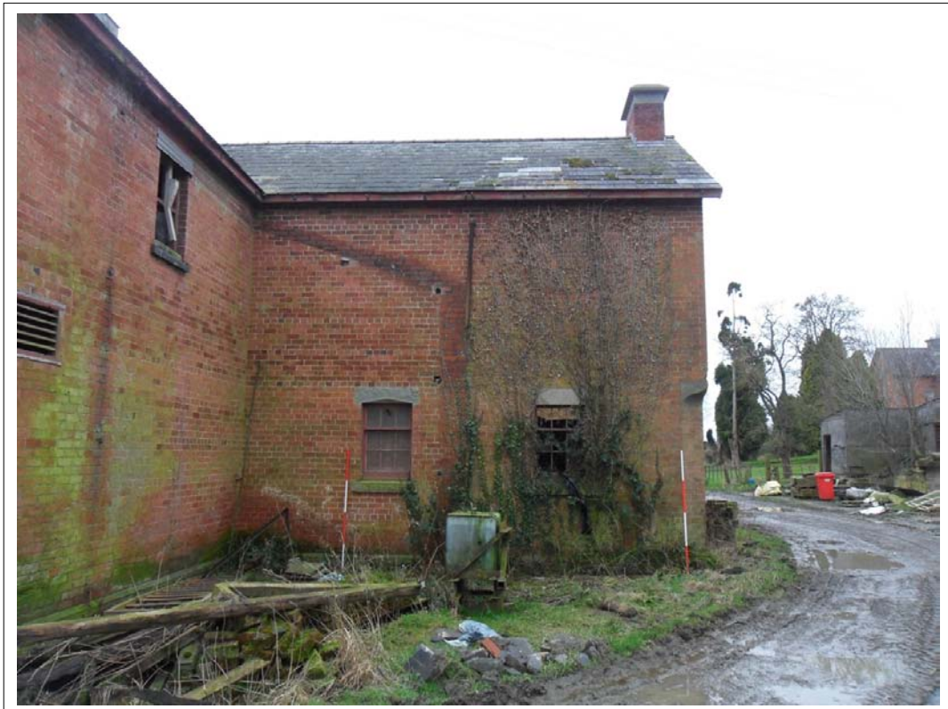
Plate 40: View of north east wall of gable end adjacent to stable block Note lines on brickwork possibly indicatin the presence of a now removed structure/lean to. Scales 2x2m, Looking south west
