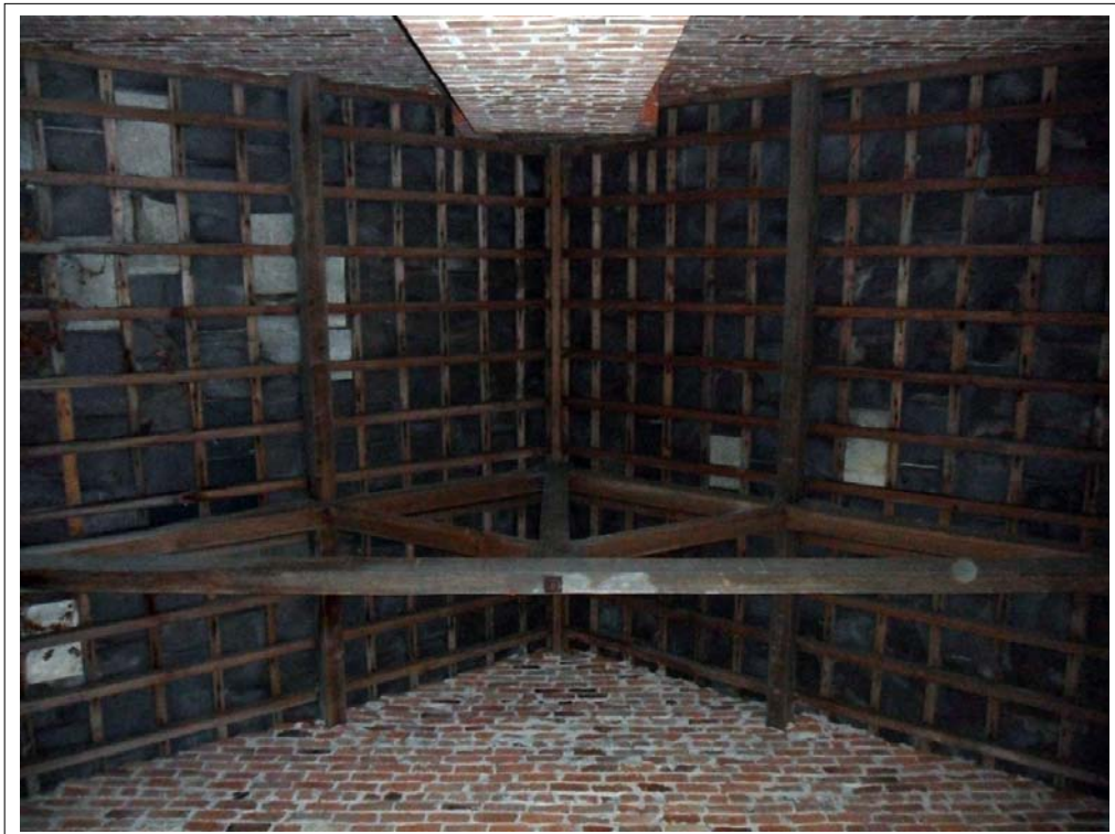
Plate 76: Detail of roof and rafter construction in room with damaged/removed fireplace. Note no upper level.
