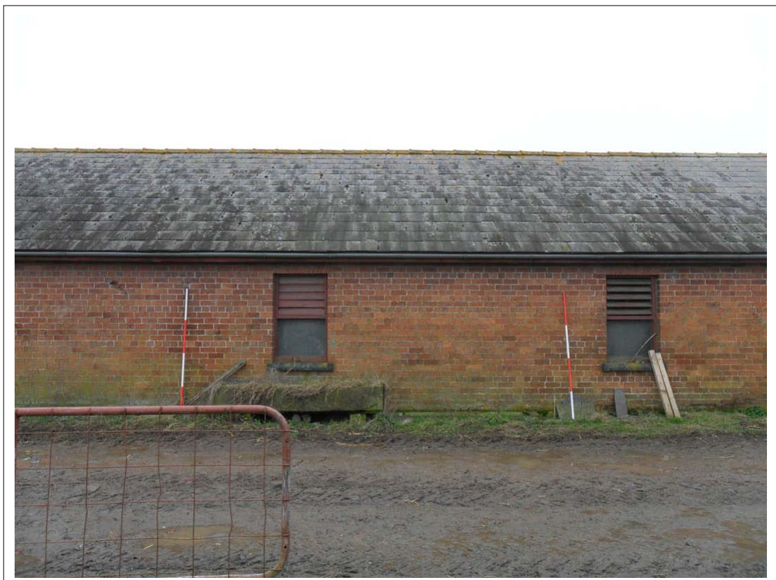
Plate 14: View of rear wall of animal range, Scales 2x2m, Looking south east
