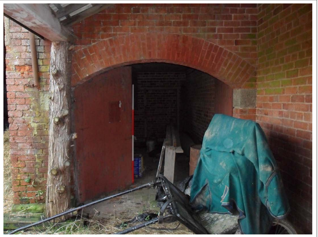
Plate 4: View of arched doorway within 'porch' area, Scale 1x2m, Looking north west
