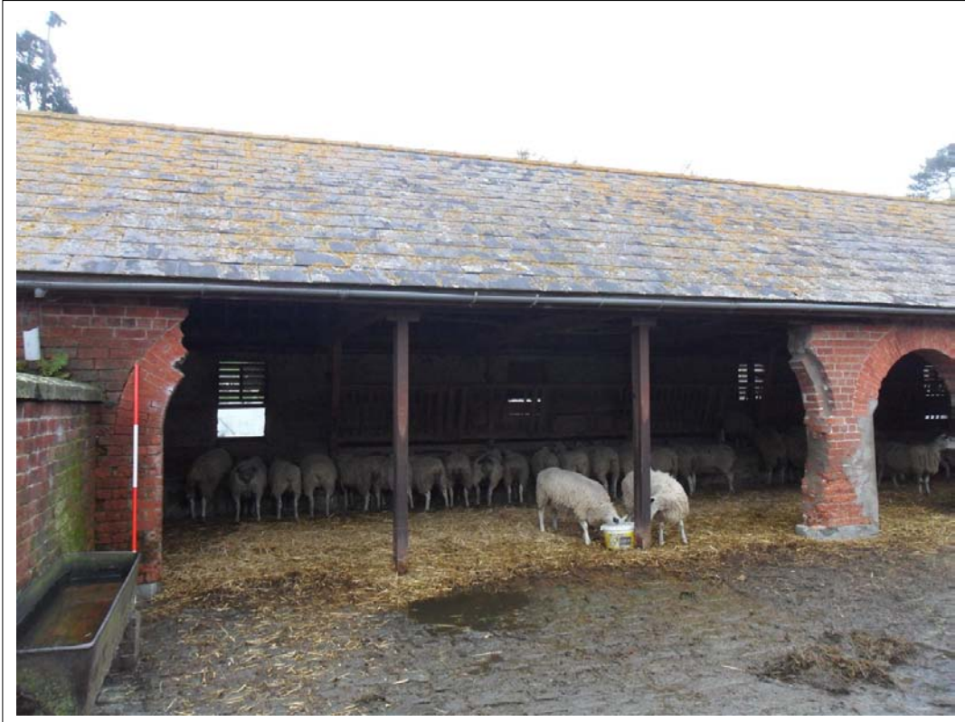
Plate 21: View of damaged/removed arched entrances into single storey animal range. Brickwork replaced with steel bars. Scales 1x2m Looking north
