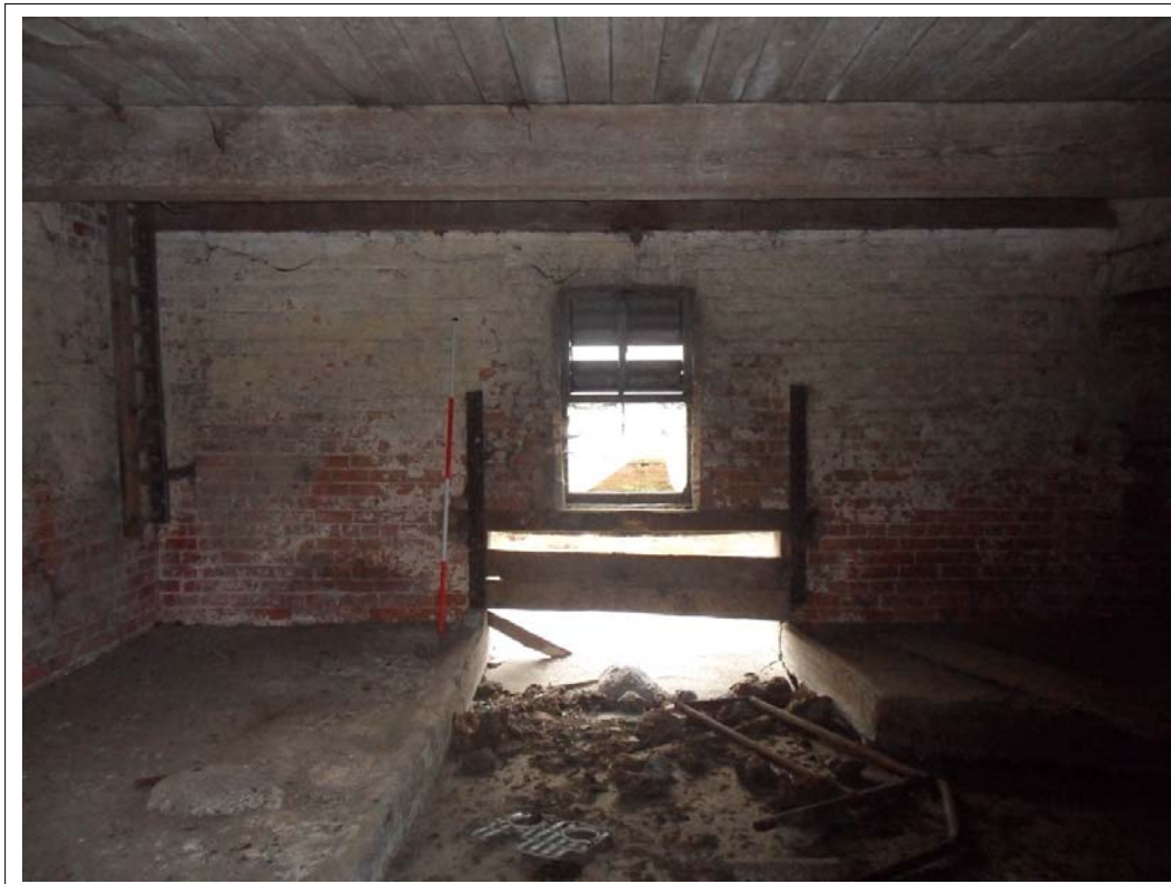
Plate 128: View of effluence recess exit through south eastern end wall of corridor Scale 1x2m
