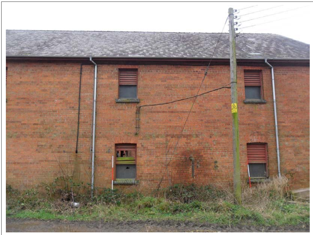
Plate 45: View of rear wall of cart store and upper storey grain store Scales 2x2m, Looking south west
