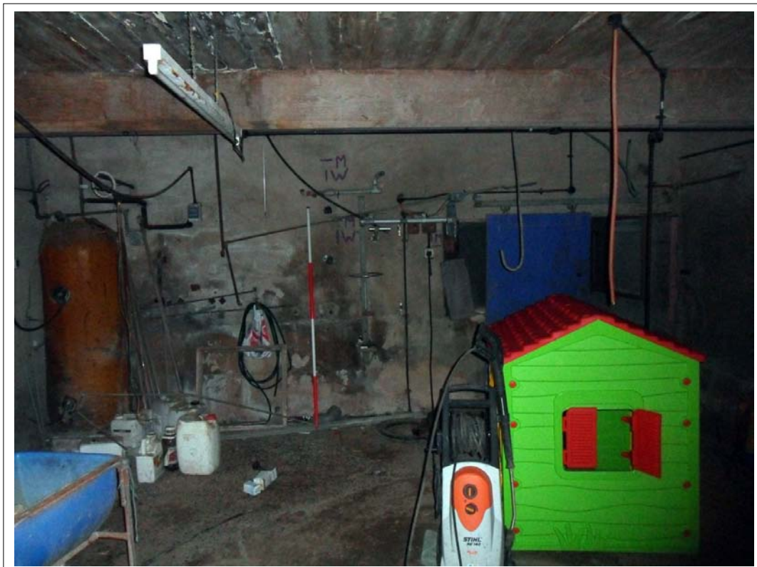
Plate 158: View of back (north east) wall of boiler room at end of animal range 3 ground floor, Scales 1x2m
