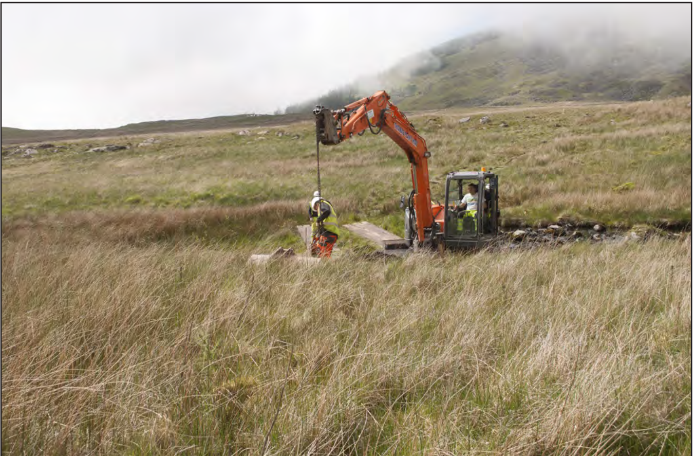
Plate 04: Working shot showing machine bringing equipment forward. View from the south east (archive reference number: G2522_50).
