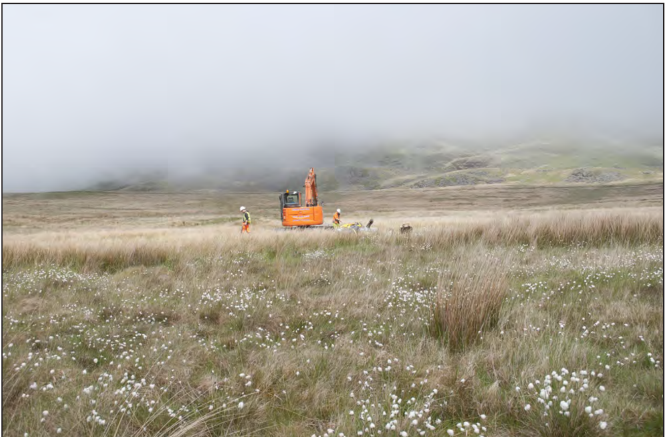
Plate 02: View from the south east along the access route prior to machine tracking over (archive reference number: G2522_38).
