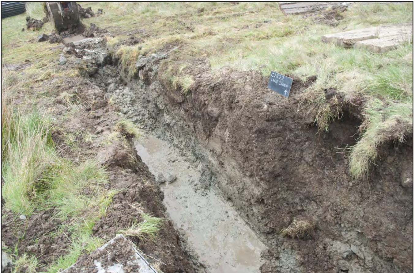
Plate 06: Working shot of excavation of land drain. View from the south east (archive reference number: G2522_54).
