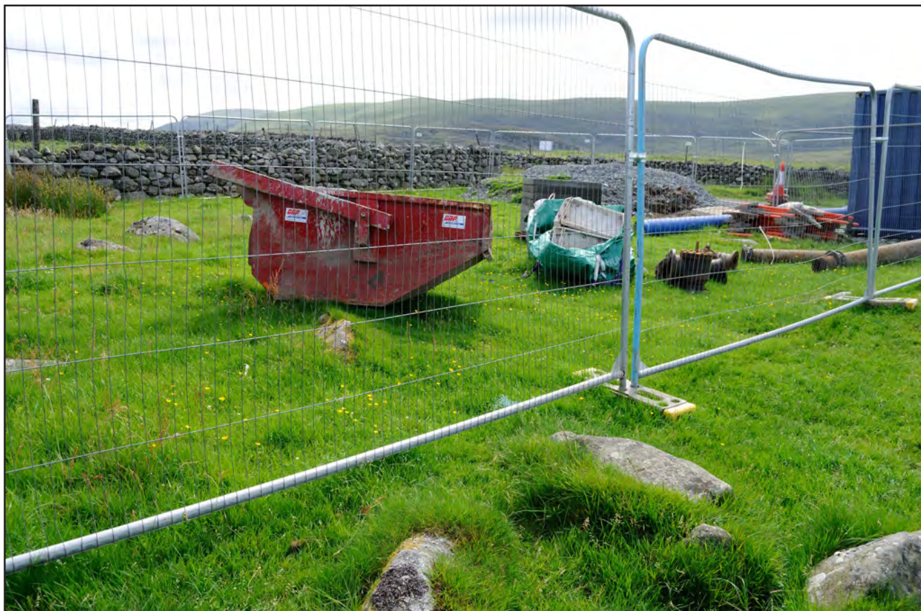
Plate 07: Compound area for stores viewed from the south west (archive reference number: G2522_63).
