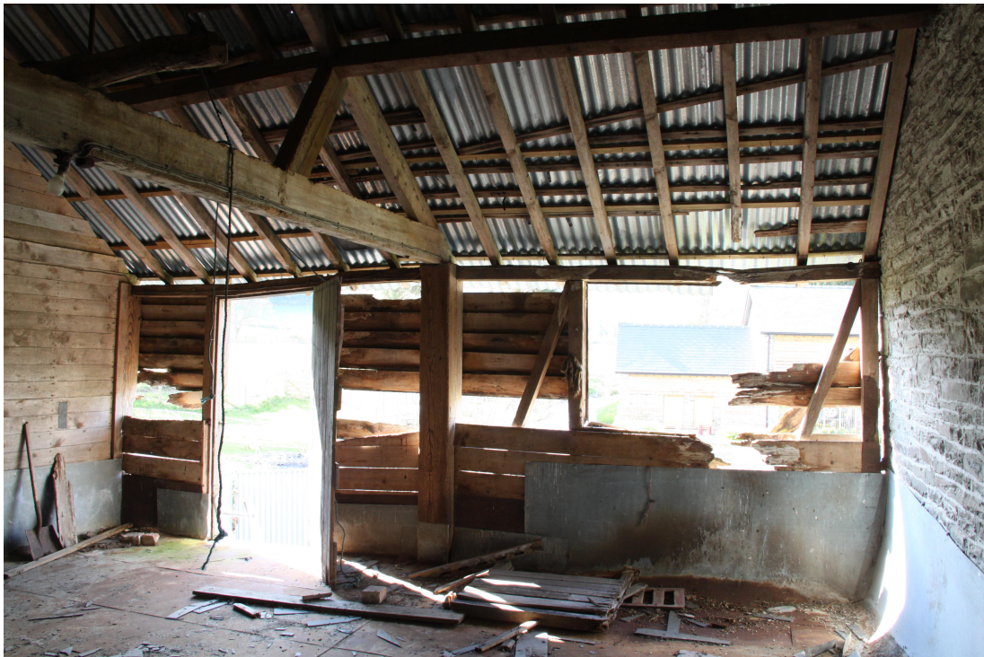
Plate 60 - AD011_060: Timber frame and weather boarding to north-east of granary/hay loft.
