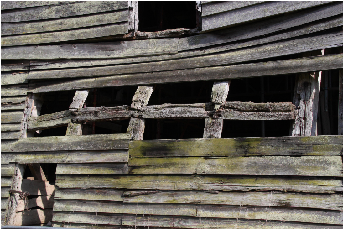
Plate 53 - AD011_053: Exposed framing on north-west lateral wall, showing weather damage.
