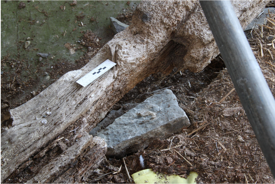
Plate 37 - AD011_037: Deteriorated mortice in sill beam.
