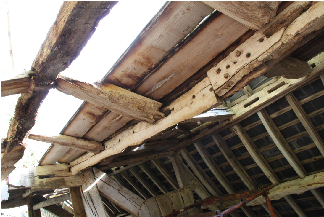
Plate 46 - AD011_046: Stave holes in rail, indicative of wattle and daub infill.
