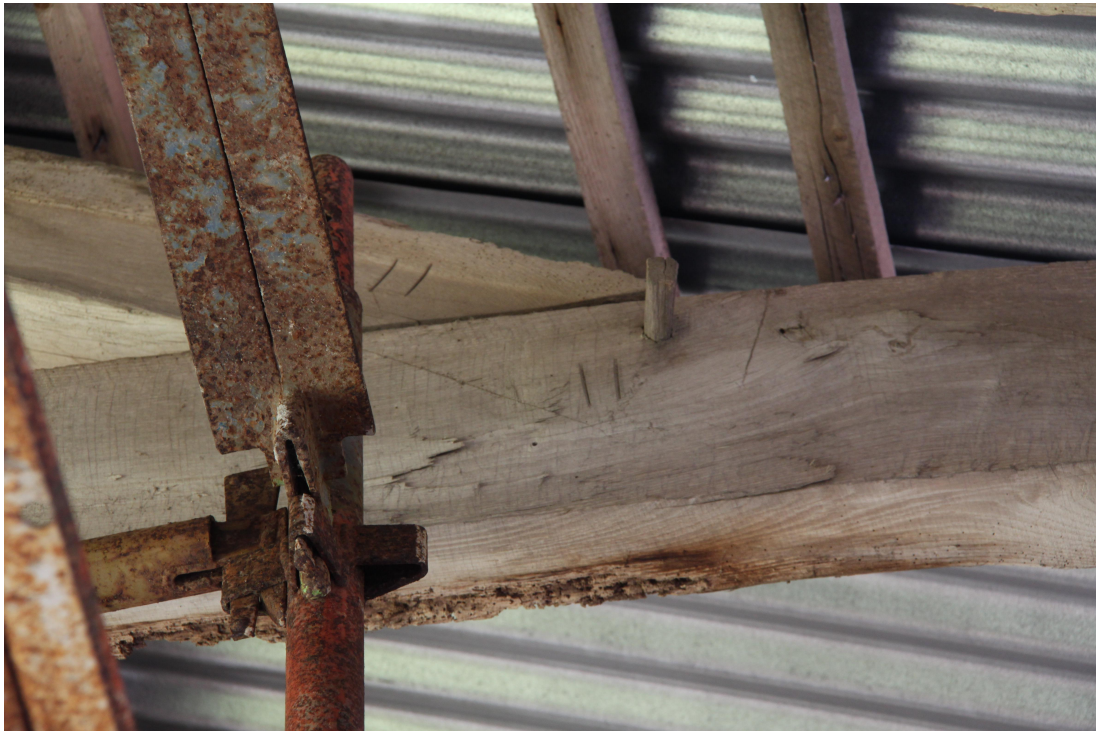
Plate 49 - AD011_049: Detail of raised roof; later principle rafter showing carpenters assembly marks.
