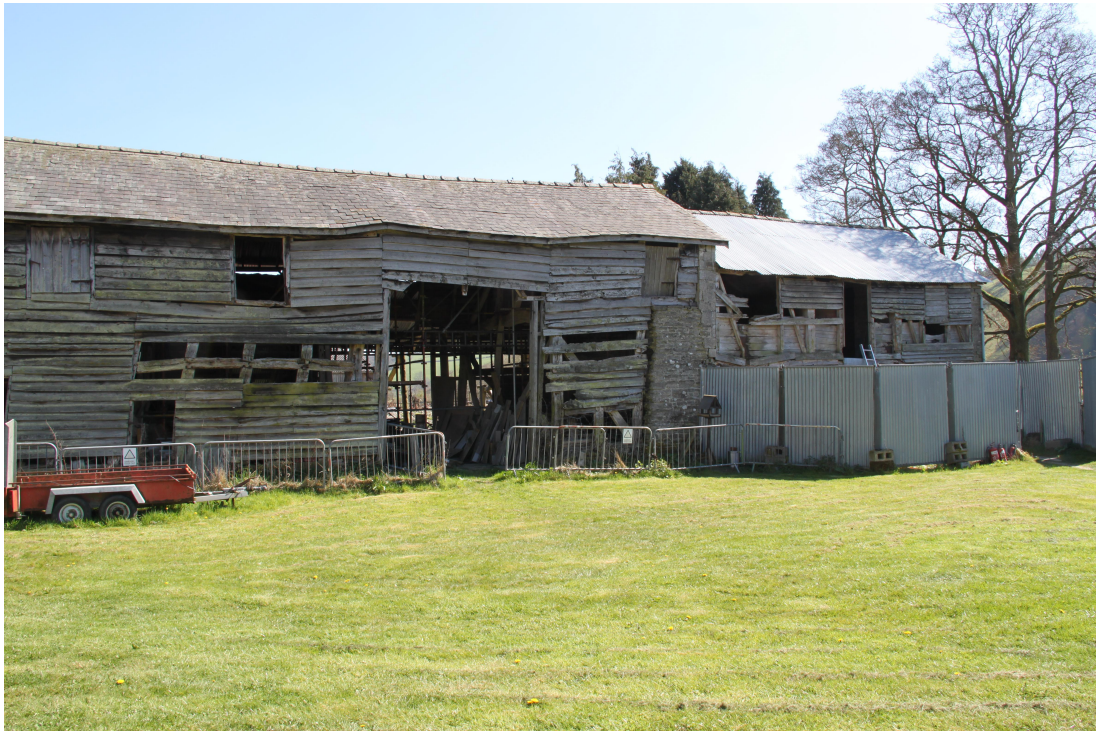
Plate 3 - AD011_003: General view of north-west elevation; Barn, and Cart Shed and Granary.
