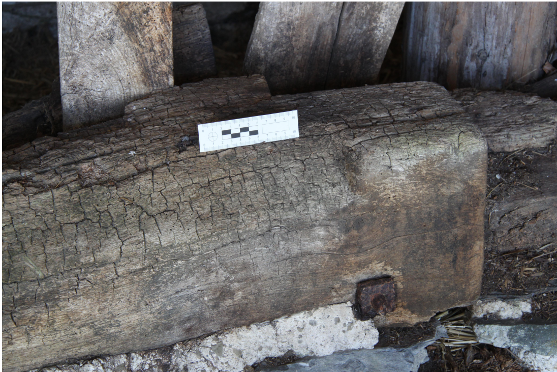
Plate 31 - AD011_031: Reused floor beam, circa late C16th. Showing stop and deep chamfer.
