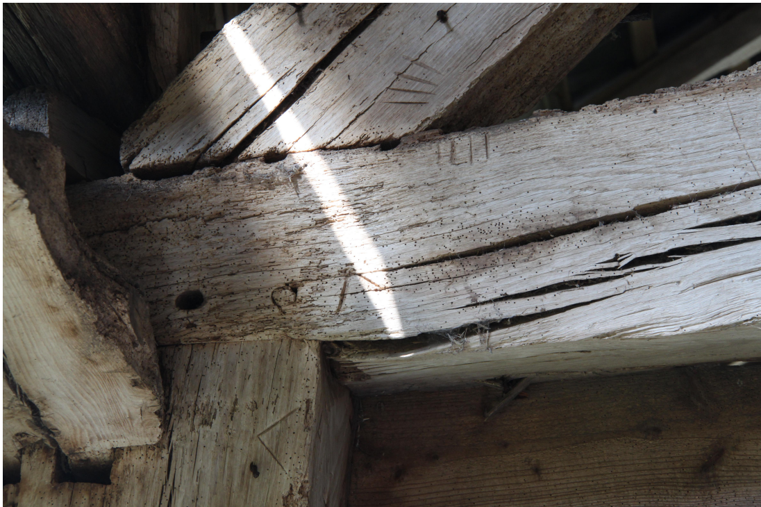
Plate 42 - AD011_042: Carpenters marks on tie beam, post and principle rafter of truss 2.
