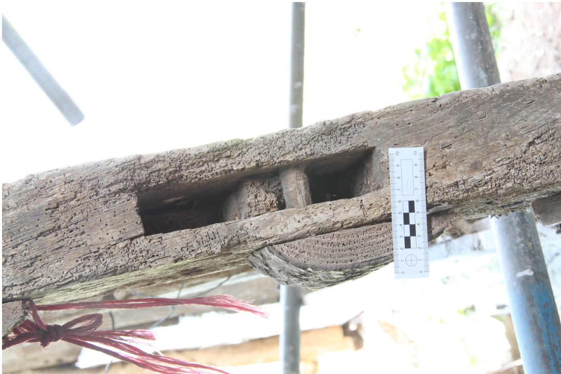
Plate 36 - AD011_036: Empty mortise in post of truss 1.
