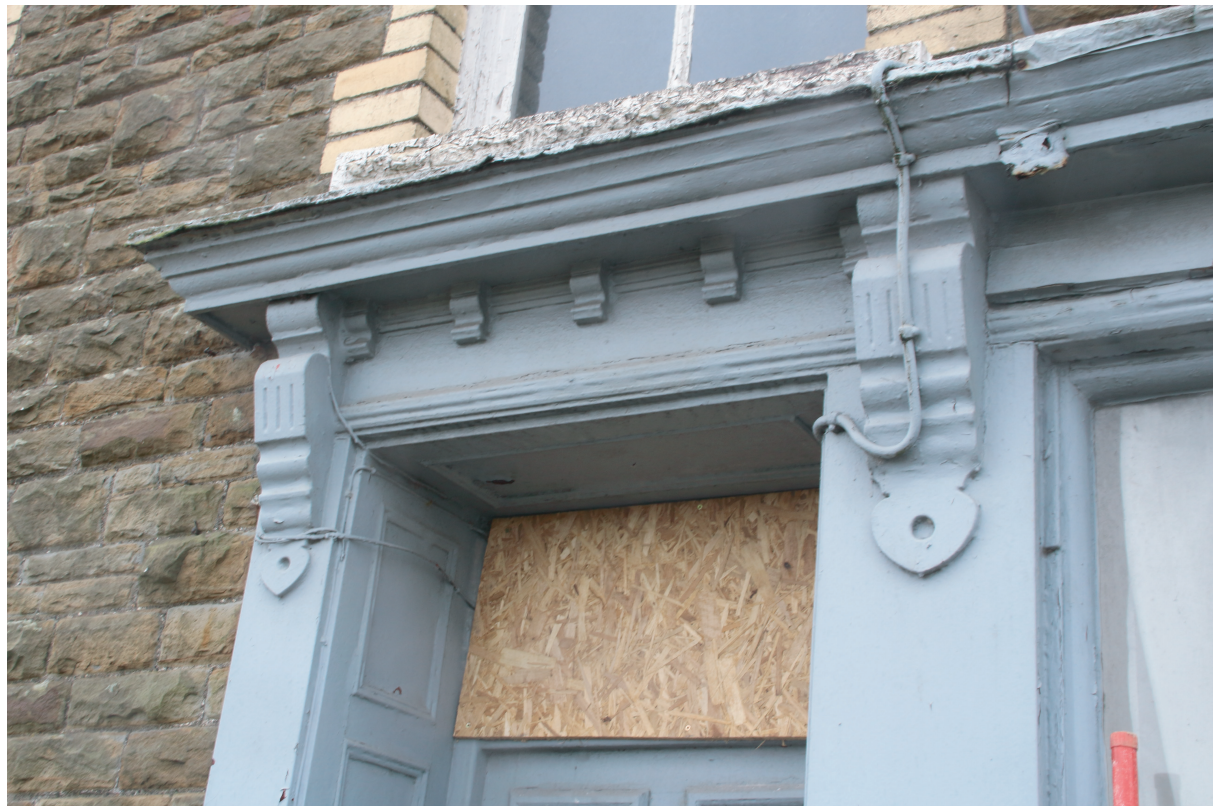
Plate 19. London House, Beach Road, Penclawdd. Detail of moulding above house doorway. Looking southwards.
