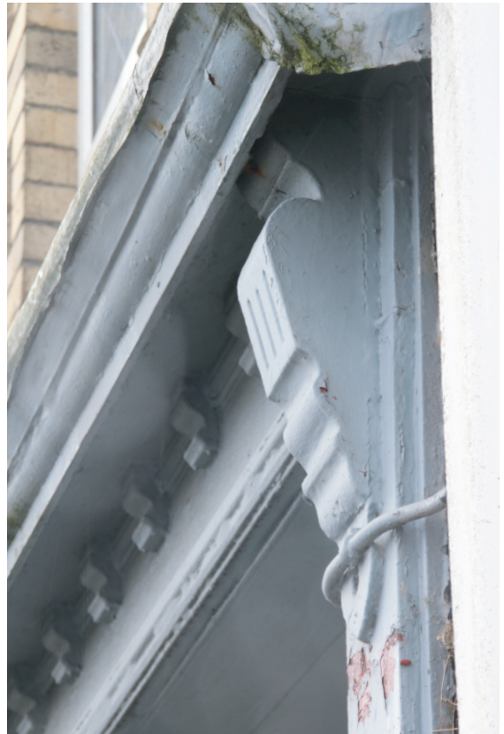
Plate 18. London House, Beach Road, Penclawdd. Detail of moulded corbel on shopfront. Looking southeast.
