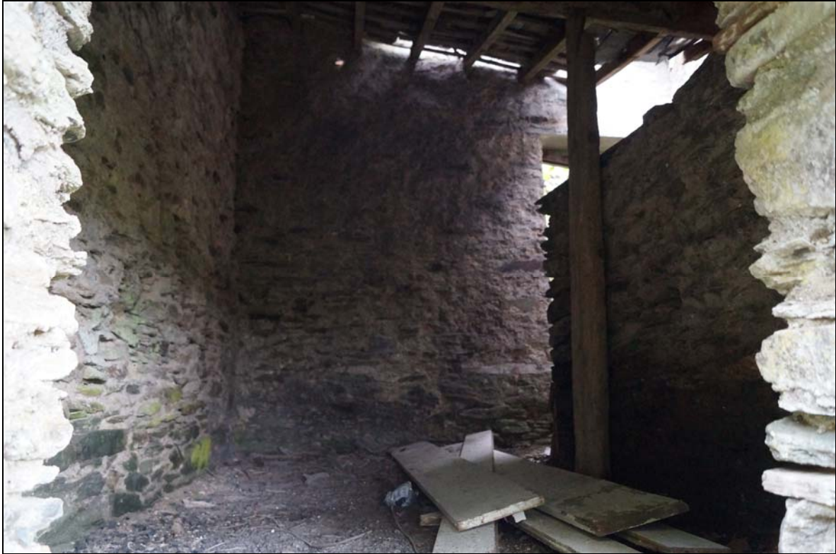
Plate 5: TYC2016_105 – the interior of the small outbuilding added to the former school at Cyfyng, ID numbers 7 & 8, looking west.
