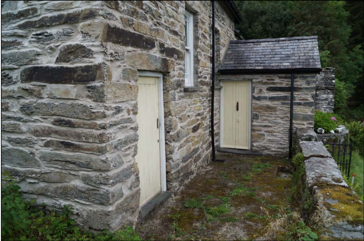
Plate 3: TYC2016_103 - the former chapel/school at Cyfyng, ID numbers 7 & 8, looking northwest. The porch was added after 1900 when the building was used as a school.
