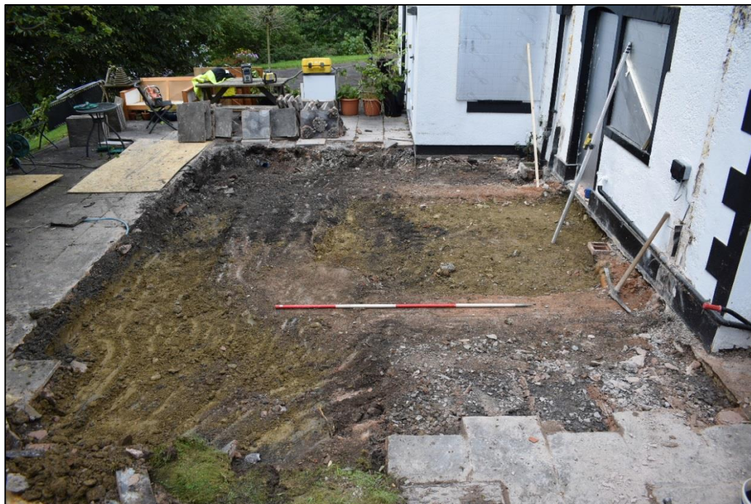
Fig. 4: The area of the new extension after the concrete base of the former extension was removed, from the south-west. (CPAT 4389-0001)
