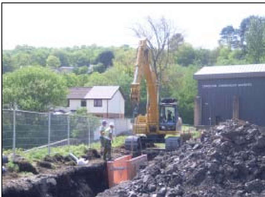
Plate 57 Excavation of a pipe trench close to the southern limit of the site, looking west towards Maesteg Sports Centre
