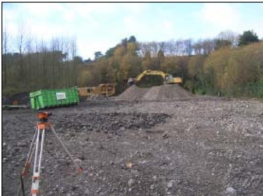
Plate 14 Looking west across the site of the former 'Cornstores Industrial Estate', after the demolition of the two modern buildings
