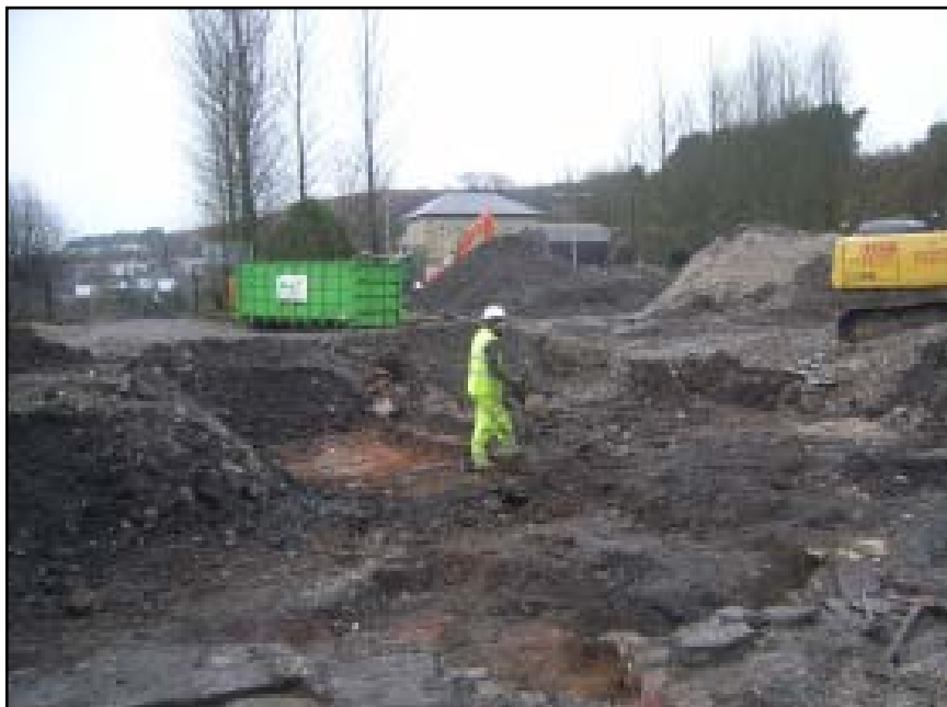
Plate 17 View south-west across the northern end of the excavated remains of the 'new puddling' (forge) building
