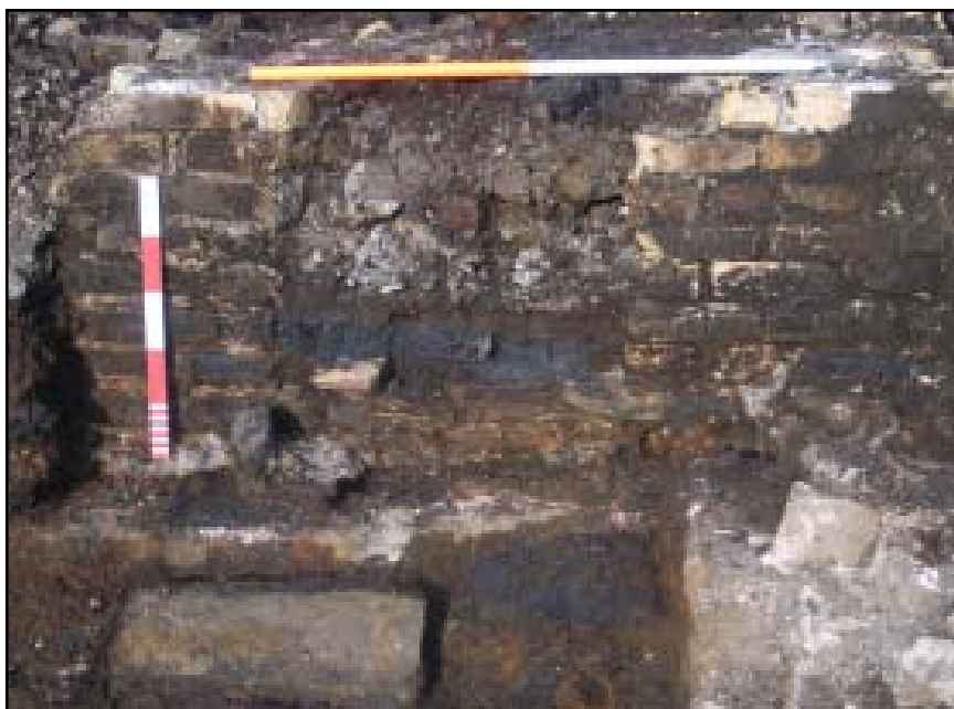
Plate 39 South-facing section in brick-built flue 101. Note cast iron tuyere reused in the construction of flue 317 (left foreground)
