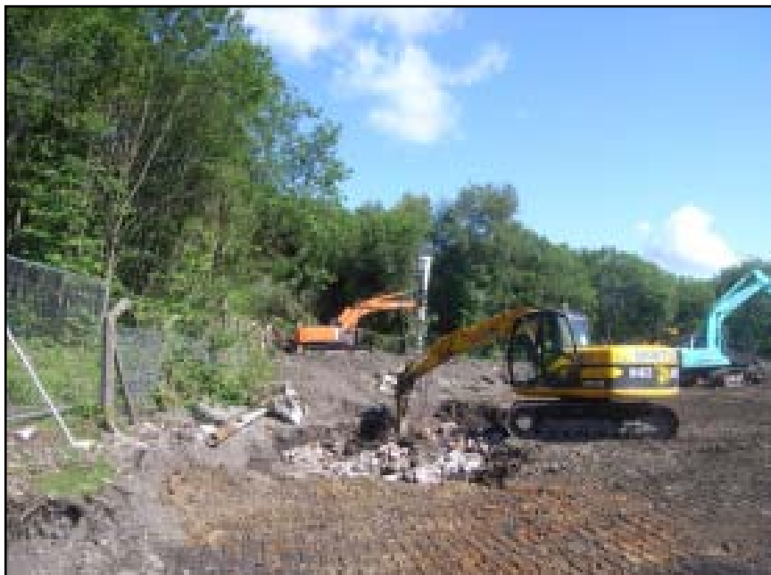
Plate 59 View of ground work in progress in the vicinity of the former casting house, close to the western site boundary, looking north-west
