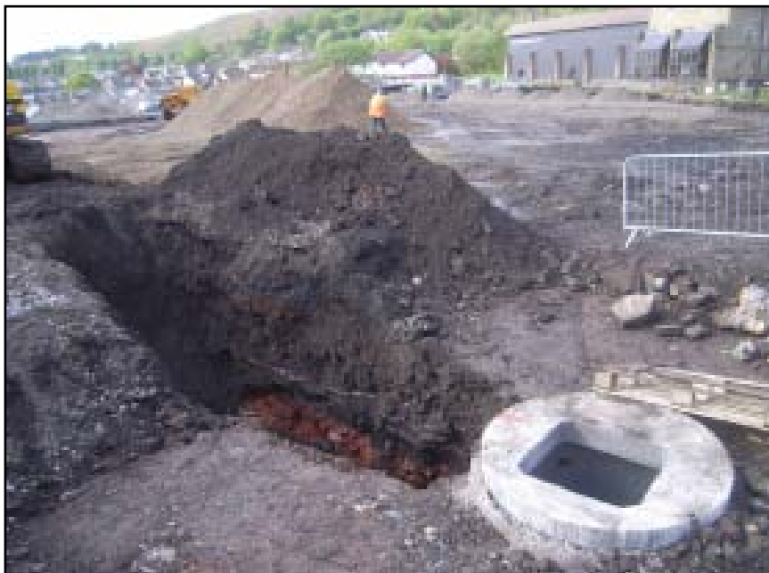
Plate 56 Excavation of a pipe trench across the former rugby club car park, looking south
