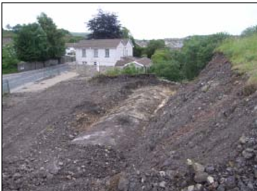
Plate 63 Looking south-east at the exposed roof of a mid 19th-century stone-built tunnel through which flows the river Llynfi. It is the surviving remnant of a three-arched railway bridge that carried a line to/from the Llynfi Vale ironworks
