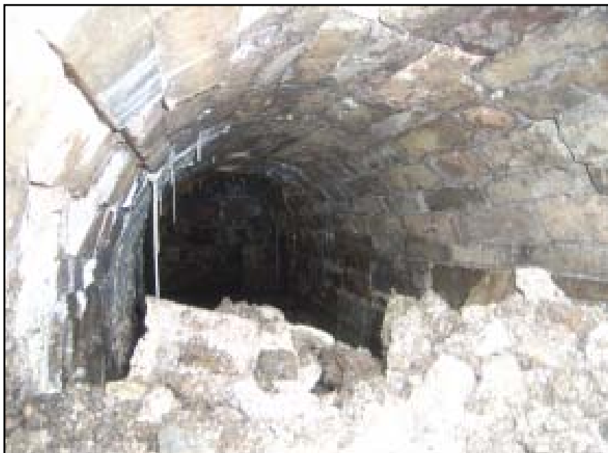
Plate 62 A view within the flue-like structure. The lack of any signs of heat affected brickwork indicates that it may have been an air duct
