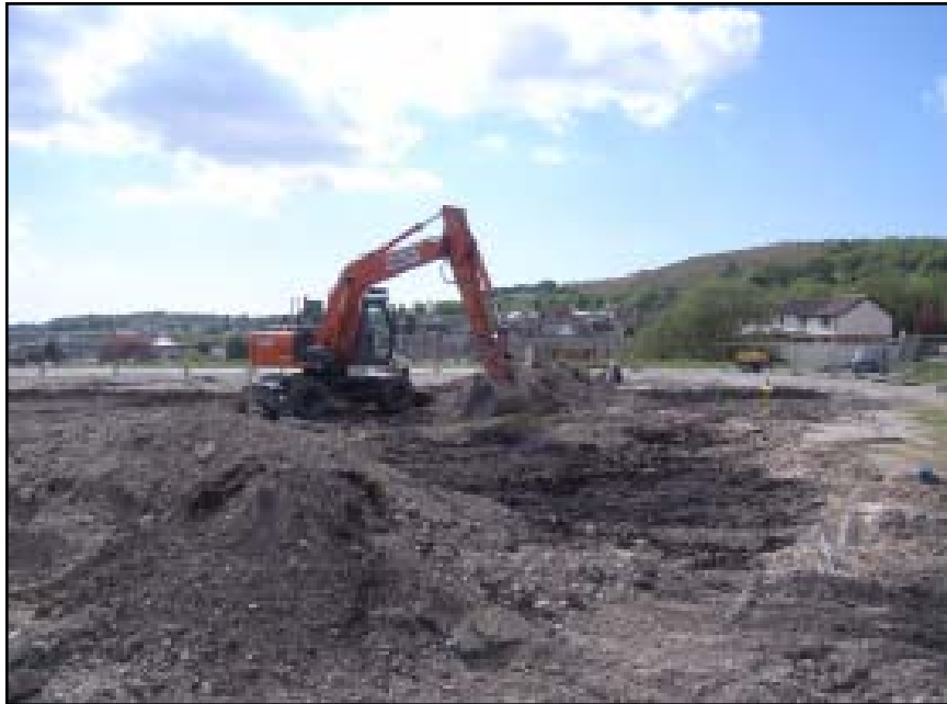
Plate 52 Ground reduction work in progress, looking south-west across former rugby club car park
