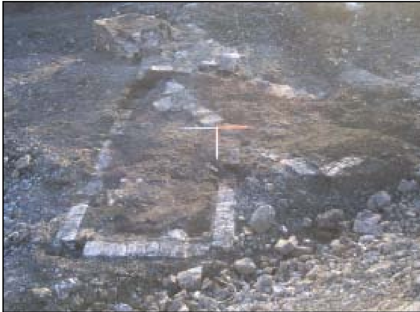
Plate 37 View east, of a brick reverberatory furnace structure (contexts 299/302/304), a chimney base (312) and a pier base (132) within the former 'new puddling' (forge)
