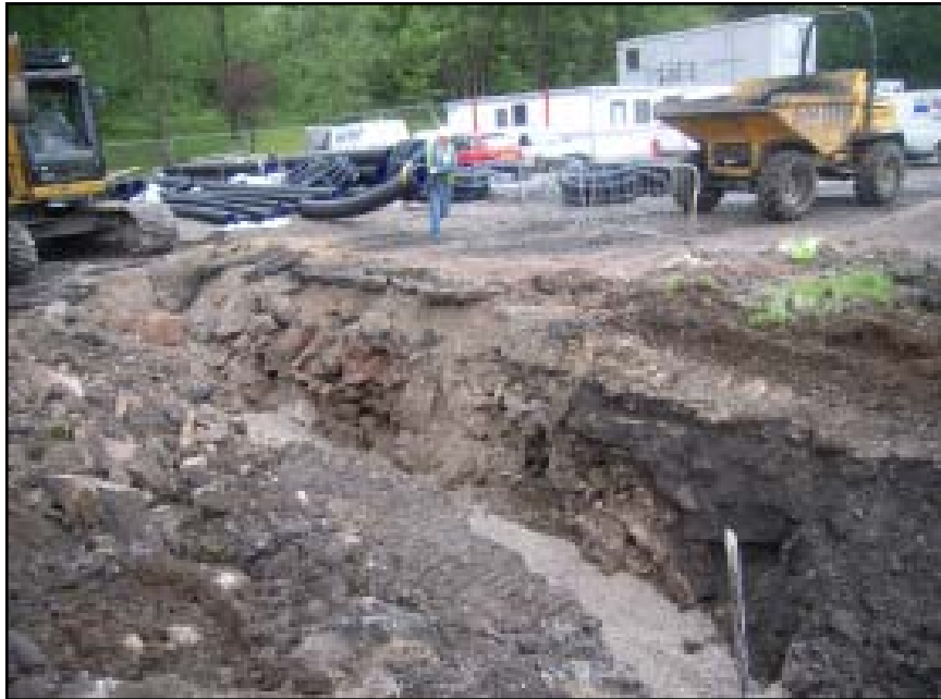
Plate 58 Excavation of a pipe trench across the sports centre car park. It exposed much redeposited sandstone masonry used to infill partially demolished brick built tunnel
