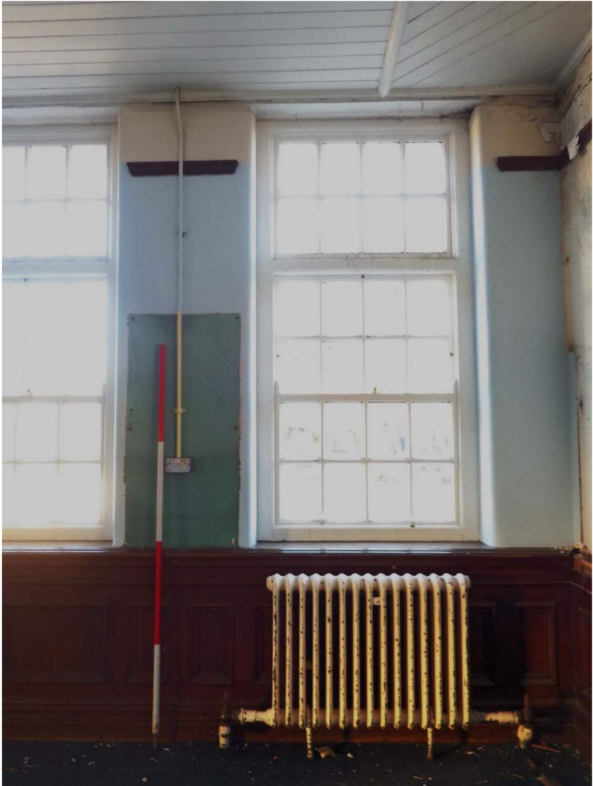
Plate 118: First Floor, view of Seminar 3 with original skirting board and fittings; shot facing north.
