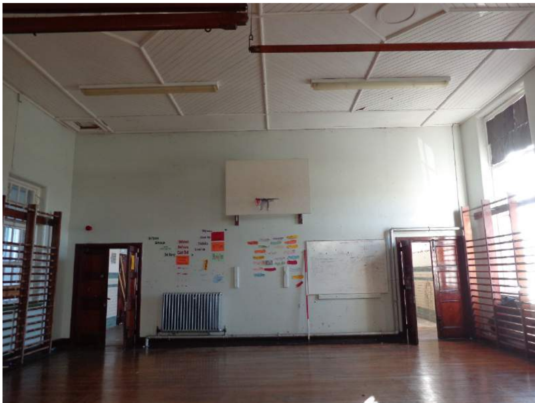
Plate 70: View of gymnasium (10) with original fittings and accesses to boys' lockers (9A); shot facing south.
