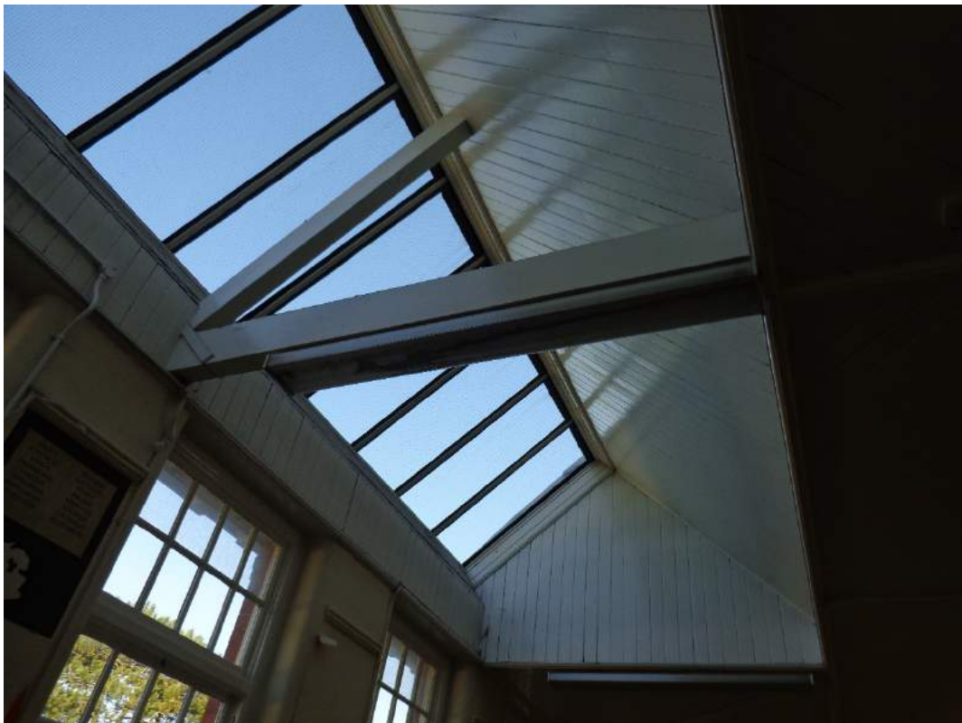
Plate 108: First Floor, view of Seminar 1 with original fittings and roof-light; shot facing northeast.
