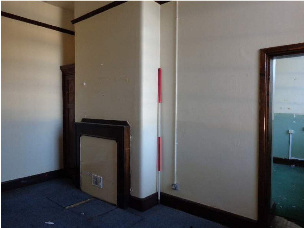
Plate 49: View of Community Office (25), with access to next Community Office (24); shot facing northwest.
