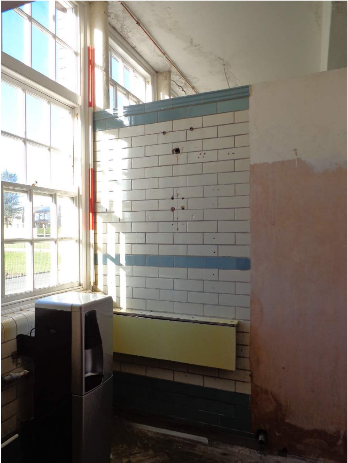
Plate 66: View of walled steam room from girls' lockers room (11); shot facing northwest.
