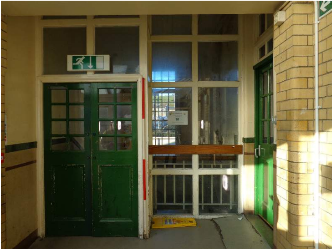
Plate 104: View of northern staircase, access to first floor, door and window; shot facing north.
