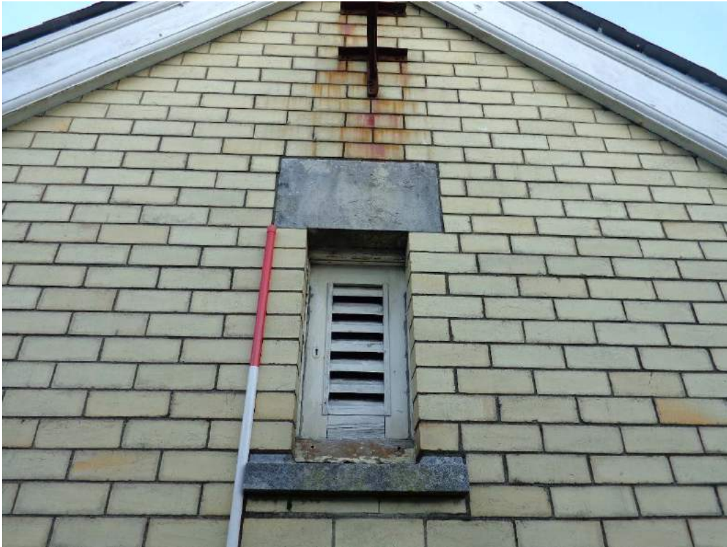
Plate 145: Roof, view of small vent and wooden blind at yellow brick gable; shot facing west.
