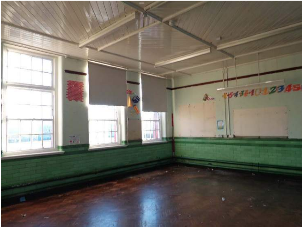
Plate 137: First Floor, view of Business Studies 5 with original fittings; shot facing southwest.
