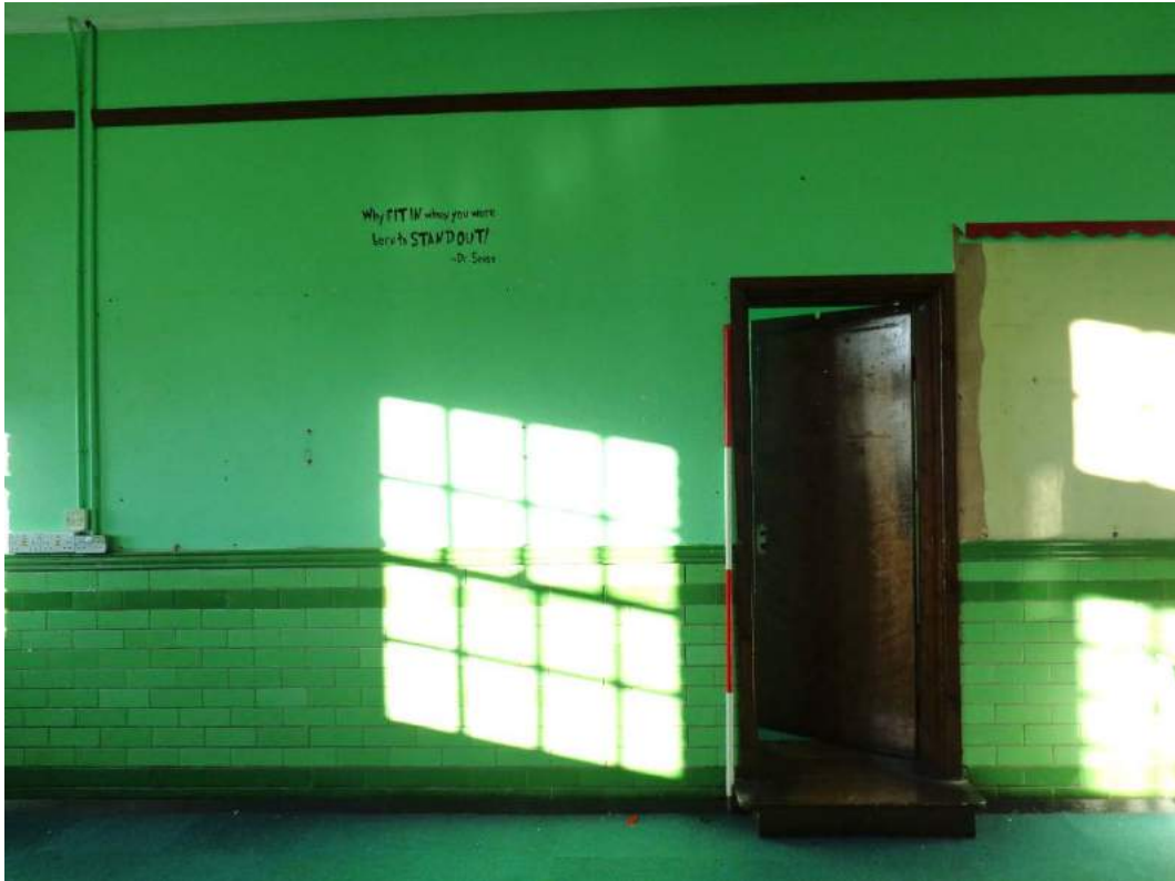
Plate 114: First Floor, view of Breakout area 1 and access from Storage room 2; shot facing north.
