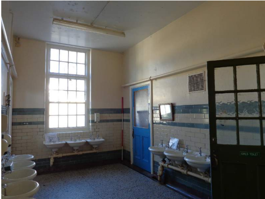
Plate 60: View of girl's toilet lobby (34), with access to girls' WC (14); shot facing northeast.
