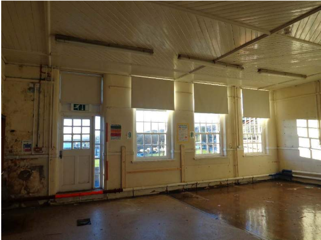
Plate 141: First Floor, view of Breakout Area 2, with fitted door to fire exit; shot facing west.
