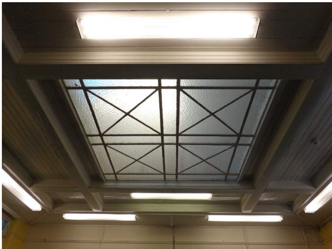
Plate 126: First Floor, view of glazed roof-light at central area of Staff Work room; shot facing to the roof.
