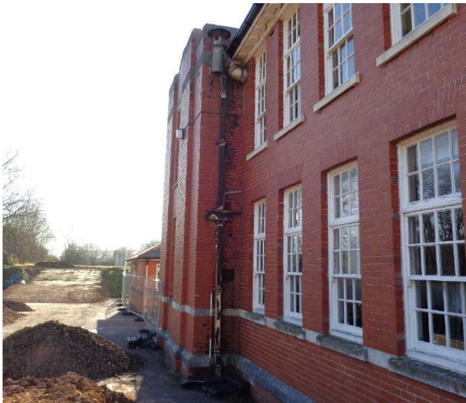
Plate 6: Frontal E façade, view of northern side and drainpipe; shot facing south.
