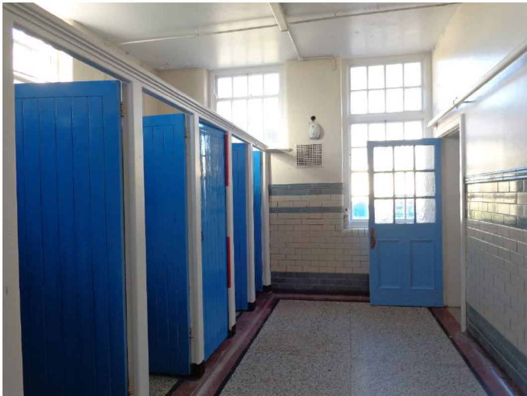
Plate 61: View of girl's WC (14), with access to girls' toilet lobby (34); shot facing north.
