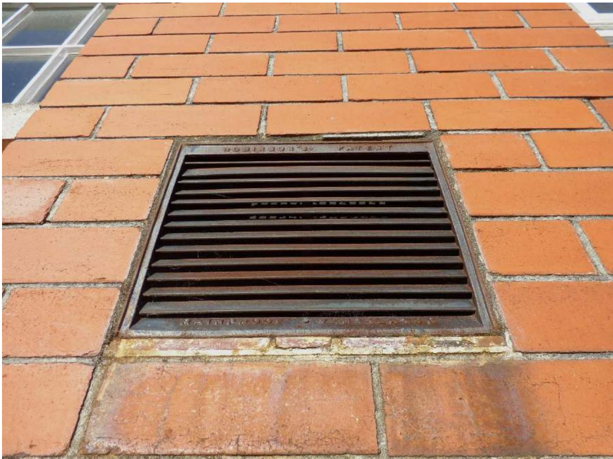
Plate 40: Boys S façade, detail of cast iron vents, located in all sides; shot facing north.
