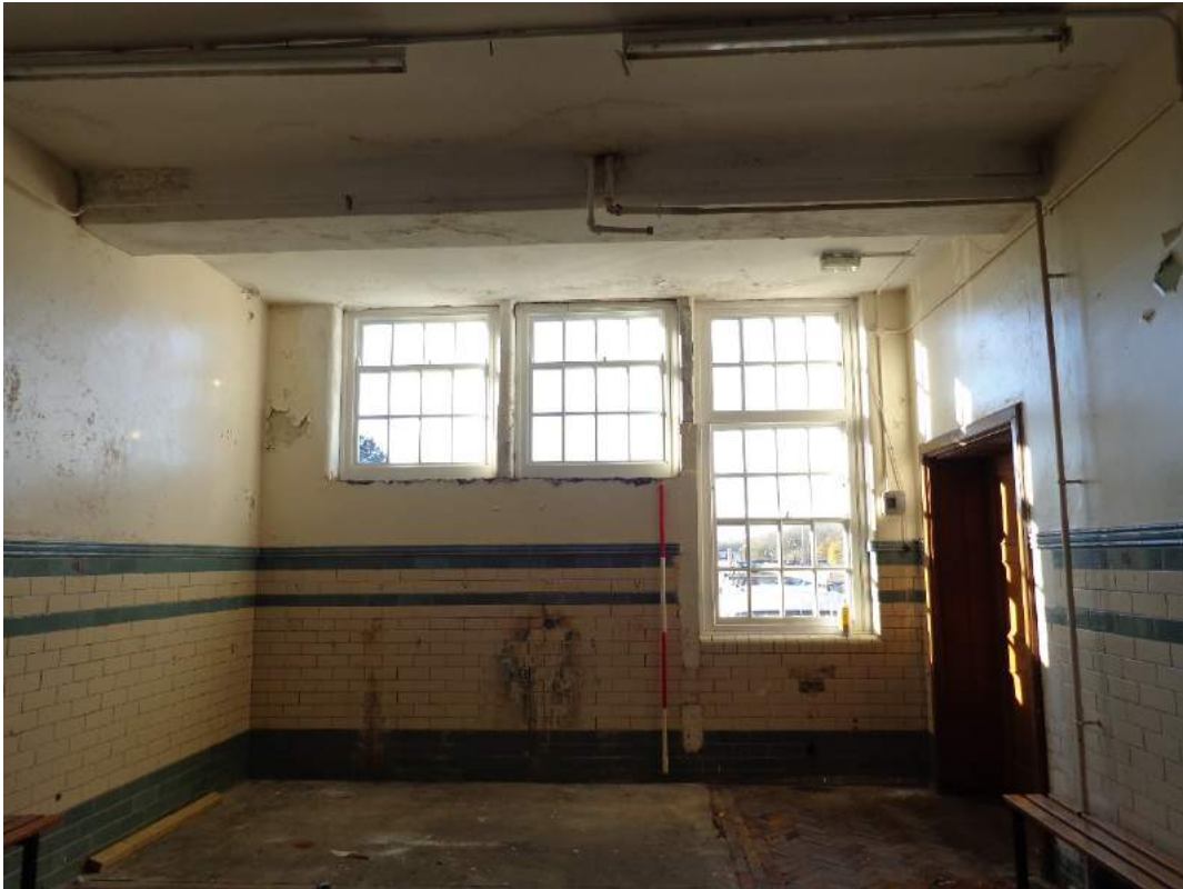
Plate 73: View of boys' lockers room (9A), with access from the gymnasium (10); shot facing west.
