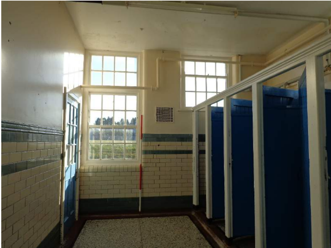
Plate 80: View of boys' WC (7), with access to boys' WC lobby (8); shot facing south.
