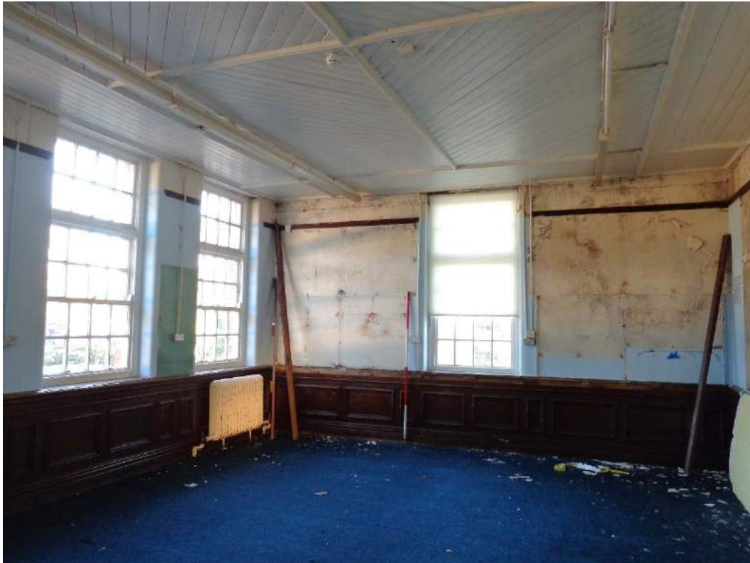
Plate 116: First Floor, view of Seminar 3 with original skirting board and fittings; shot facing northeast.
