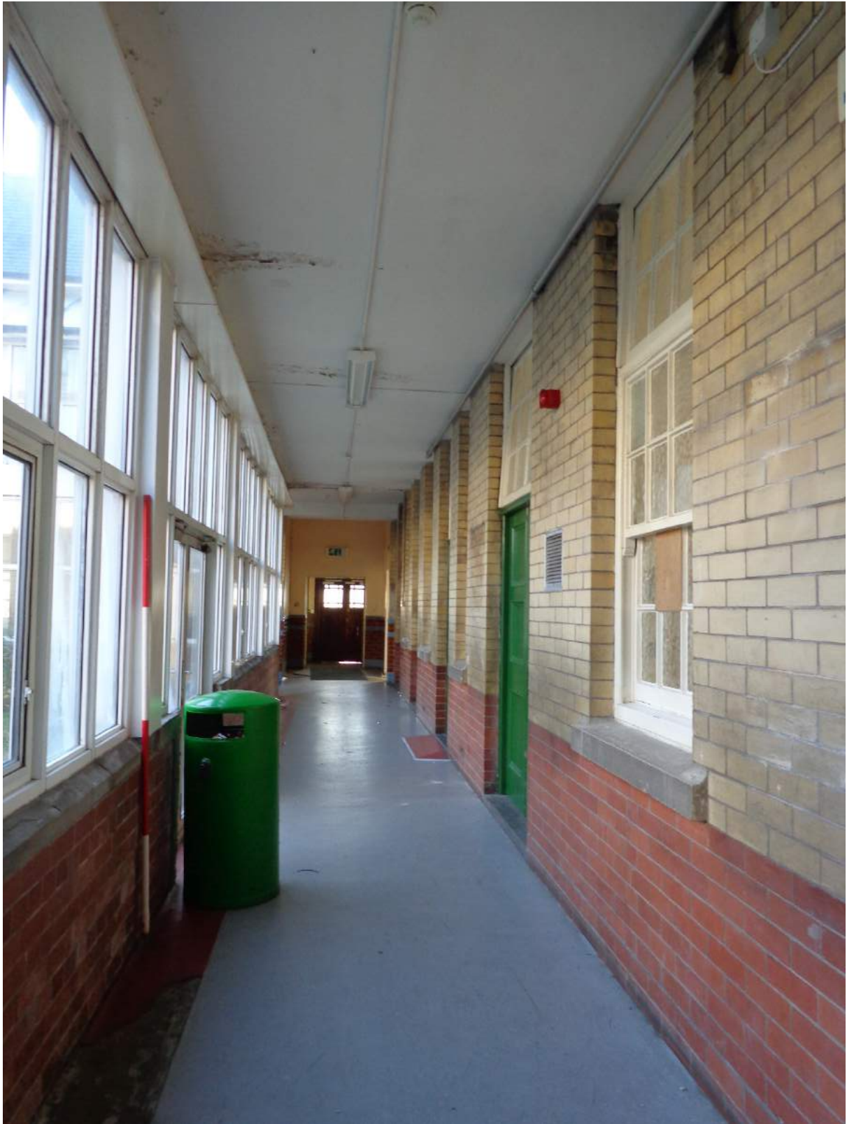
Plate 72: View of corridor (35) southwest, which gives access to (9A), (9), (8) and (6), and boys' western entry hall (95) at the end; shot facing south.
