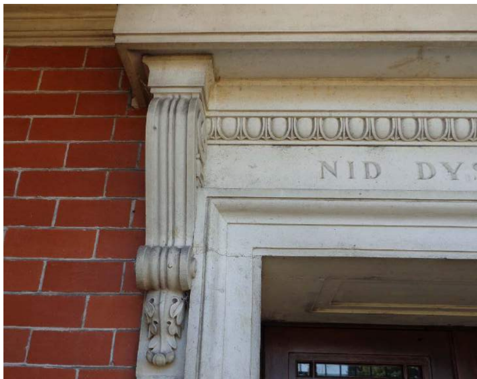
Plate 34: Front E façade, main entrance door, detail of decorations; shot facing west.
