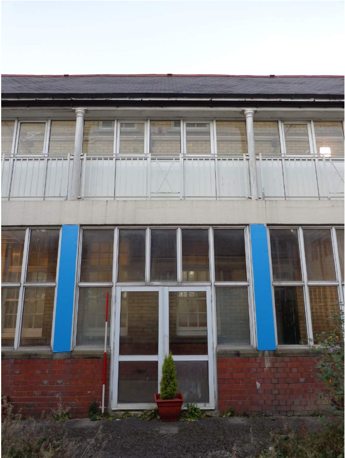
Plate 150: Courtyard 2, detail view of access, windows and first floor; shot facing east.
