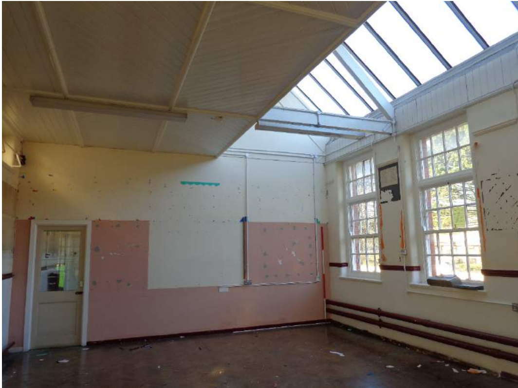
Plate 107: First Floor, view of Seminar 1 with original and new fittings; shot facing northwest.
