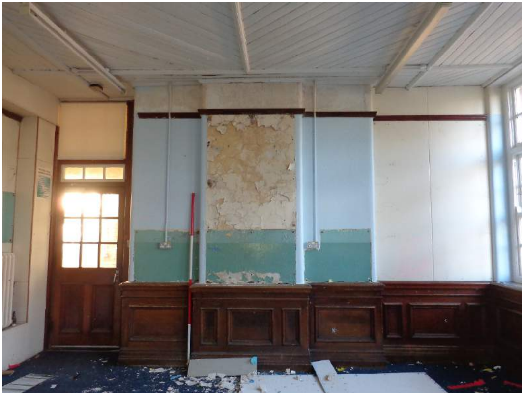
Plate 117: First Floor, view of Seminar 3 with original skirting board and fittings; shot facing west.
