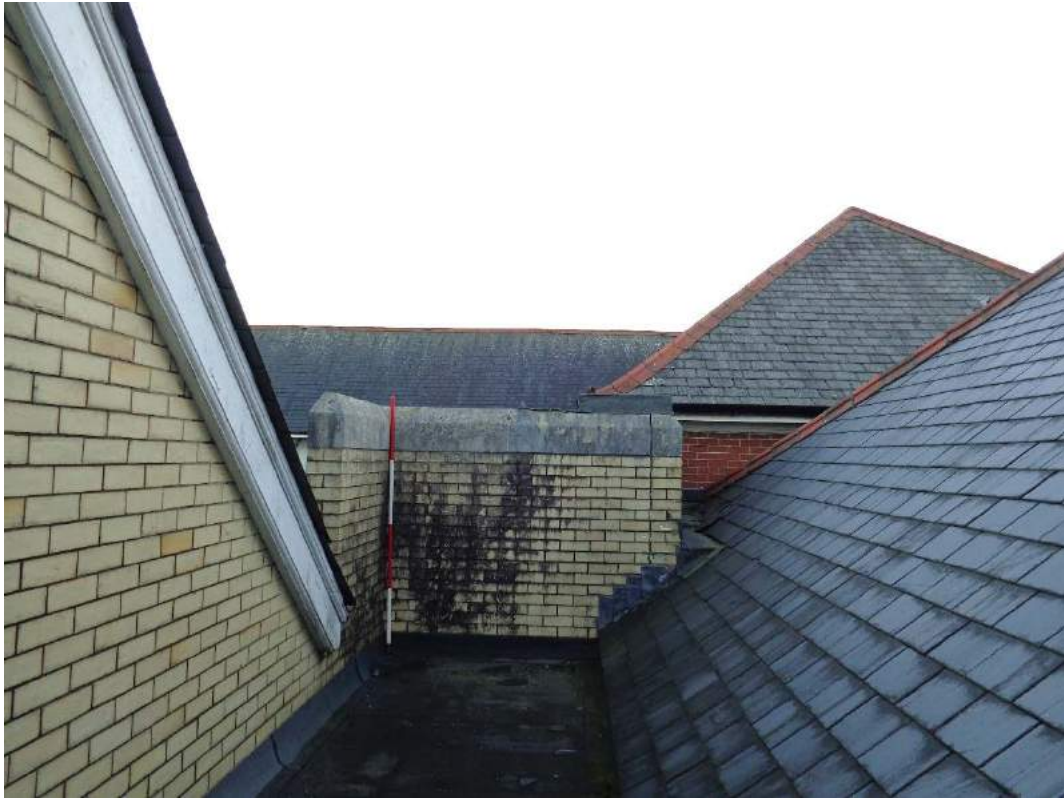
Plate 143: Roof, view of flattened access, yellow brick gable and cross-hip, slate tiled roofs; shot facing south.
