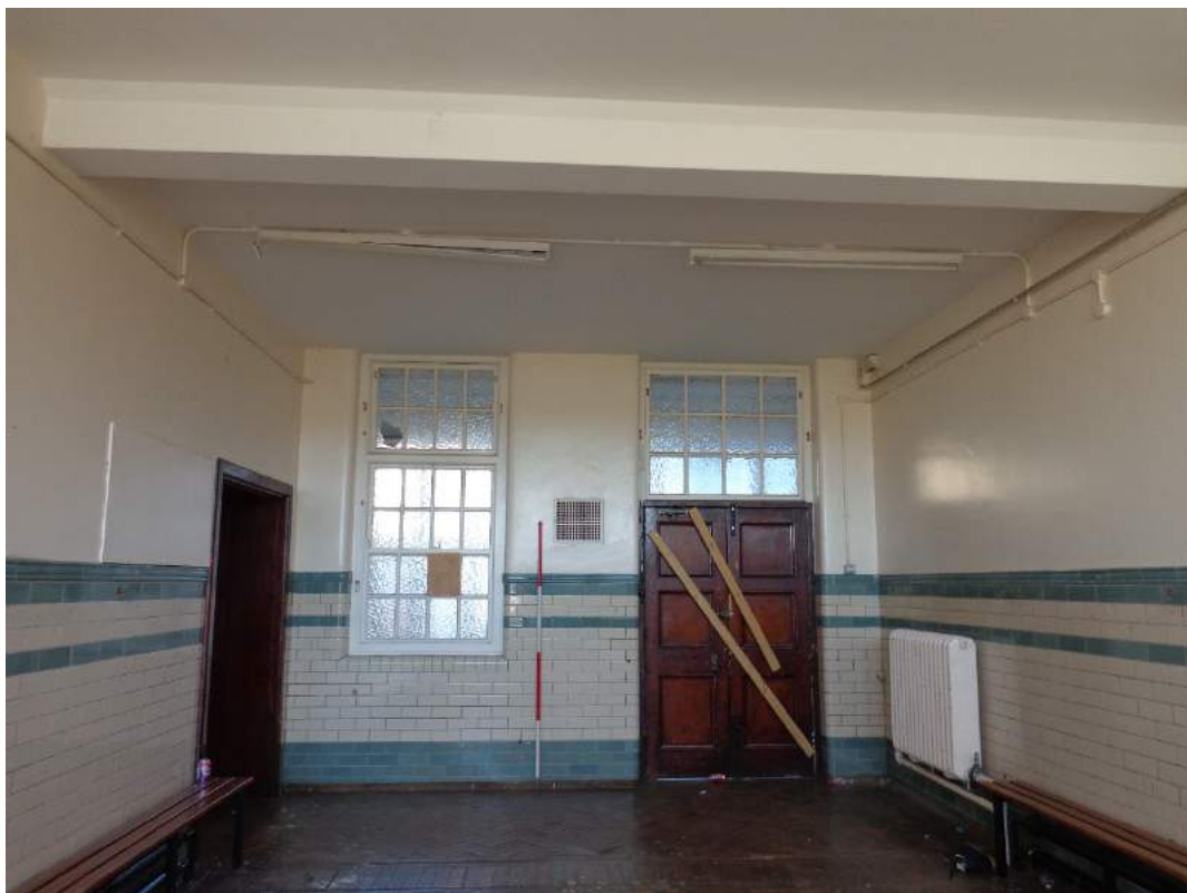
Plate 74: View of boys' lockers room (9A), with access from the gymnasium (10); shot facing east.
