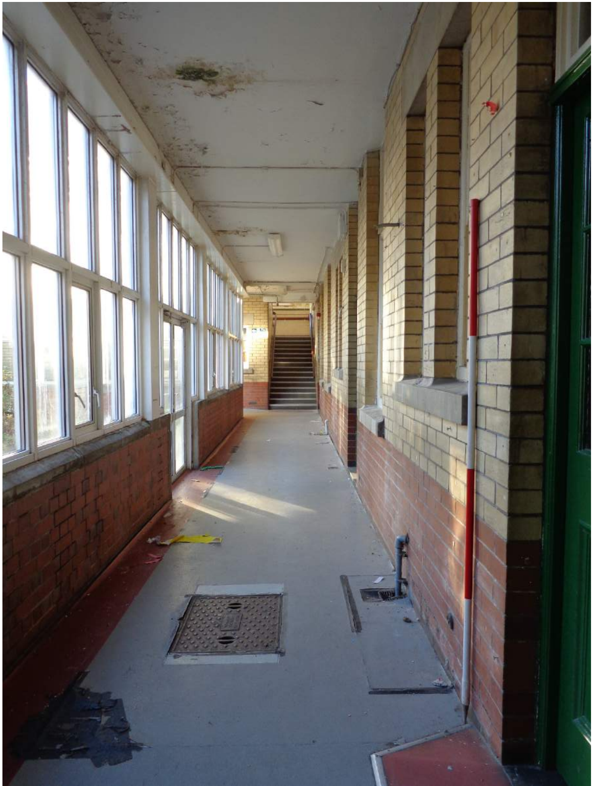
Plate 48: View of corridor (63) east section, gives access to (25), (24), (21) and north stairs; shot facing north.
