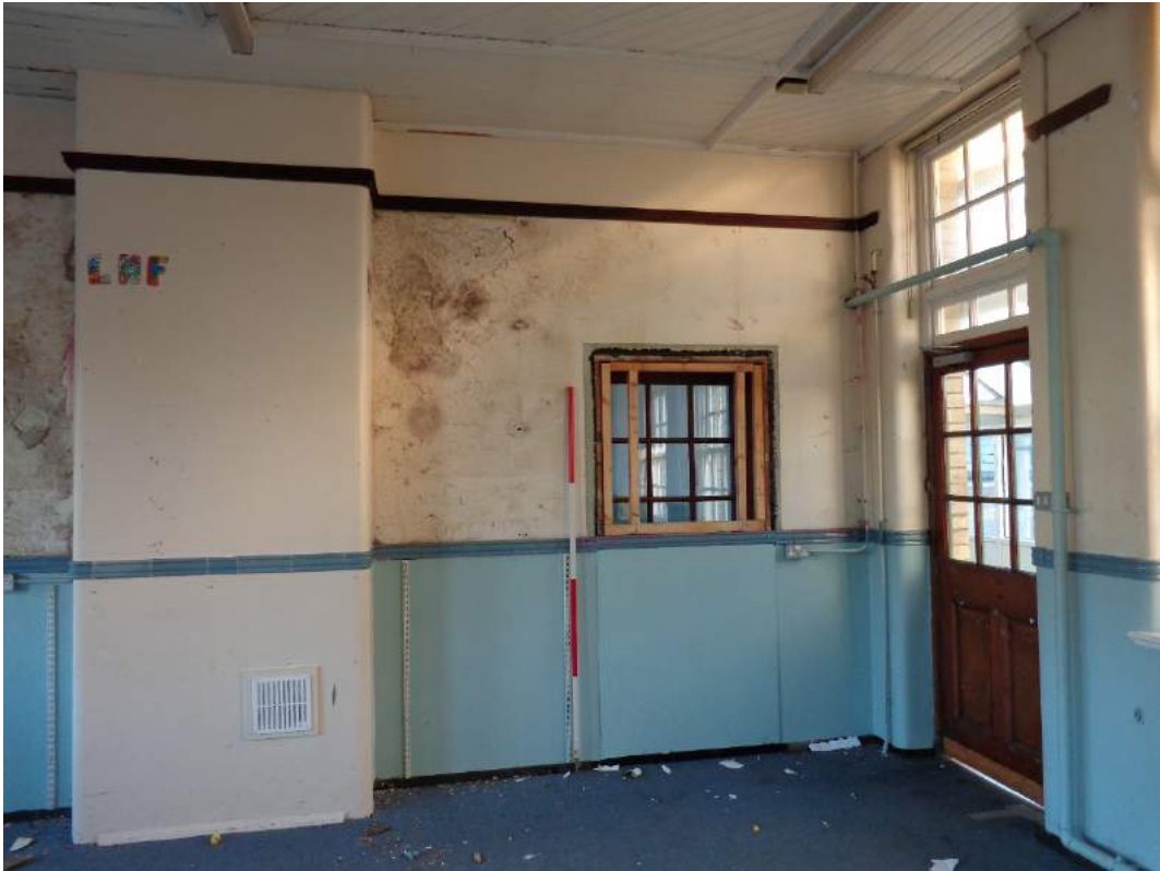
Plate 121: First Floor, view of Business Studies 1, with blocked off door and chimney fitting; shot facing south.
