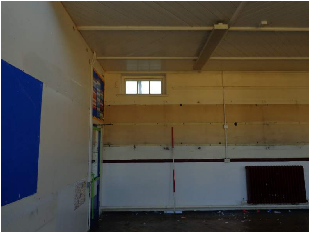
Plate 110: First Floor, view of Seminar 2 with original fittings and small window; shot facing south.
