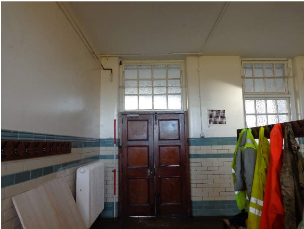
Plate 65: View of girls' lockers room (11) with access to corridor (63) west; shot facing east.
