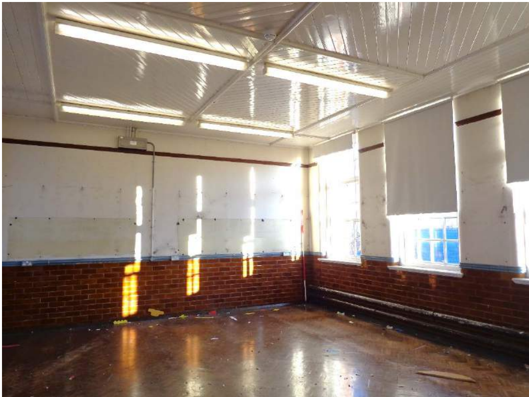
Plate 136: First Floor, view of Business Studies 4 with original fittings; shot facing southeast.
