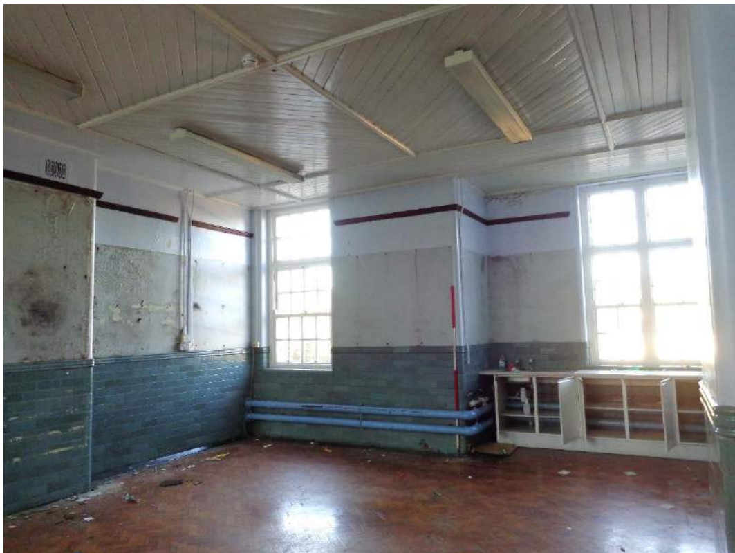
Plate 122: First Floor, view of Seminar 4, with original and modern fittings; shot facing east.
