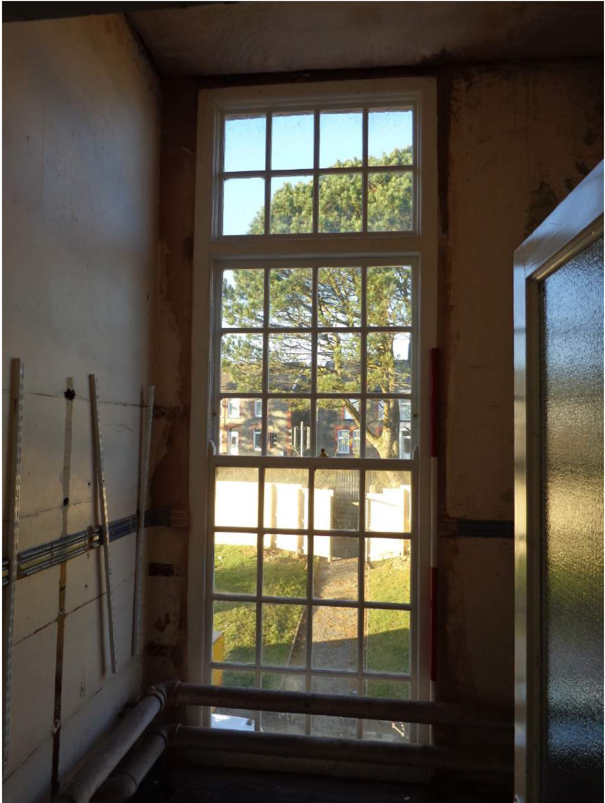
Plate 111: First Floor, view of Storage room 1 with original and modern fittings; shot facing north.
