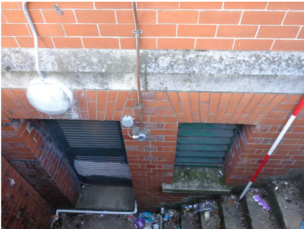
Plate 28: Girls N façade, eastern section, access to boiling room; shot facing south.
