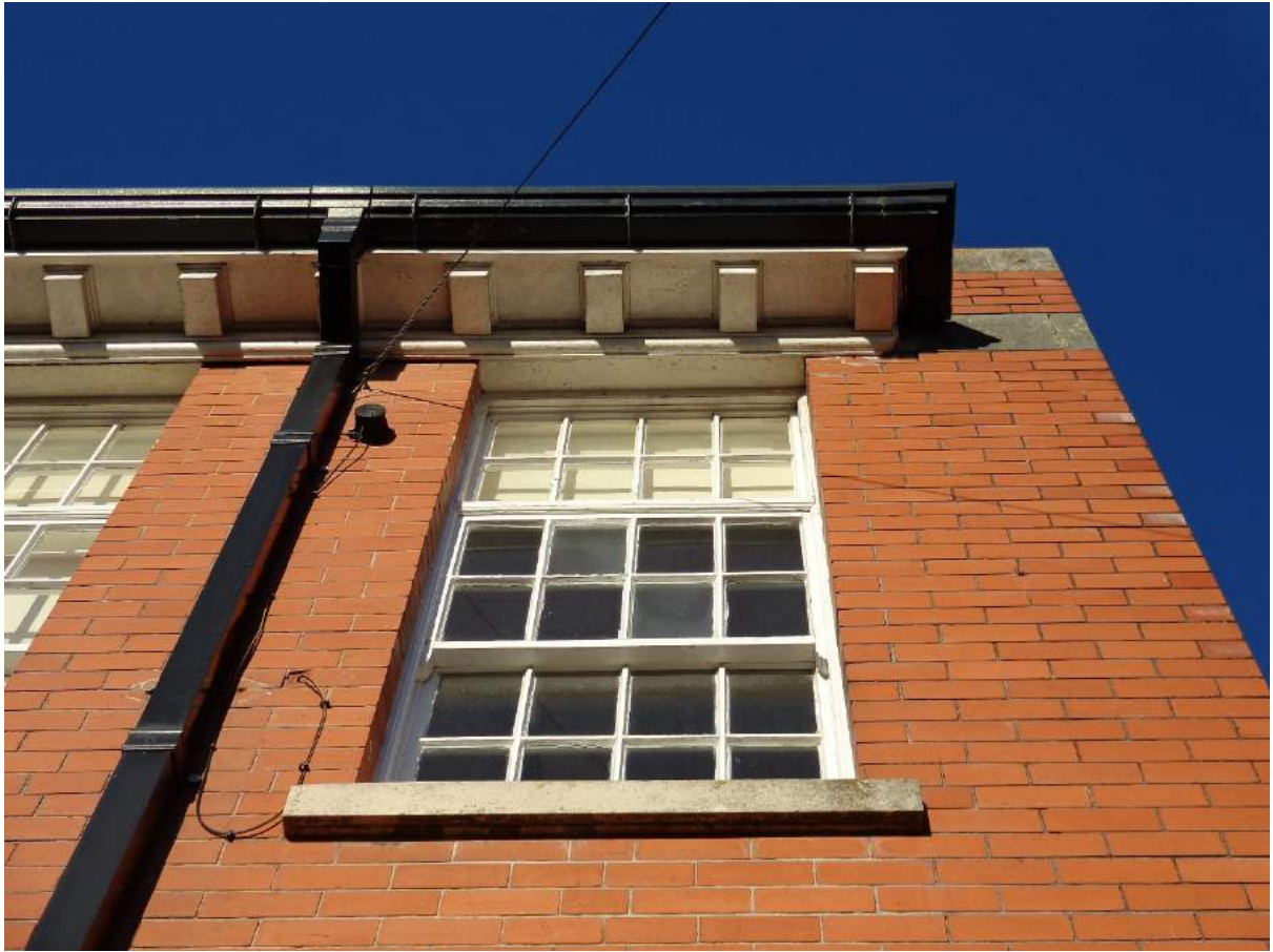
Plate 41: Boys S façade, detail of dentil decoration at top cornice, same in all sides; shot facing north.
