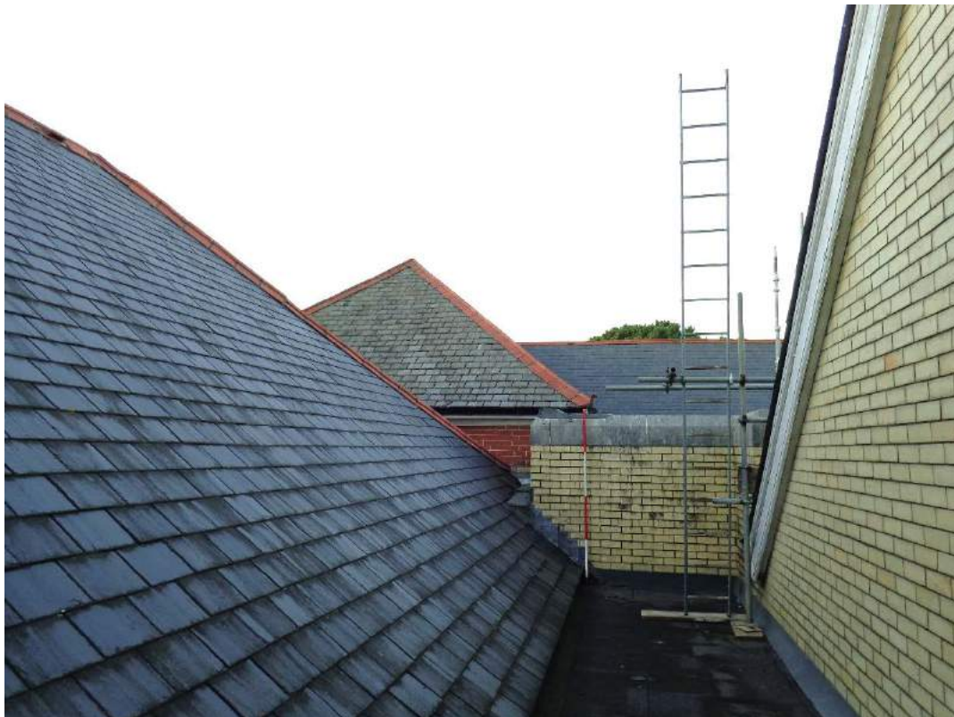
Plate 144: Roof, view of flattened access, yellow brick gable and cross-hip, slate tiled roofs; shot facing north.
