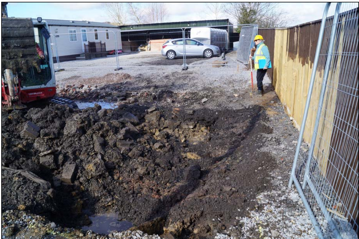
Plate 4: GVB2016_104, During removal of building rubble, 001, with clay layers, 002 and 003, just visible. Also groundwater is visible seeping into the excavated areas, looking northwest.
