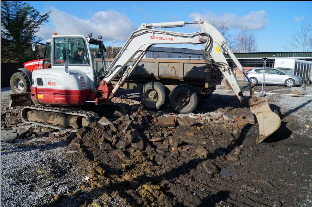
Plate 1: GVB2016_101, Starting to remove the building rubble, 001, which was shallower on the east and northern sides of the area excavated, looking west.
