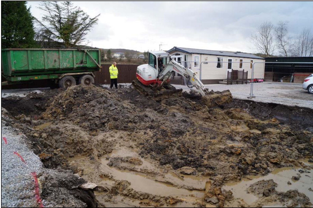
Plate 7: GVB2016_107, as excavation progressed across the plot, the groundwater became more of a problem and the clay subsoils became liquid, looking west.
