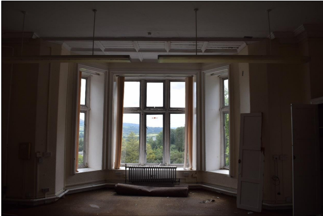
Fig. 36: The interior view of the bay window on the first floor at the western end of the historic core (Fig.12, F6). CPAT 4537-0099
