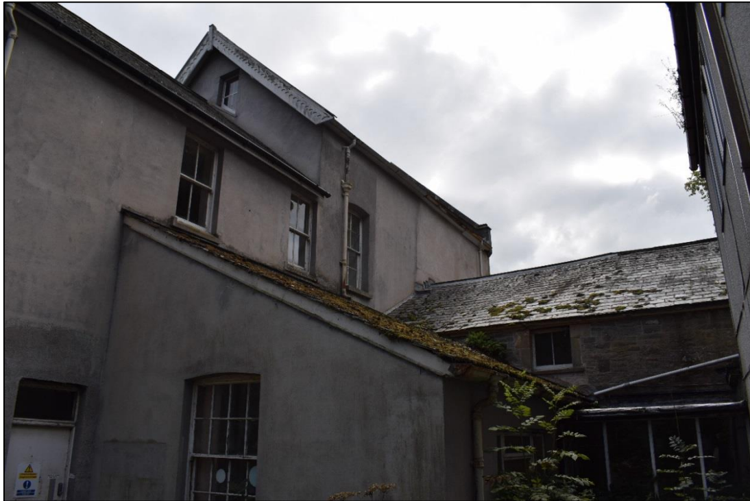
Fig. 20: Close up view, showing the junction between the historic core of the building (centre top) and the piecemeal later additions on its west and north. CPAT 4537-0041
