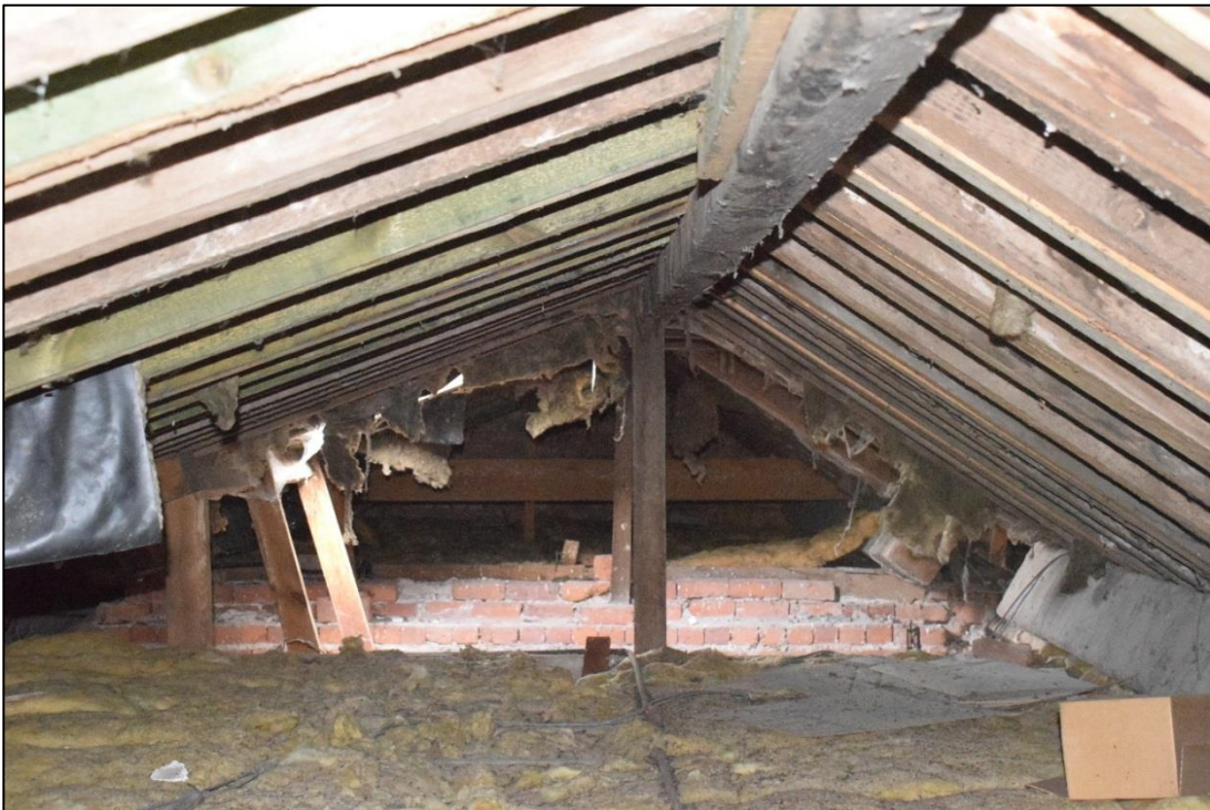
Fig. 43: The roof space above the central part of the historic core, visible through a hatch in room S6. CPAT 4537-0124
