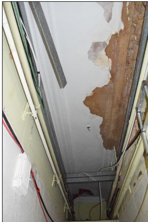
Fig. 33: Ornamental mouldings in the passage behind the rooms on the ground floor of the historic core (Fig. 11, G22). CPAT 4537-0152
