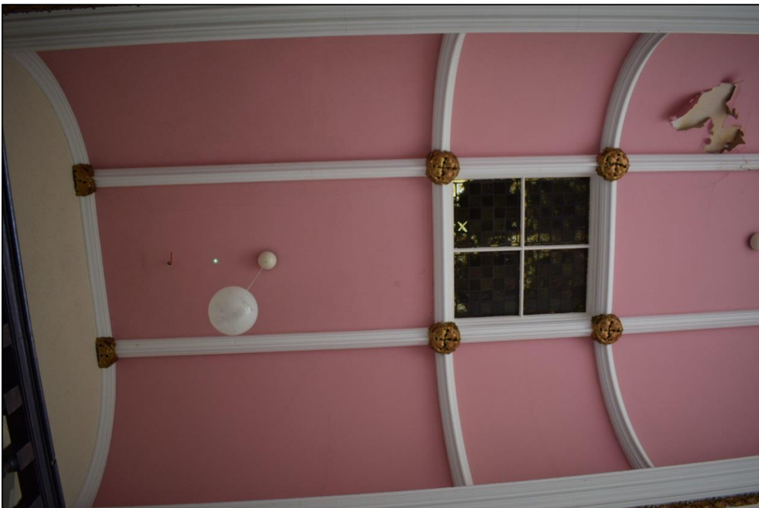
Fig. 35: Ornamental mouldings and roof light above the entrance hall (Fig. 11, F20). CPAT 4537-0086
