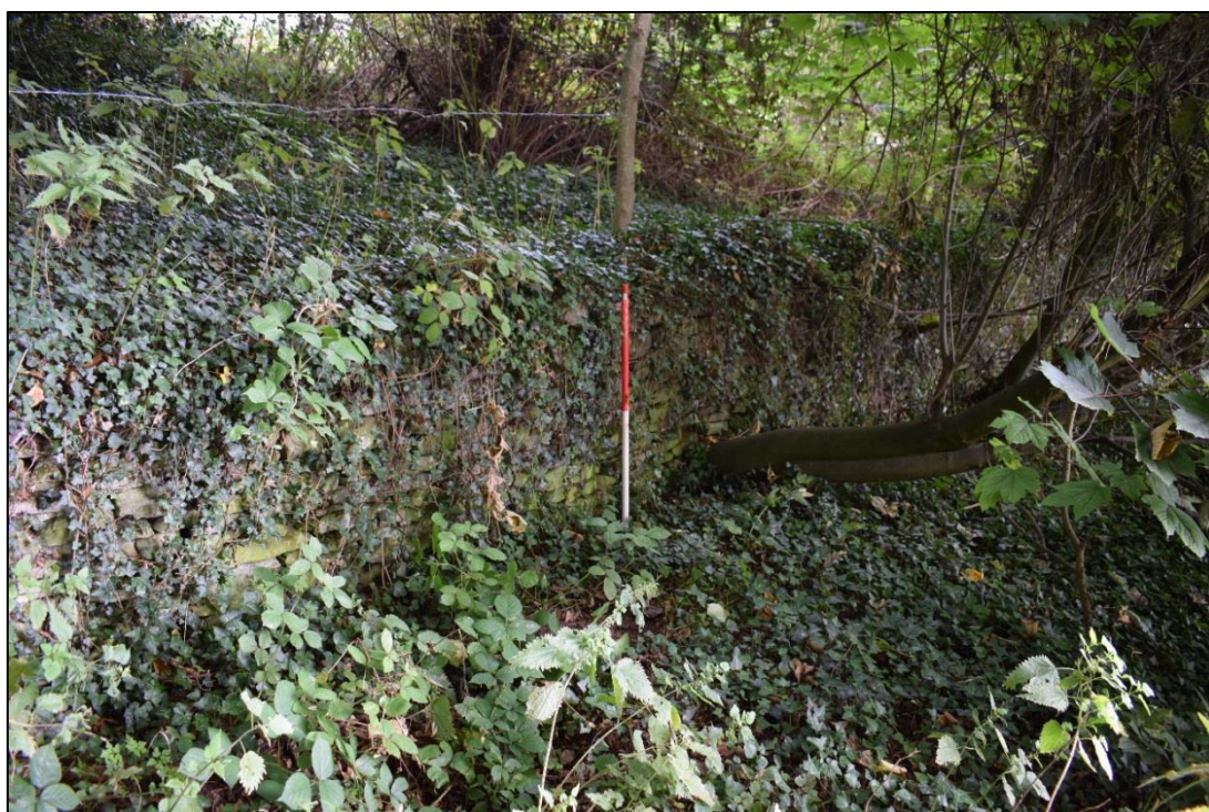
Fig. 55: The ha-ha to the south of the hall, showing tree damage. CPAT 4537-0006
