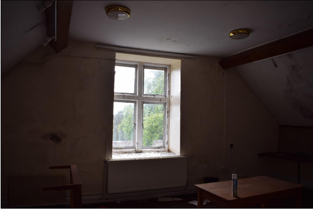
Fig. 42: The main second floor room at the west end of the historic core (Fig.13, S6)
