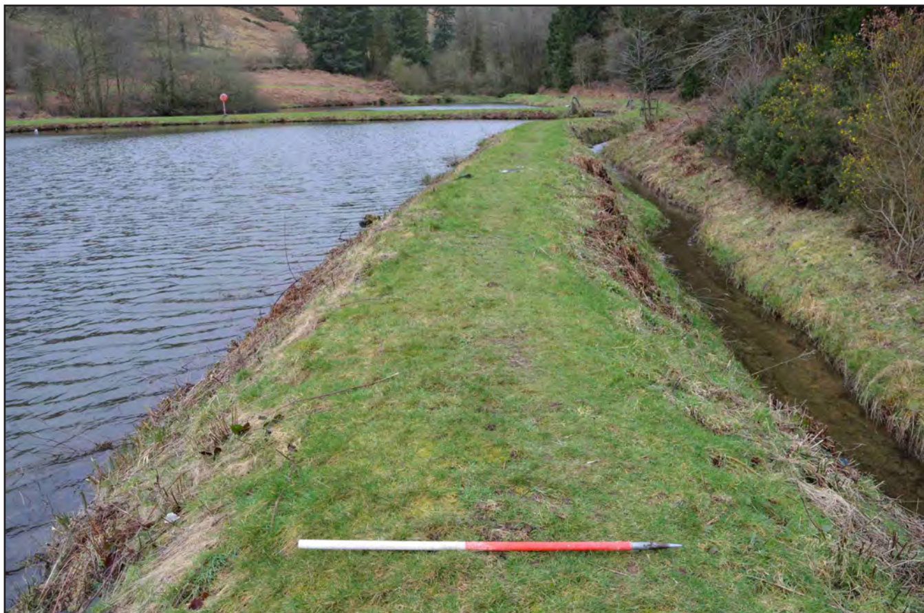
Plate 07: Embankment running to the north of both reservoirs; scale 1x1 m (archive reference: G2597_013)
