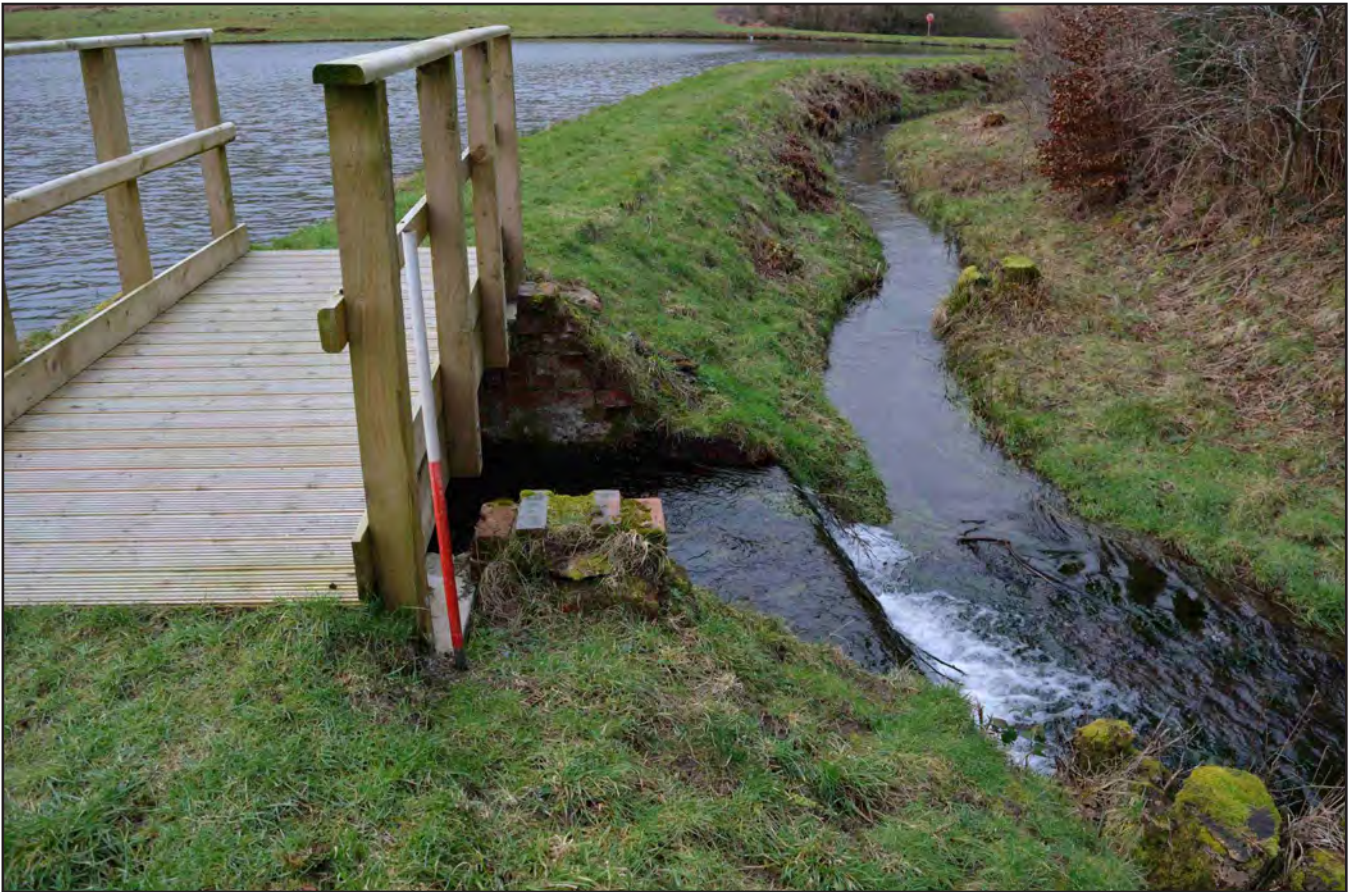
Plate 05: Brick and concrete construction of spillway access; scale 1x1m (archive reference: G2597_009)
