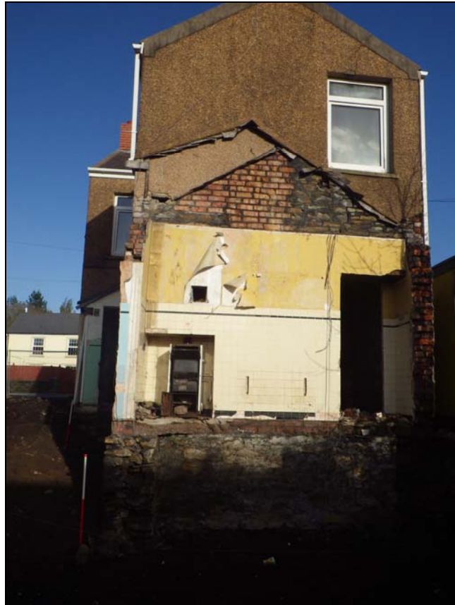
Plate 1: CSL2013_101: Back of the house after removal of the previous extension revealing the stone foundations of the house and brick and stone above, looking north northwest.
