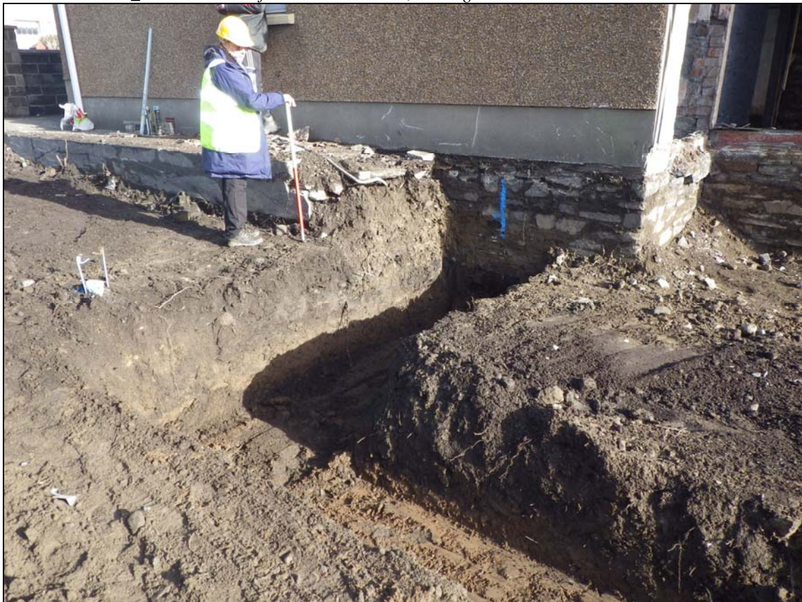
Plate 6:CSL2013_106: Looking at the northern foundation trench and the remains of a raised concrete path to its north, looking northeast.
