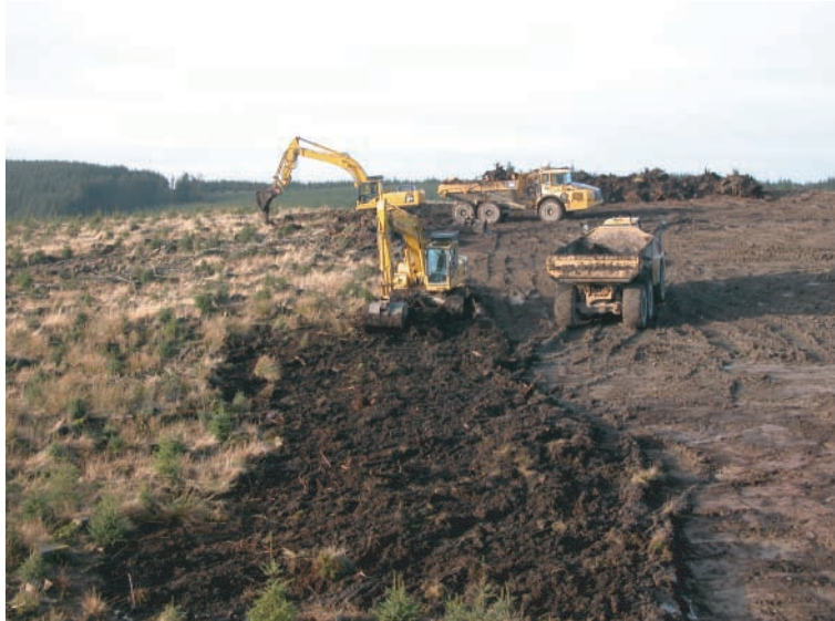
Plate 13. Working shot during top soil stripping in area of Cut 6. Looking northward.
