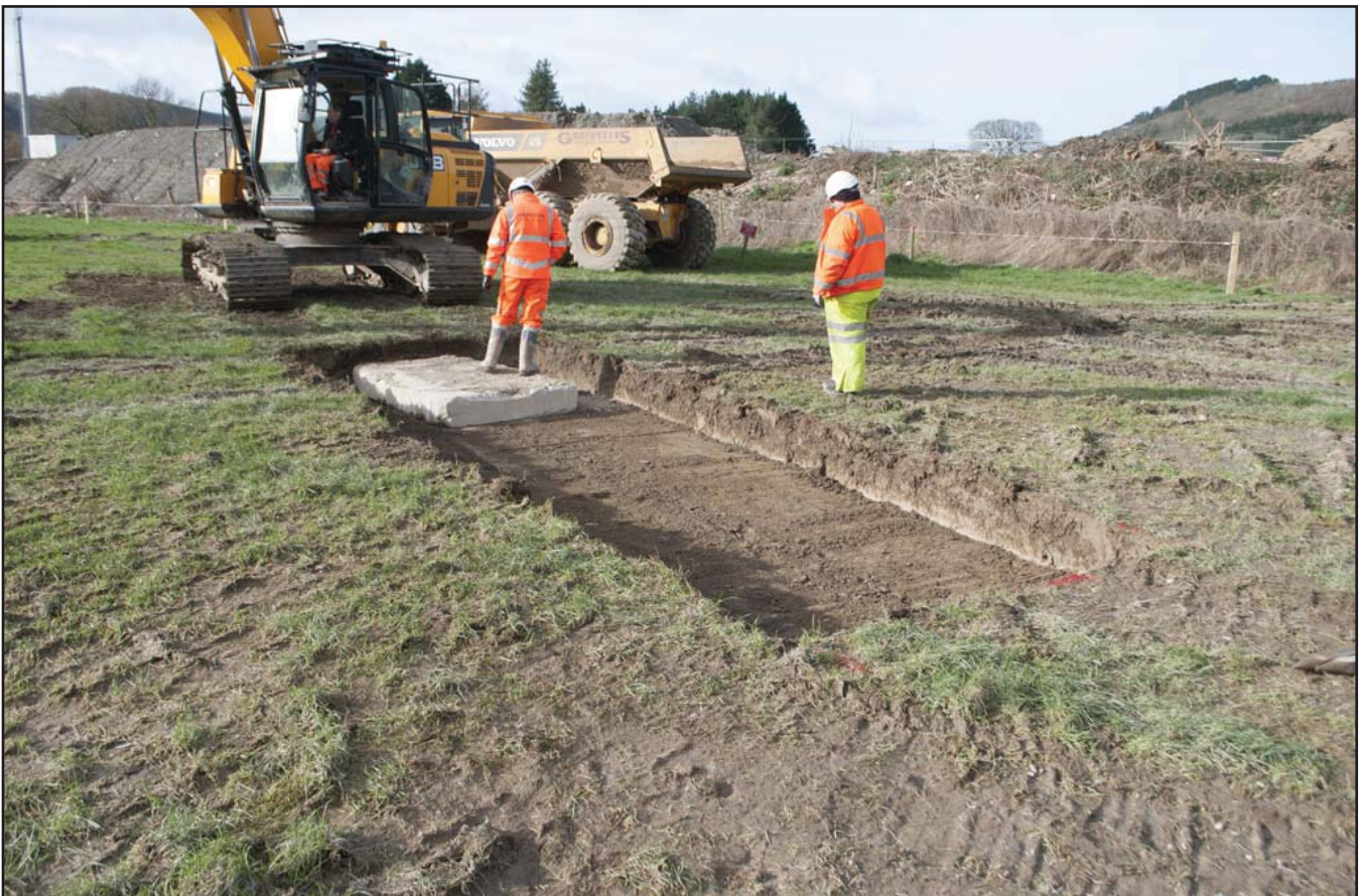
Plate 29: Working shot showing the laying of protective concrete slabs; scale not used; view from NE (archive reference: G2589_117).
