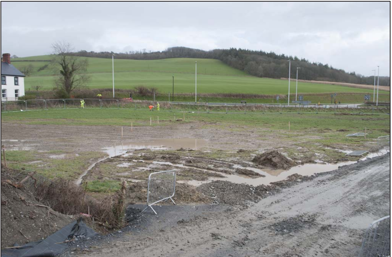
Plate 35: General view of the phase 2 topsoil strip area prior to the stripping; scale not used; view from SW (archive reference: G2589_142).
