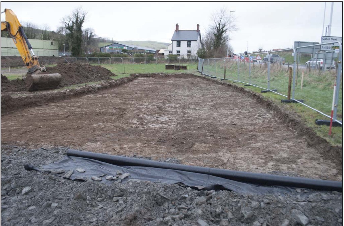
Plate 37: General view of topsoil stripping in Phase 2; scale not used; view from S (archive reference: G2589_146).
