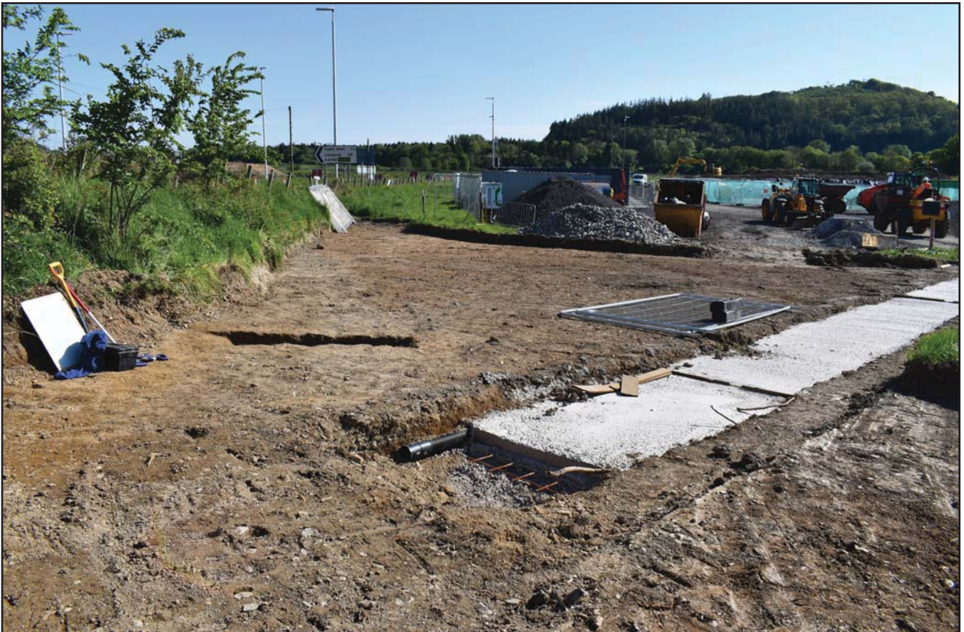
Plate 45: Ditch and concrete sewer cover; scale not used; view from NW (archive reference: G2589_187).
