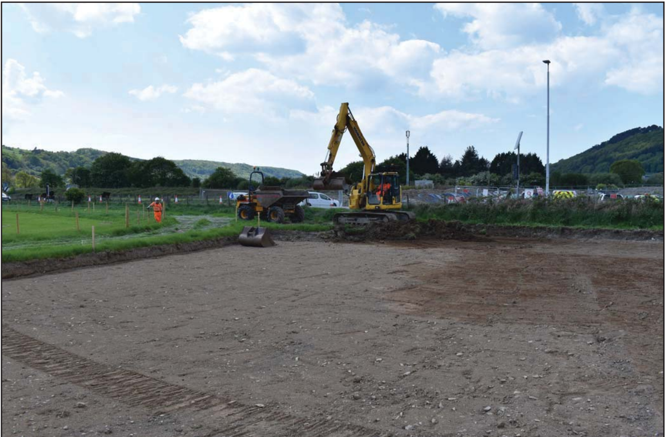
Plate 51: SW corner of area nearly finished; scale not used; view from NE (archive reference: G2589_174).
