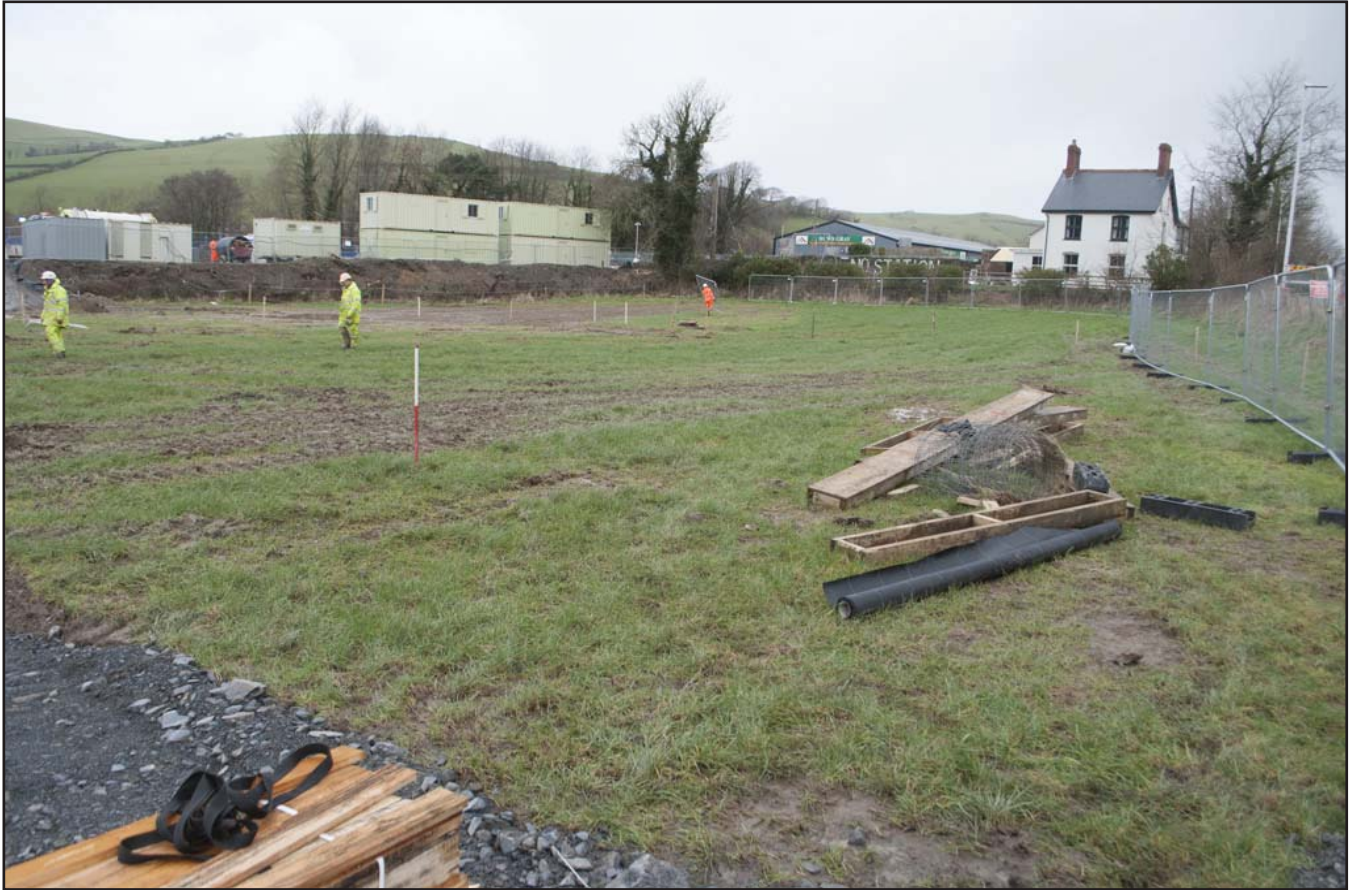
Plate 34: General view of the phase 2 topsoil strip area prior to the stripping; scale 1x1 m; view from SSE (archive reference: G2589_141).
