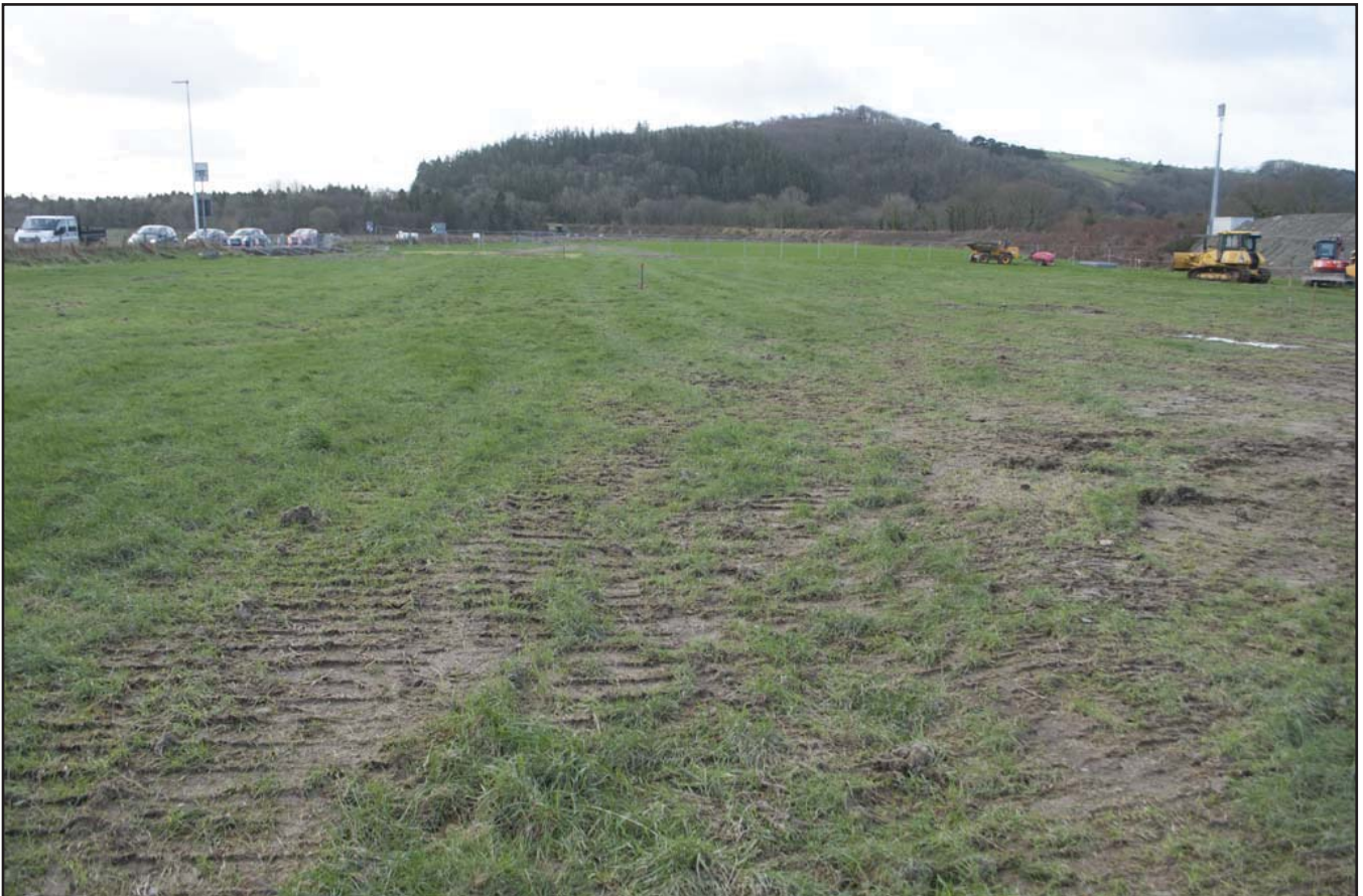
Plate 27: General view of the area to be stripped in Phase 1; scale not used; view from N (archive reference: G2589_113).
