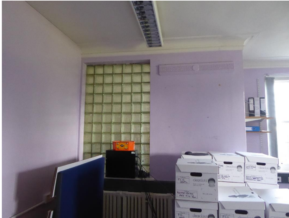
Figure. 49 same style of glazing seen in internal wall between the large south-eastern office to the centre of the 1938 enlargement and an adjacent single cell office
