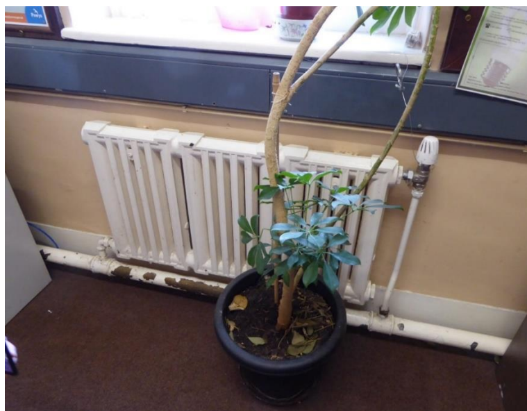
Figure 26. Original radiator seen in east/west corridor to rear
