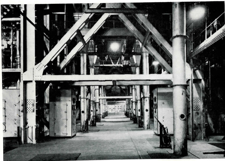
BOILER FIRING AISLE
