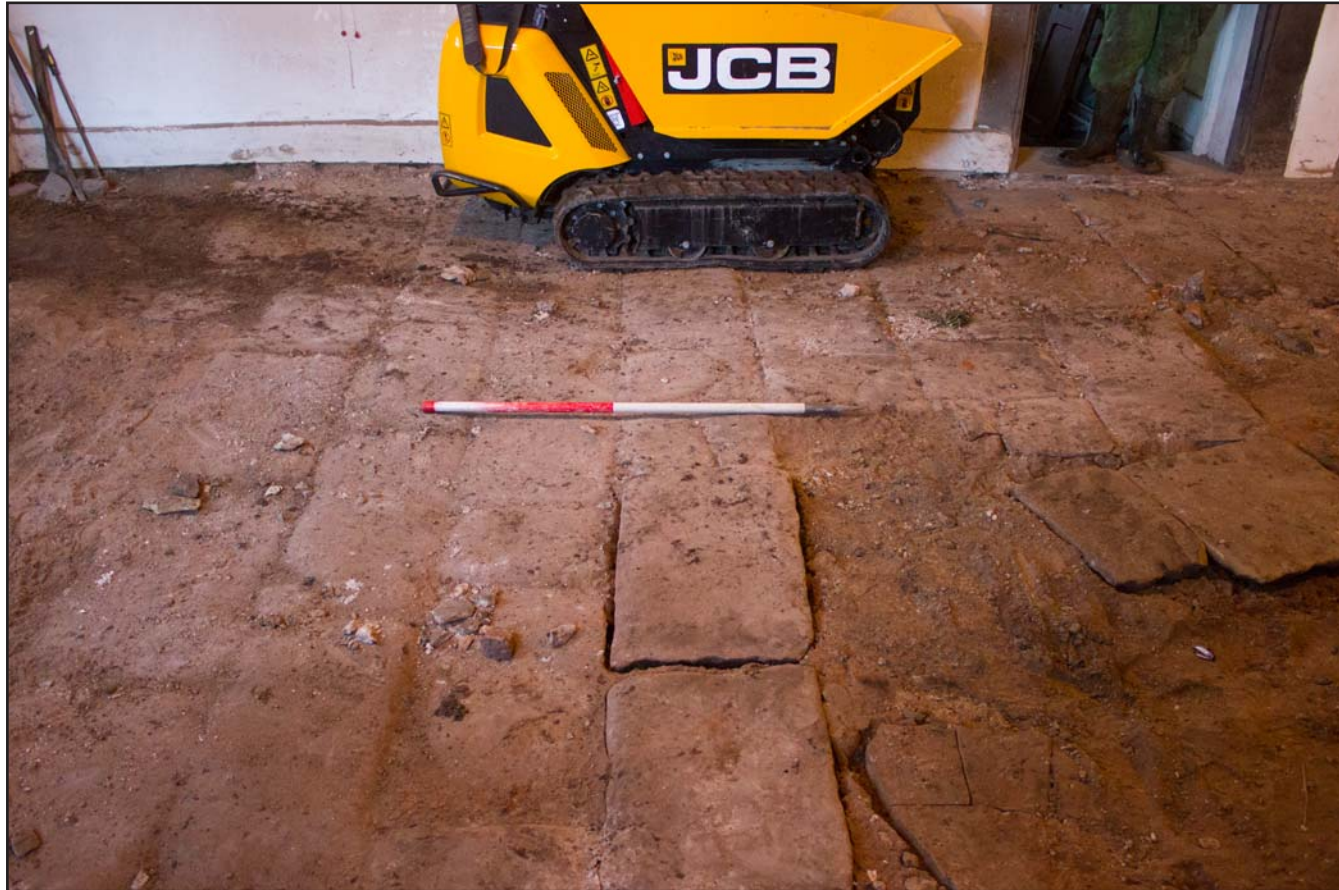
Plate 07: Pre removal of Flagstones in Entrance Hall, Argoed Hall, Mynydd Isa, Mold, Flintshire - from the north - scale 1.00m
