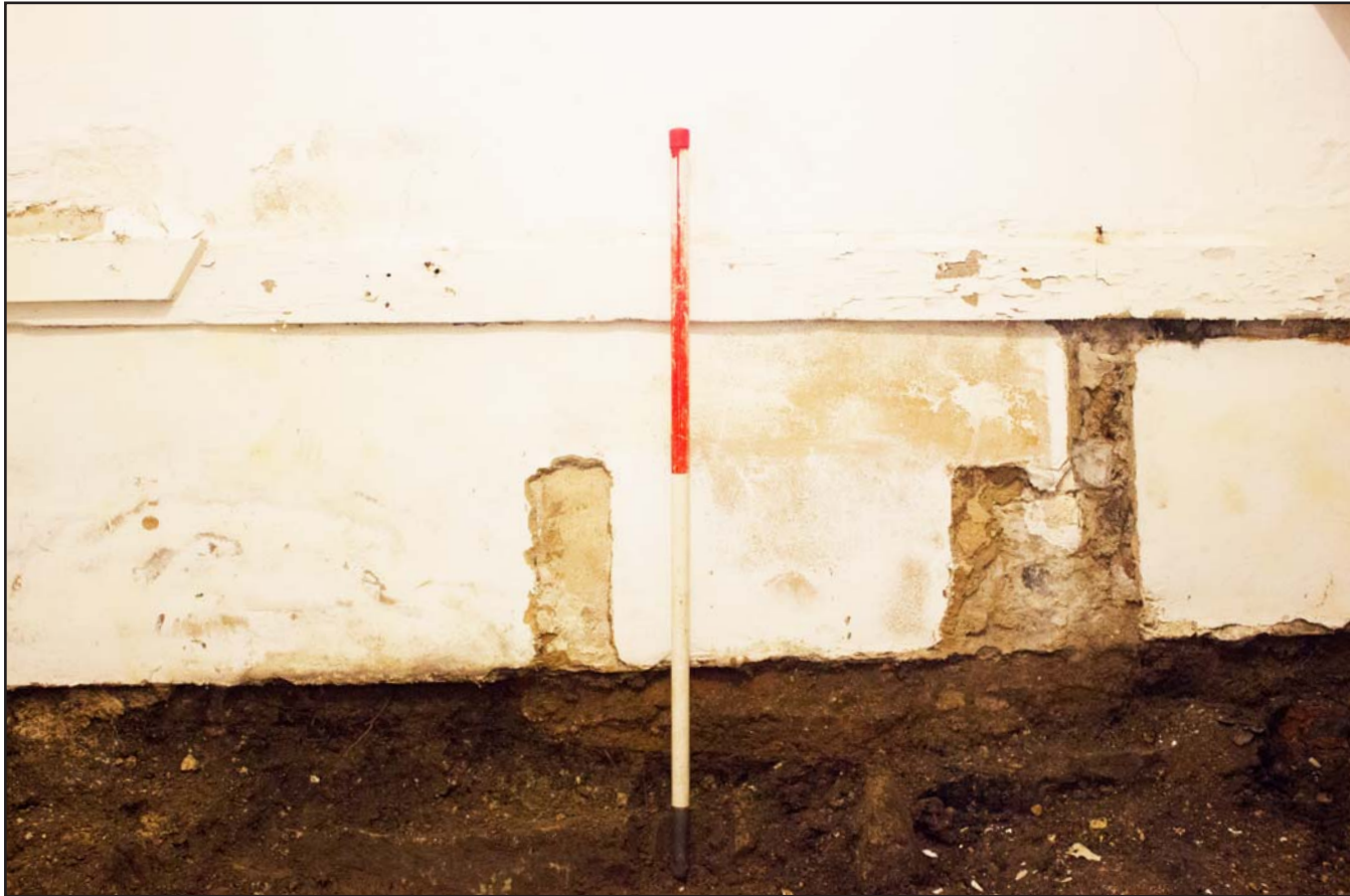
Plate 03: Northern elevation of Pantry, Argoed Hall, Mynydd Isa, Mold, Flintshire - from the south - scale 1.00m
