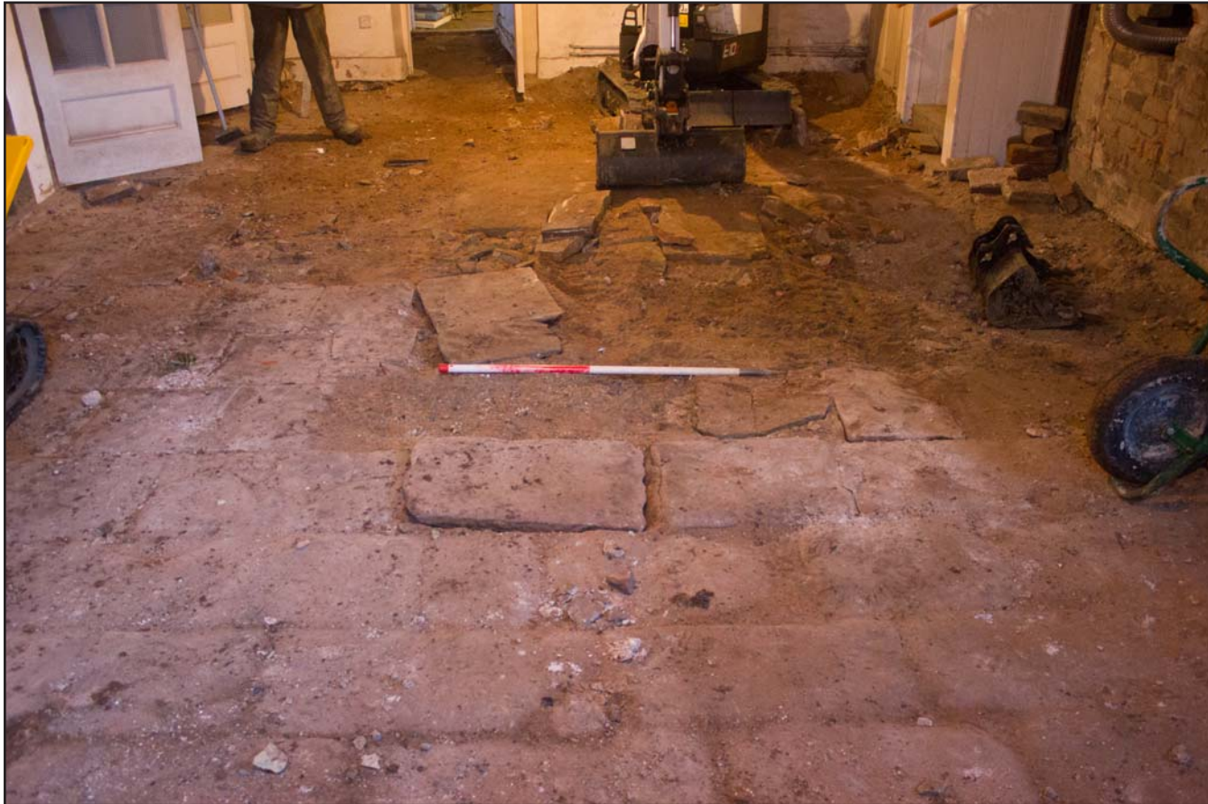
Plate 05: Pre removal of Flagstones in Entrance Hall, Argoed Hall, Mynydd Isa, Mold, Flintshire - from the east - scale 1.00m
