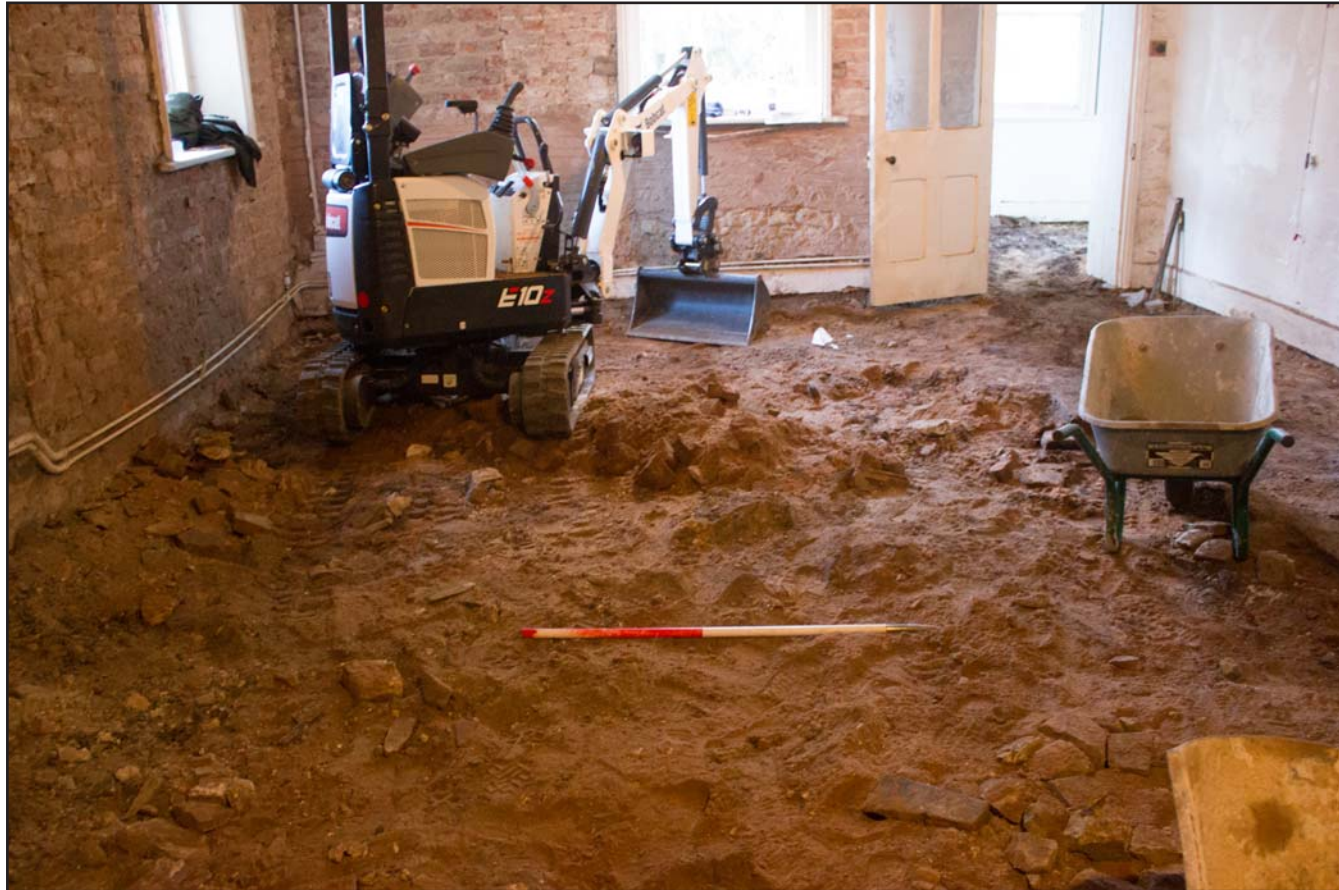
Plate 10: Post removal of Flagstones in Entrance Hall, Argoed Hall, Mynydd Isa, Mold, Flintshire - from the west - scale 1.00m
