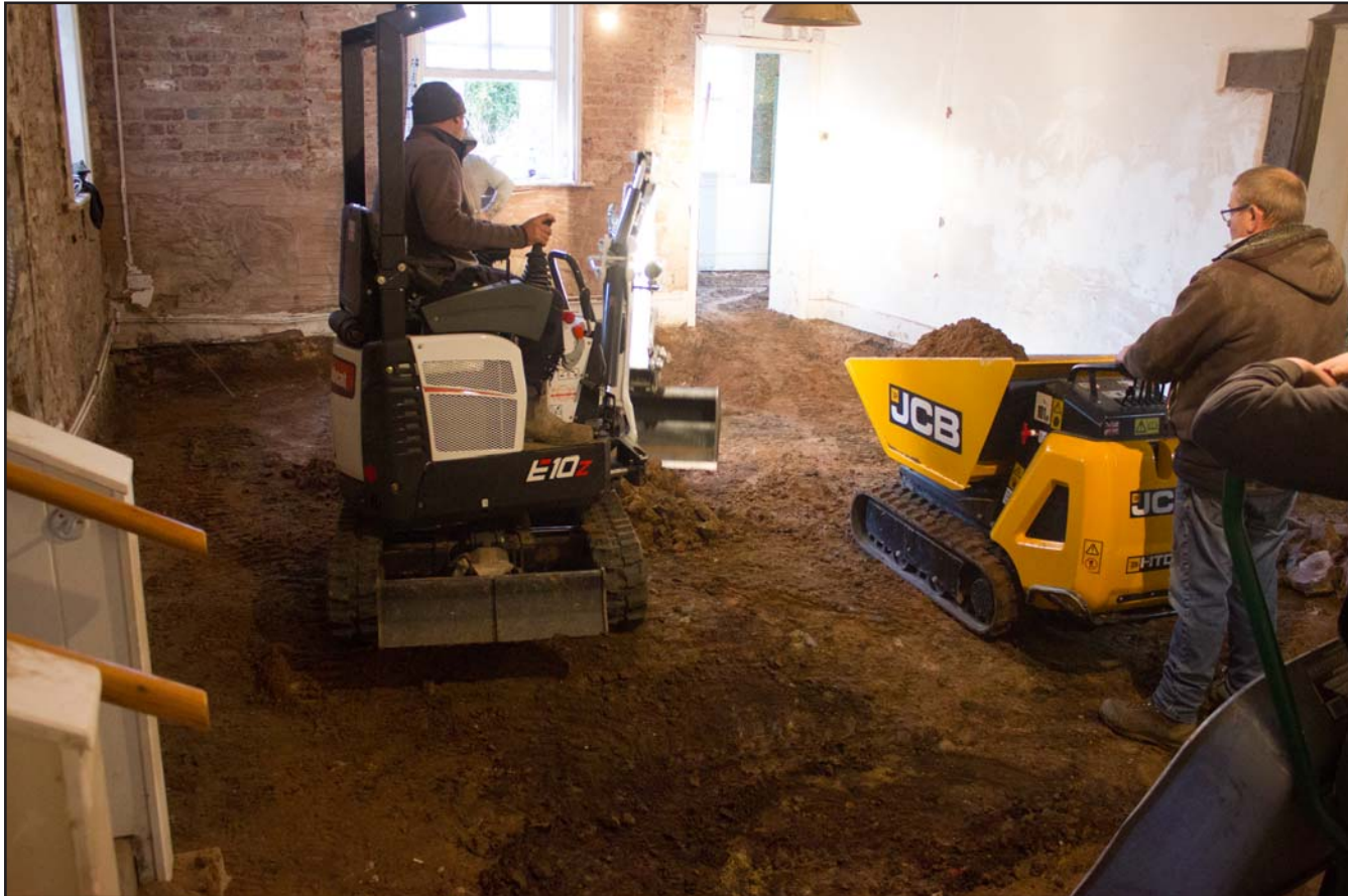
Plate 13: Working shot of ground level within the Entrance Hall, Argoed Hall, Mynydd Isa, Mold, Flintshire - from the northwest - no scale
