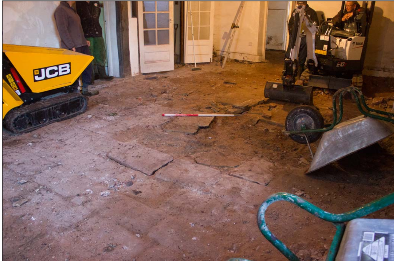
Plate 08: Pre removal of Flagstones in Entrance Hall, Argoed Hall, Mynydd Isa, Mold, Flintshire - from the northeast - scale 1.00m
