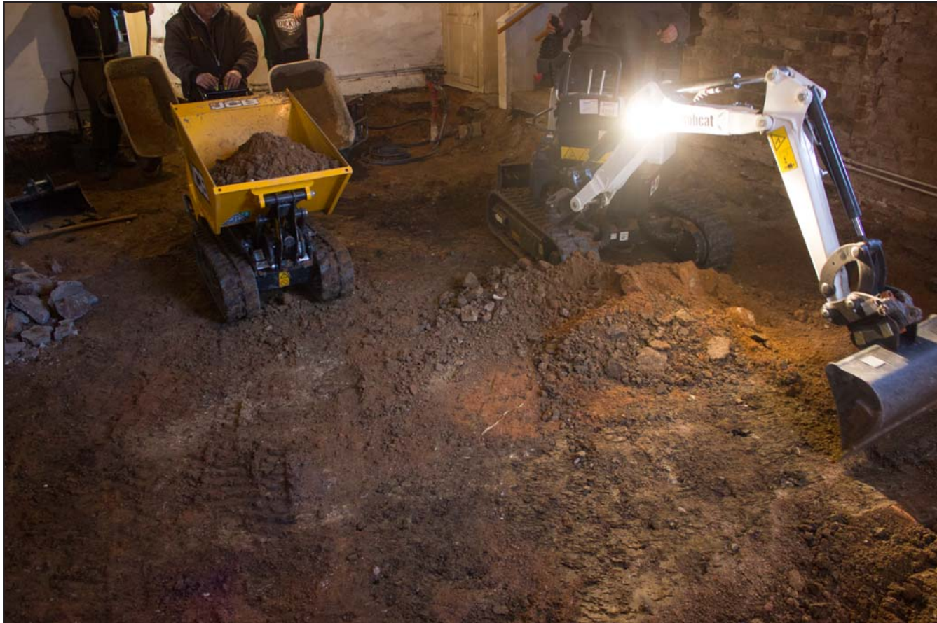
Plate 12: Working shot of ground level within the Entrance Hall, Argoed Hall, Mynydd Isa, Mold, Flintshire - from the southeast - no scale
