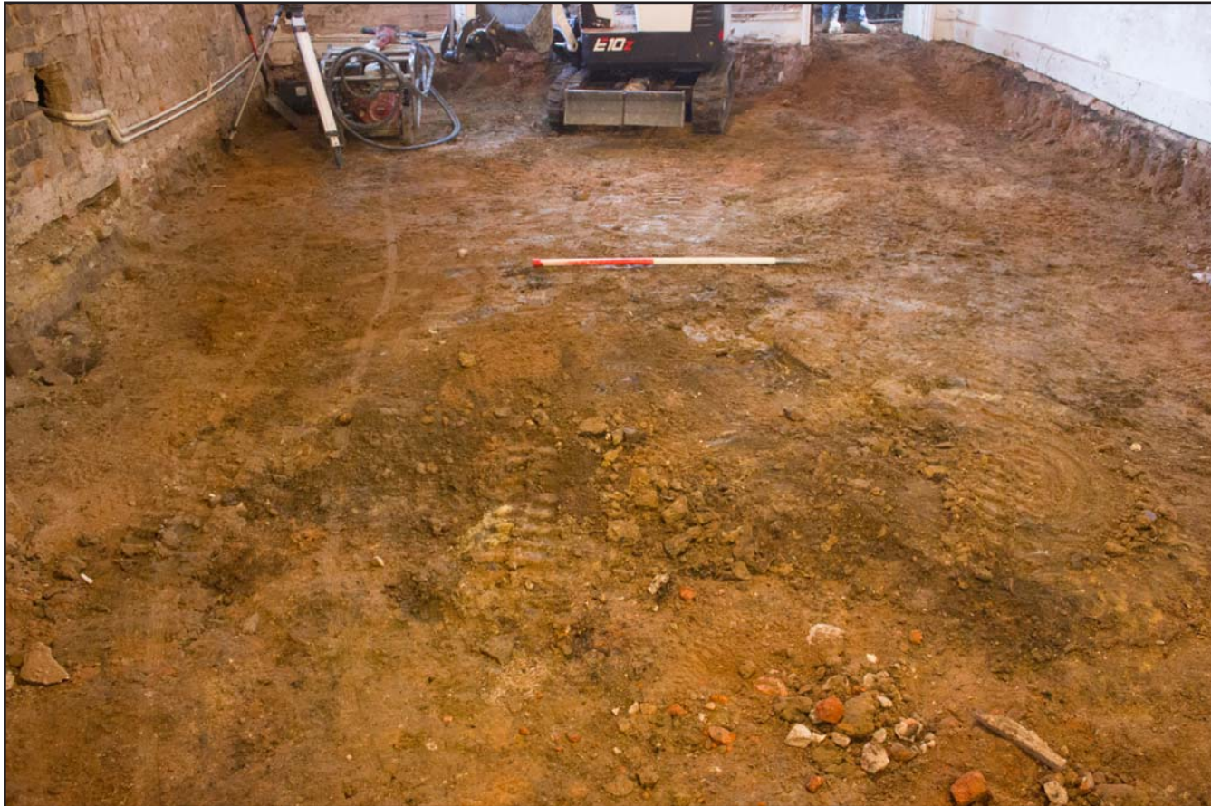
Plate 14: Post excavation shot of Entrance Hall, Argoed Hall, Mynydd Isa, Mold, Flintshire - from the west - scale 1.00m
