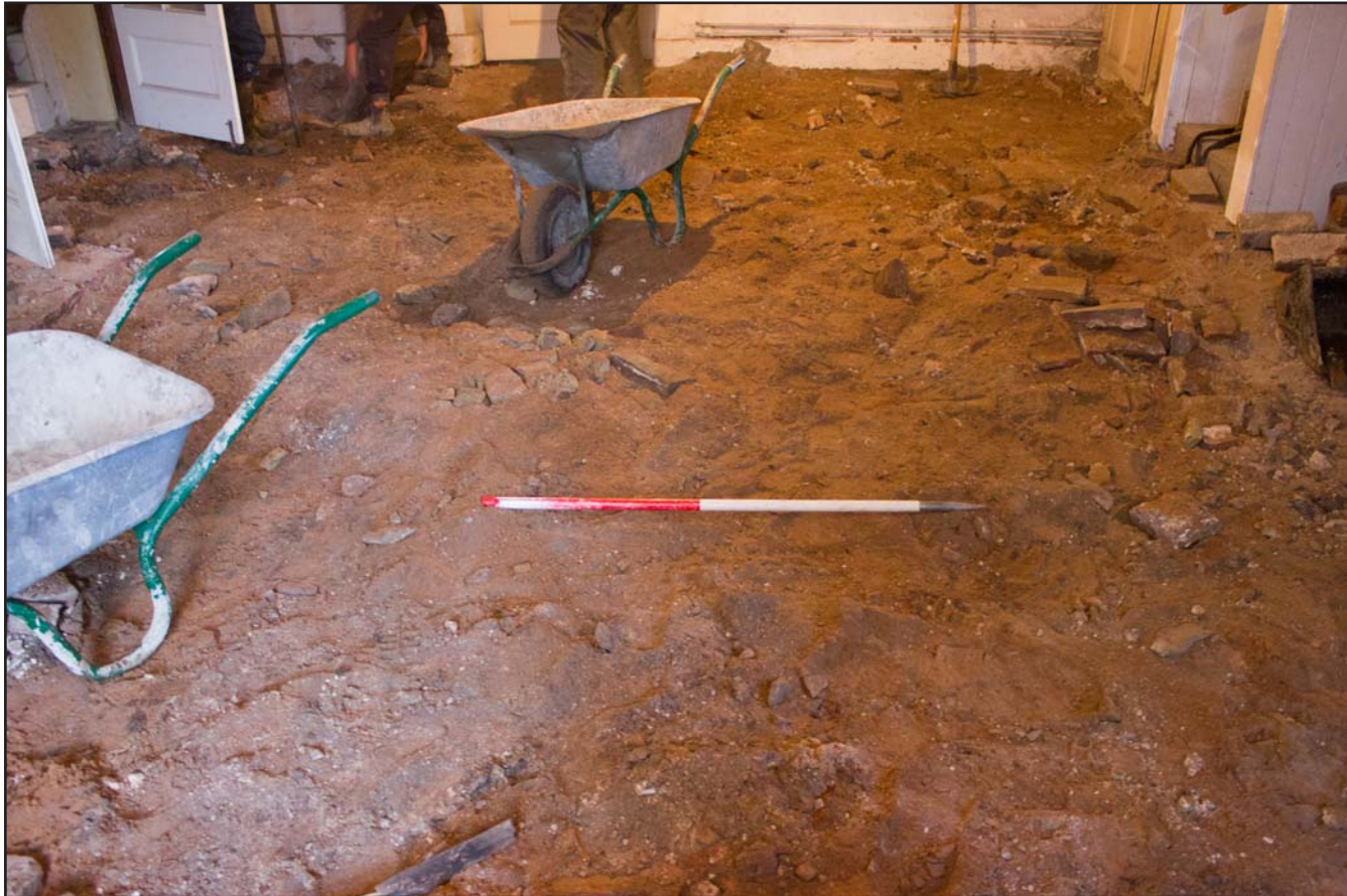
Plate 11: Post removal of Flagstones in Entrance Hall, Argoed Hall, Mynydd Isa, Mold, Flintshire - from the east - scale 1.00m
