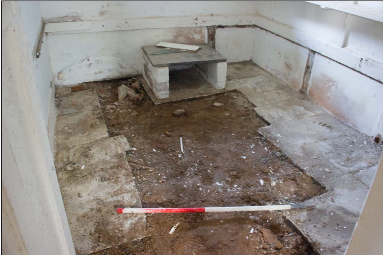
Plate 01: Pre excavation shot of Pantry, Argored Hall, Mynydd Isa, Mold, Flintshire - from the southwest - scale 1.00m
