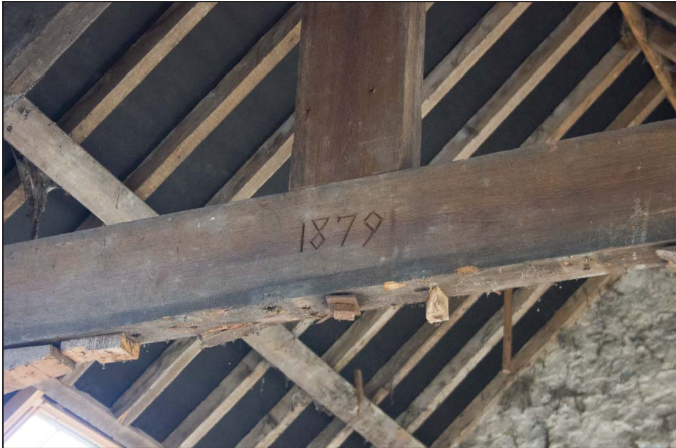
Plate 20: Carved date “1879” on roof truss within Capel Sion, Pontfadog, Llangollen - from the north - no scale
