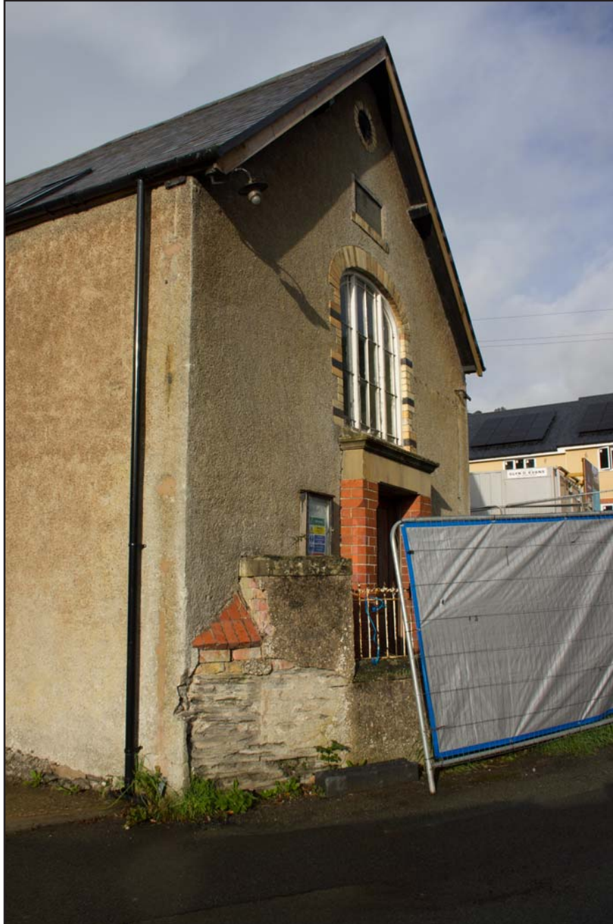
Plate 08: Oblique shot of southeast and northeast external elevations of Capel Sion, Pontfadog, Llangollen - from the east - 1.00m scale
