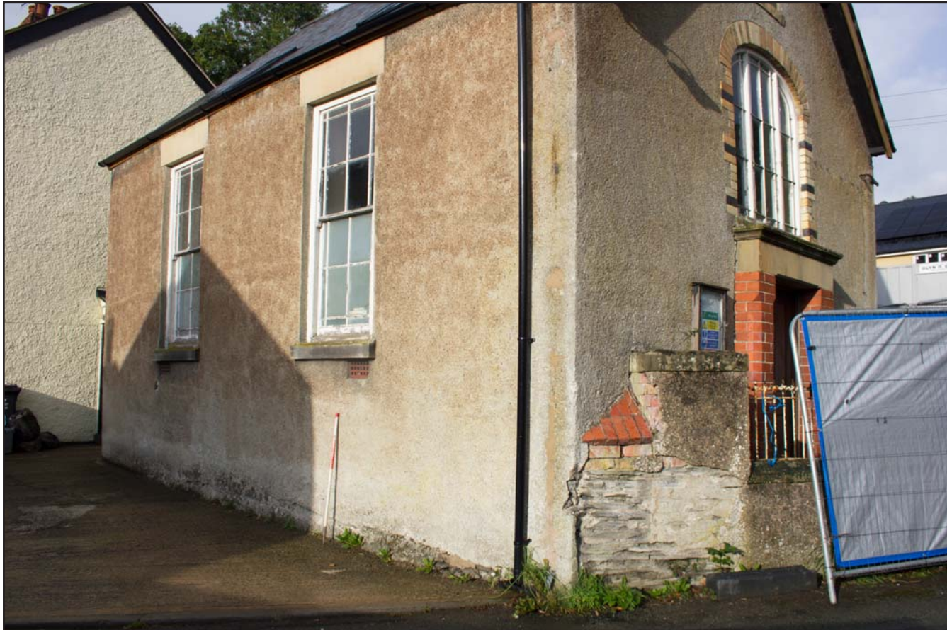
Plate 07: Oblique shot of southeast and northeast external elevations of Capel Sion, Pontfadog, Llangollen - from the east - 1.00m scale
