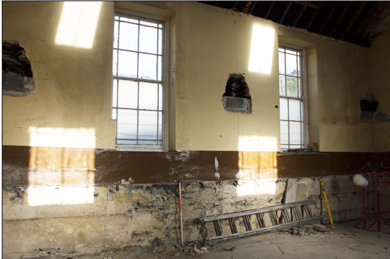
Plate 17: Framed shot of northwest internal elevation of Capel Sion, Pontfadog, Llangollen - from the south - 1.00m scale
