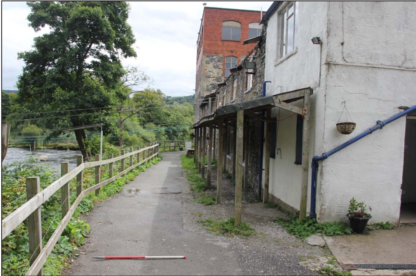
Plate 05: Proposed hydro-scheme route along east side of Mill, from the north. Scale 1.0m.
