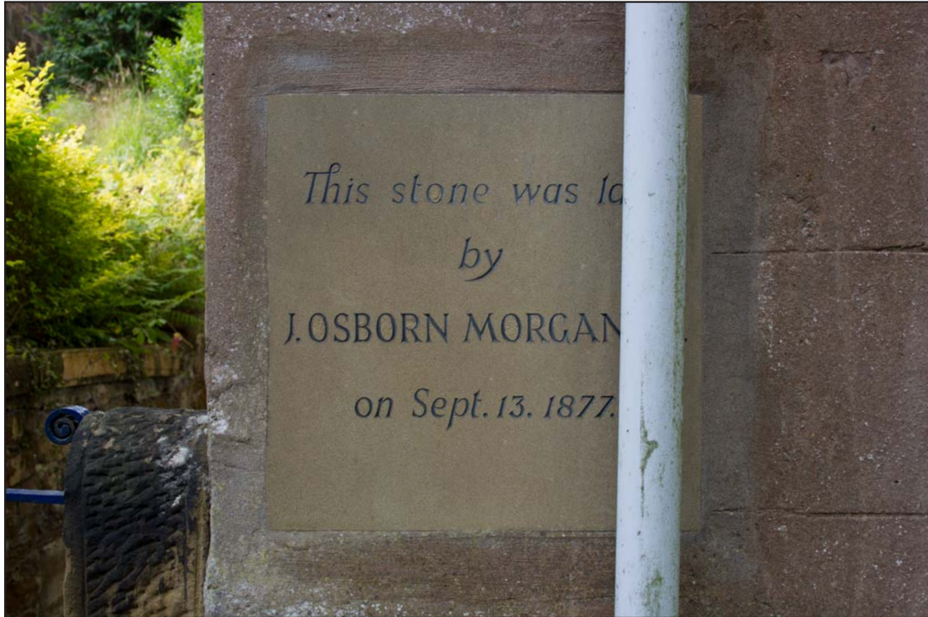
Plate 03: Ffrwd Chapel north facing external elevation showing date stone (east), from the north.
