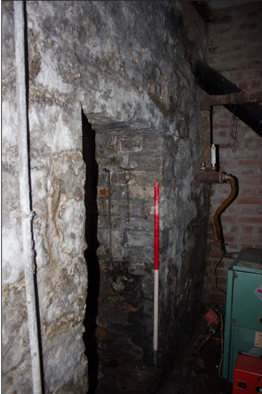
Plate 20: Ffrwd Chapel ground floor Boiler Room showing blocked doorway, from the northeast. Scale 1.0m.
