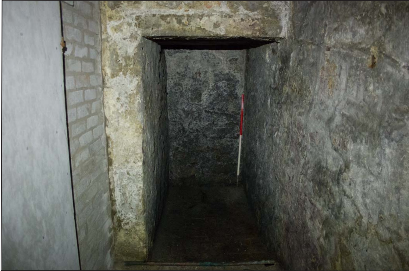
Plate 19: Ffrwd Chapel ground floor Boiler Room showing coal chute, from the west. Scale 1.0m.
