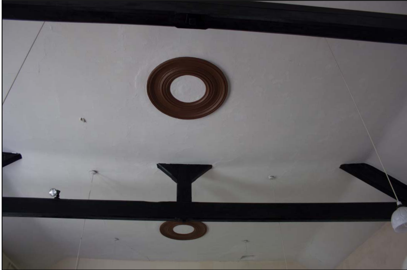
Plate 26: Ffrwd Chapel first floor chapel showing ceiling roses and trusses, from the north.
