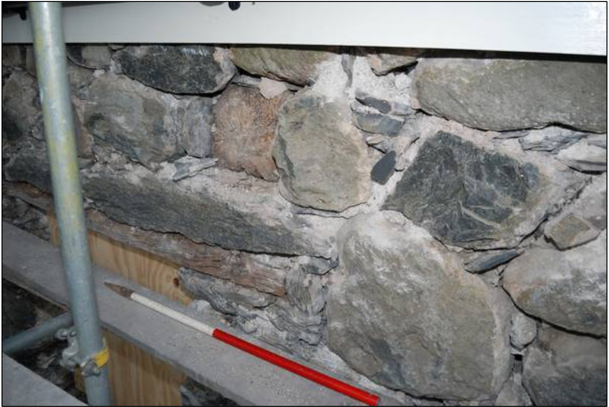
Plate 27: End of a timber above the level of the windows in the “Kitchen Range”
