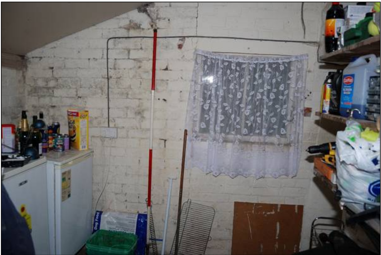
Plate 40: Partially blocked doorway in the scullery
