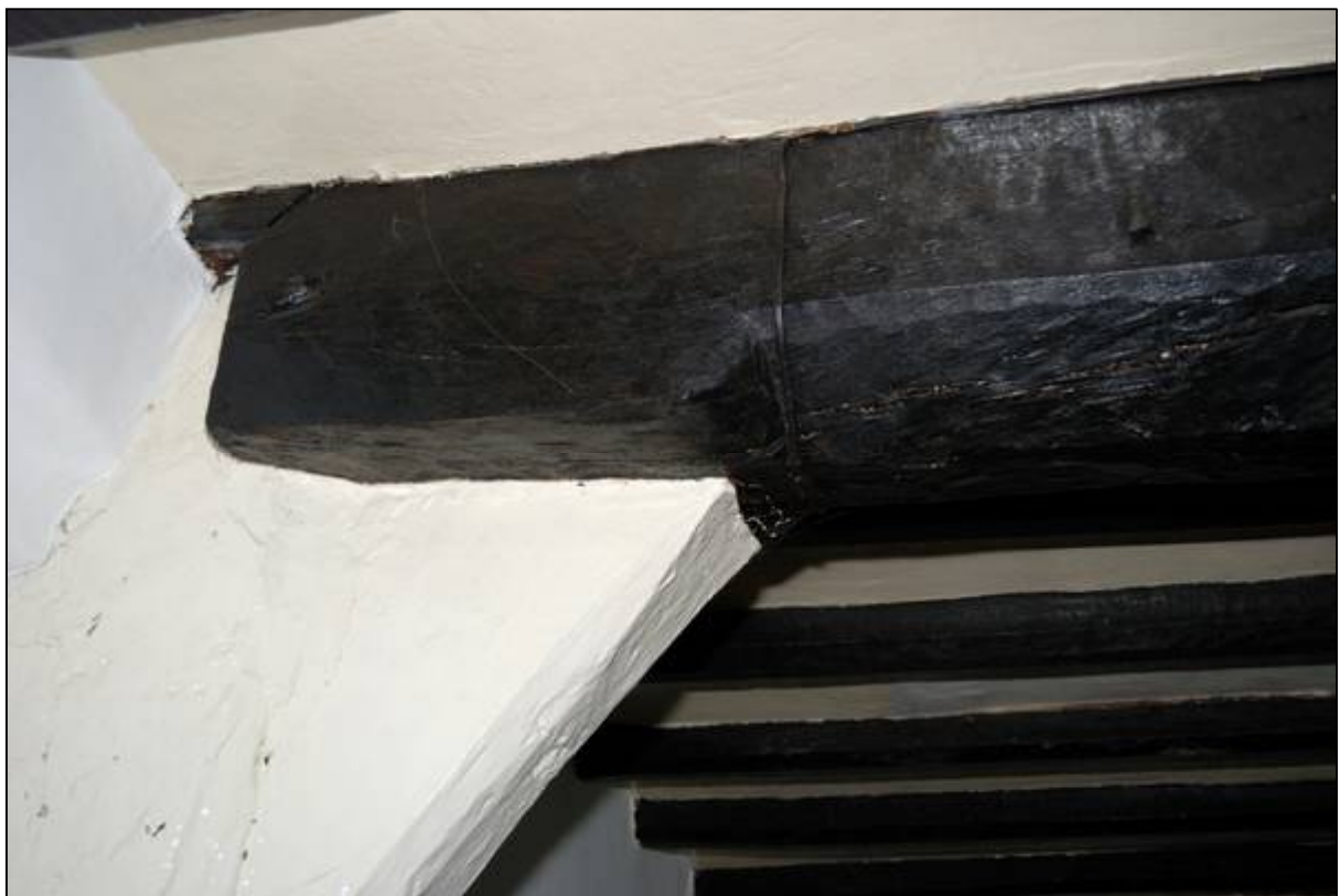
Plate 44: The relationship between the transverse ceiling beam and the post in the hall
