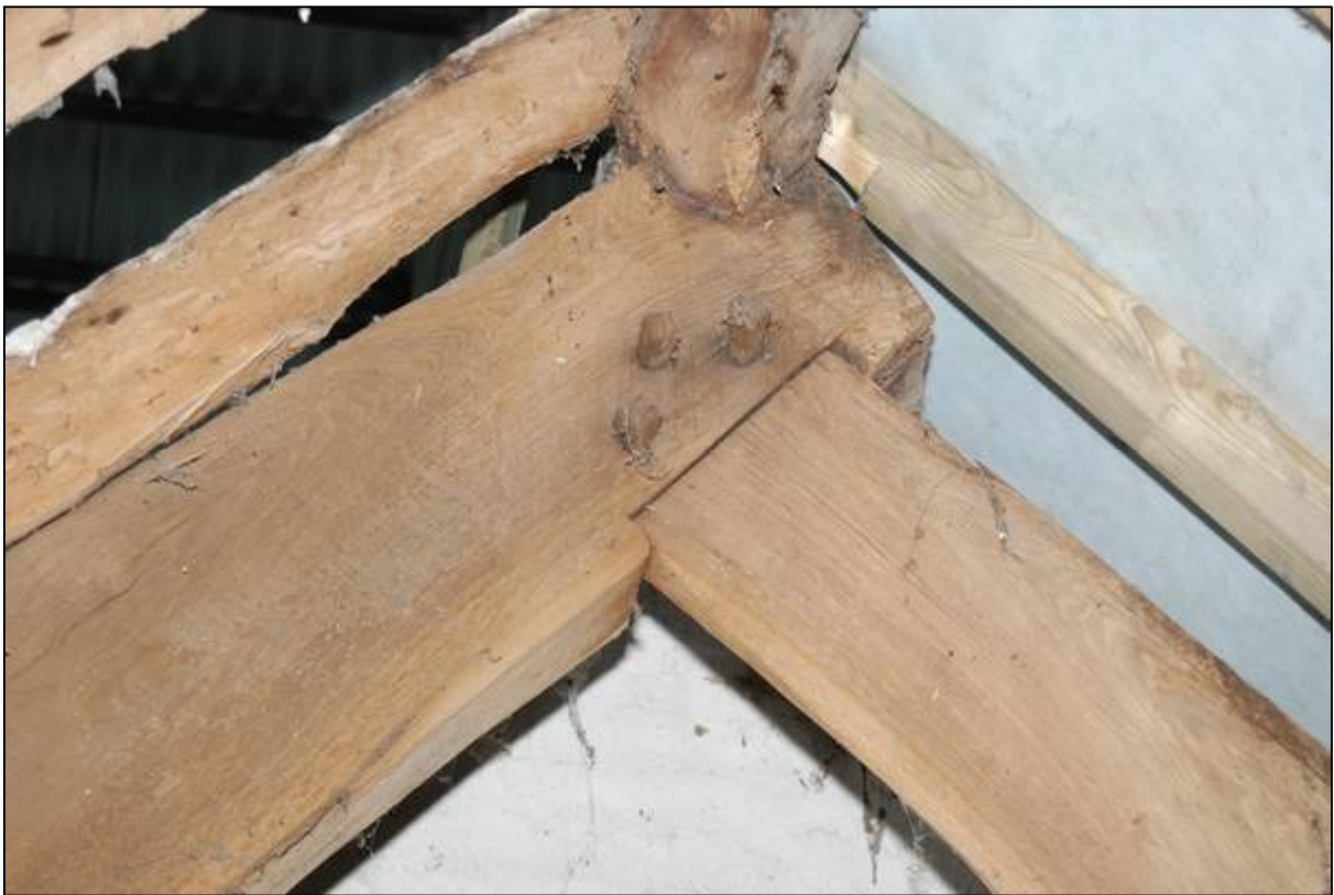
Plate 68: The peak of Truss 2 showing the notch for the ridge piece and the pegged joint between the principle rafters.
