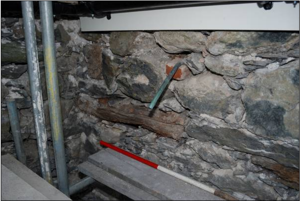
Plate 25: Detail of the lintel for the blocked window in the “Kitchen Range”
