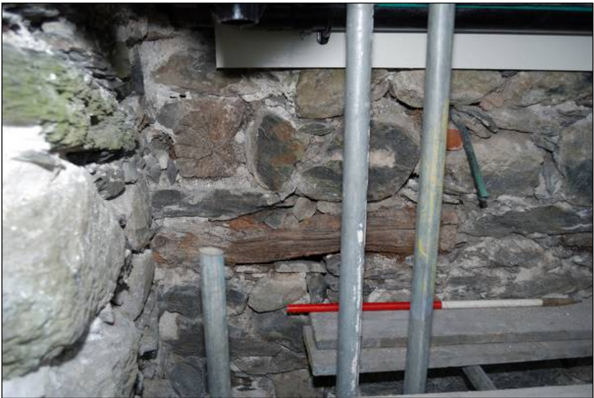
Plate 26: End of a timber above the level of the windows in the “Kitchen Range”
