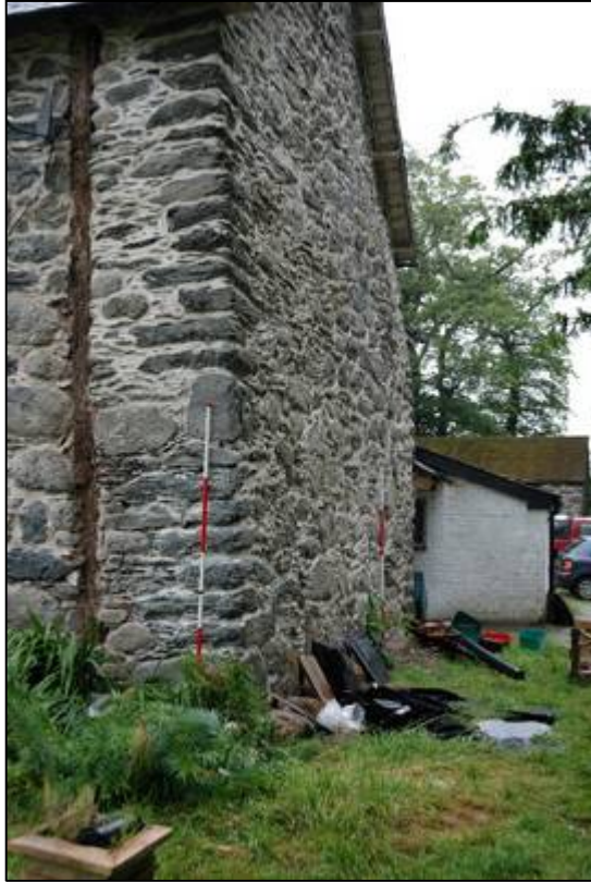
Plate 21: Bulge in the northern gable end of the main range
