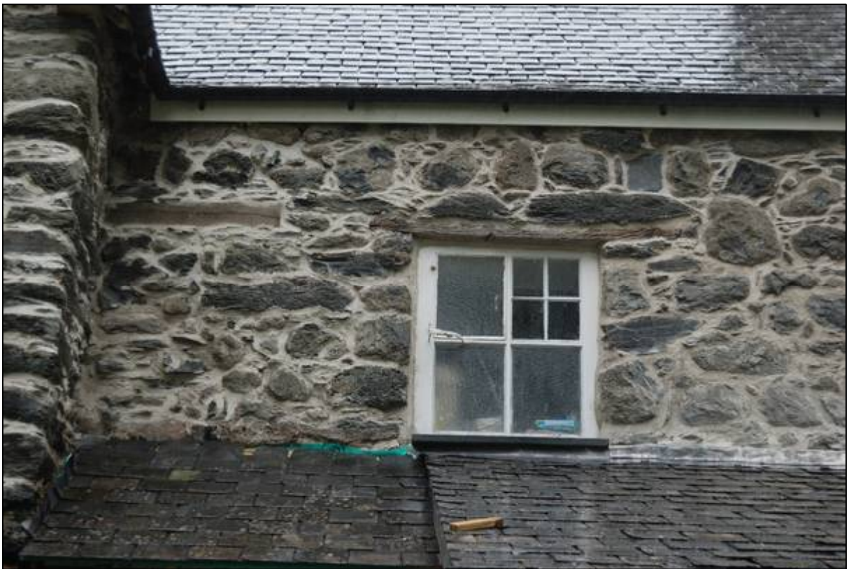
Plate 24: Lintel for the blocked window in the northern face of the “Kitchen Range”
