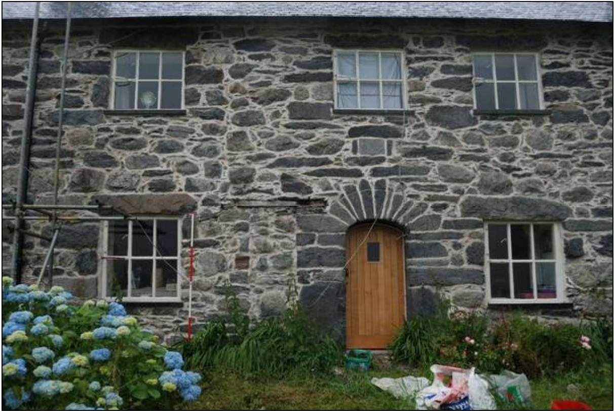
Plate 19: Break in the stonework on the front elevation
