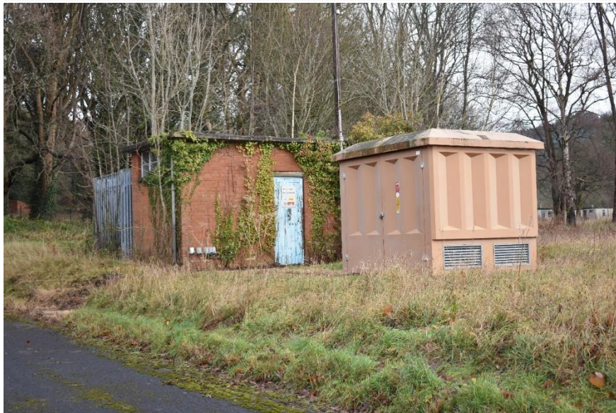
Fig. 27 Building 13 –Intake Switch Room, Phase 3. Photo CPAT 4720-0031
