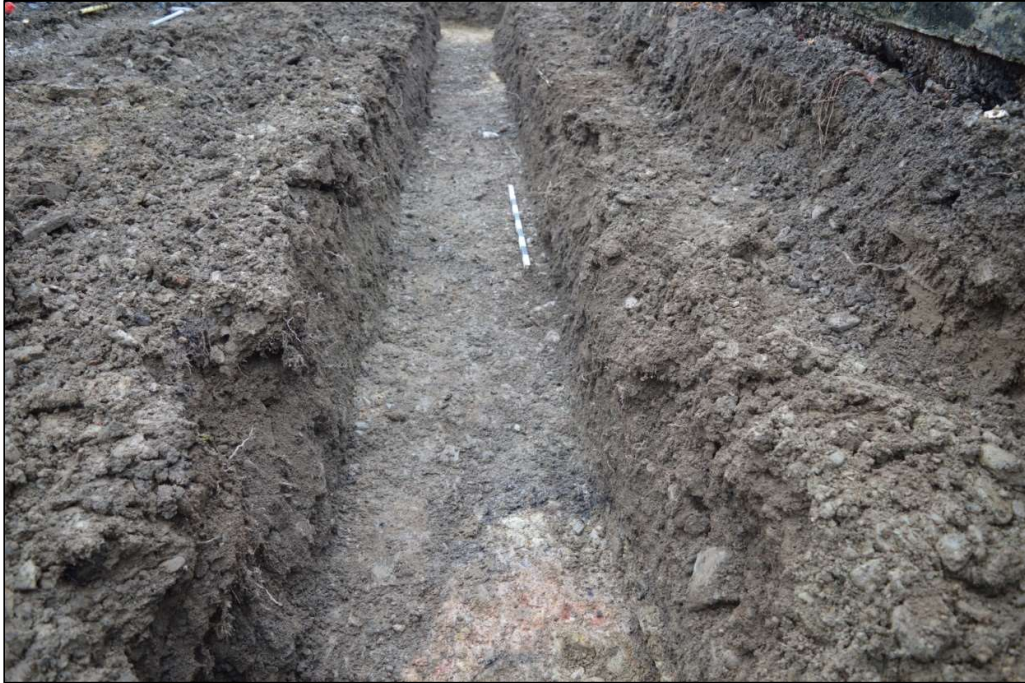
Fig. 4: Foundation trench from north-east, showing the heated clay (7) in the foreground overlain by dark grey silt (5), both of which were cut by the later service trench (4). CPAT 4850-0008
