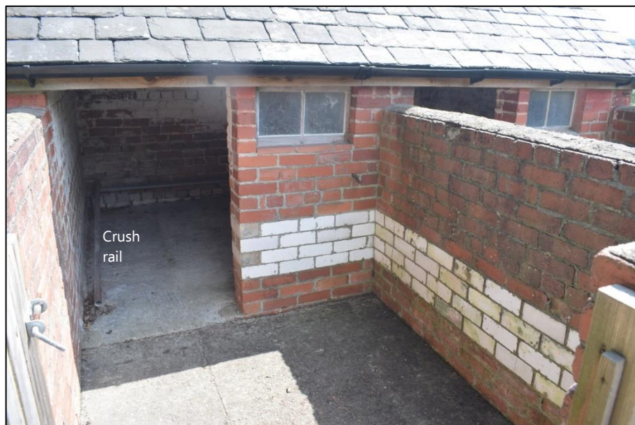
Fig. 3 Central box of the pigsty showing crush rail and mixture of brick types used in the construction Photo CPAT 4935-007
