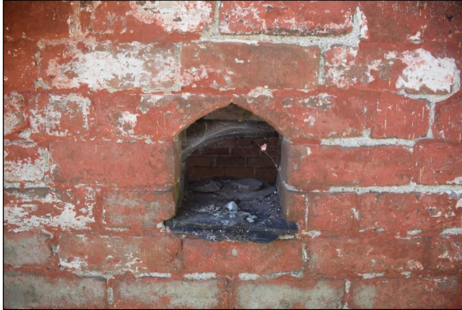
Fig. 3 Ventilator in north gable end Photo CPAT 4935-005
