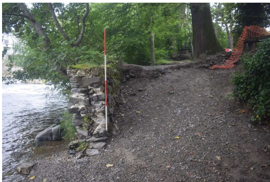
Fig. 12 Exposed cross section through the revetment viewed from the east Photo CPAT 4948-002
