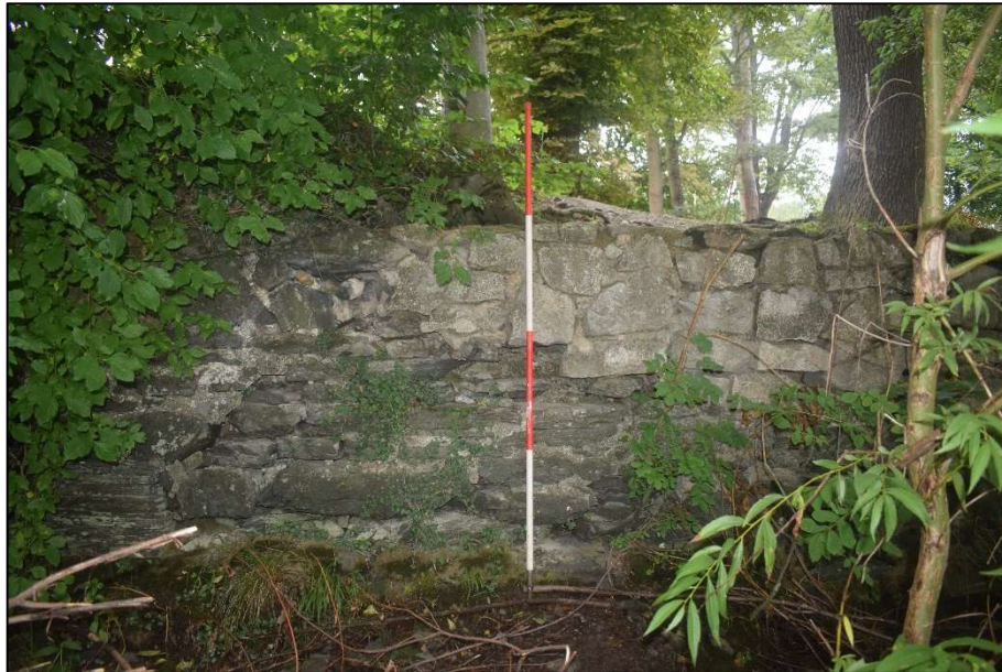
Fig. 11 Western visible extent of the revetment showing the difference in stonework between the upper and lower structure Photo CPAT 4948-032
