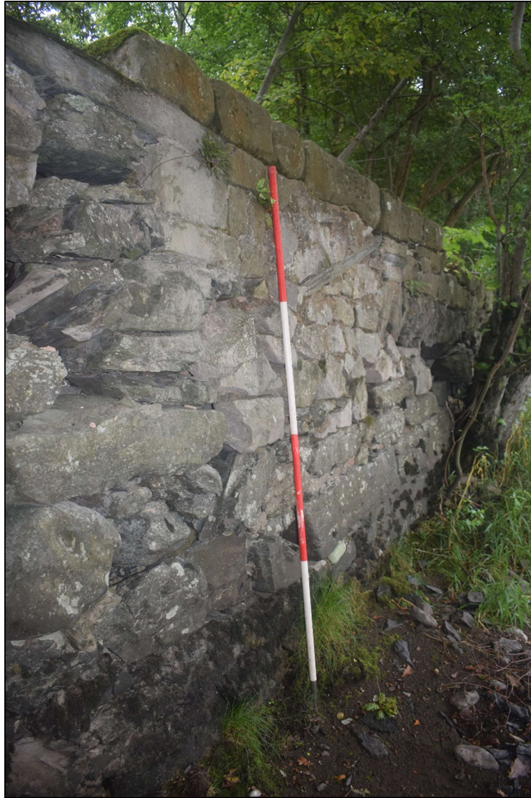
Fig. 13 View from the west along the revetment showing the batter on the lower structure Photo CPAT 4948-034
