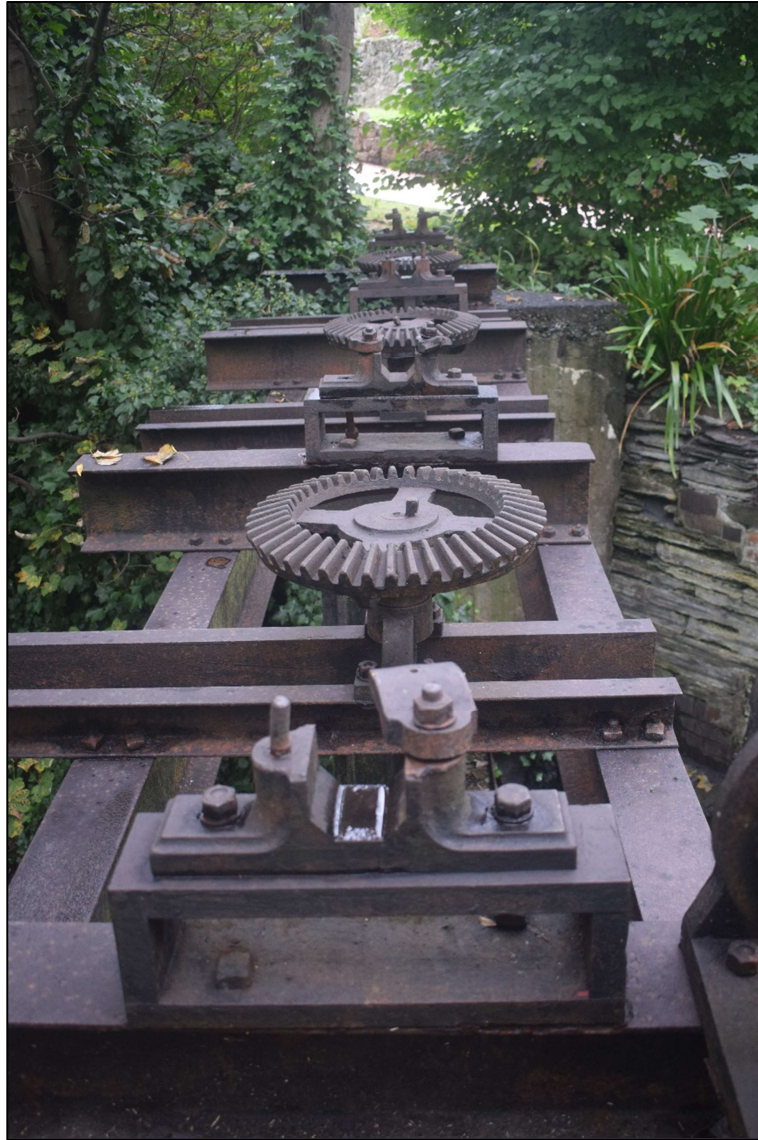
Fig. 10 Detail of the winding gear for the sluice gate Photo CPAT 4948-010
