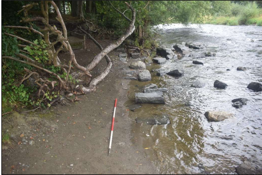
Fig. 14 View east showing the line of the revetment visible as a partially buried foundation Photo CPAT 4948-035
