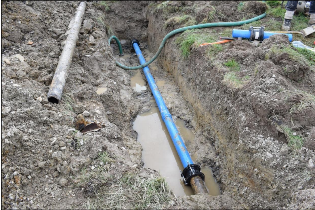
Fig. 3: The final excavation, showing the replacement pipe, from the north-east. Photo CPAT 4782-0008
