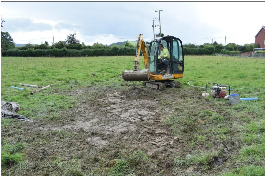
Fig. 5: The area of the leak following its reinstatement. Photo CPAT 4782-0010
