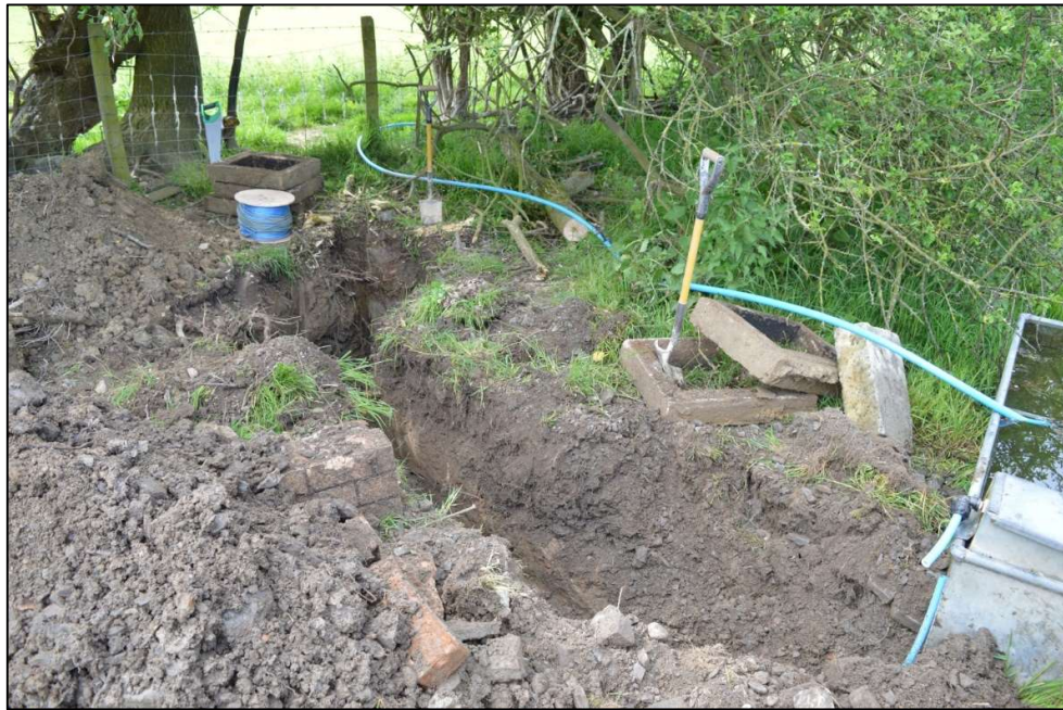
Fig. 5: Excavation No 5, at the north end of the main, showing the connecting trench to the stock water supply, from the north. CPAT 4927-0008
