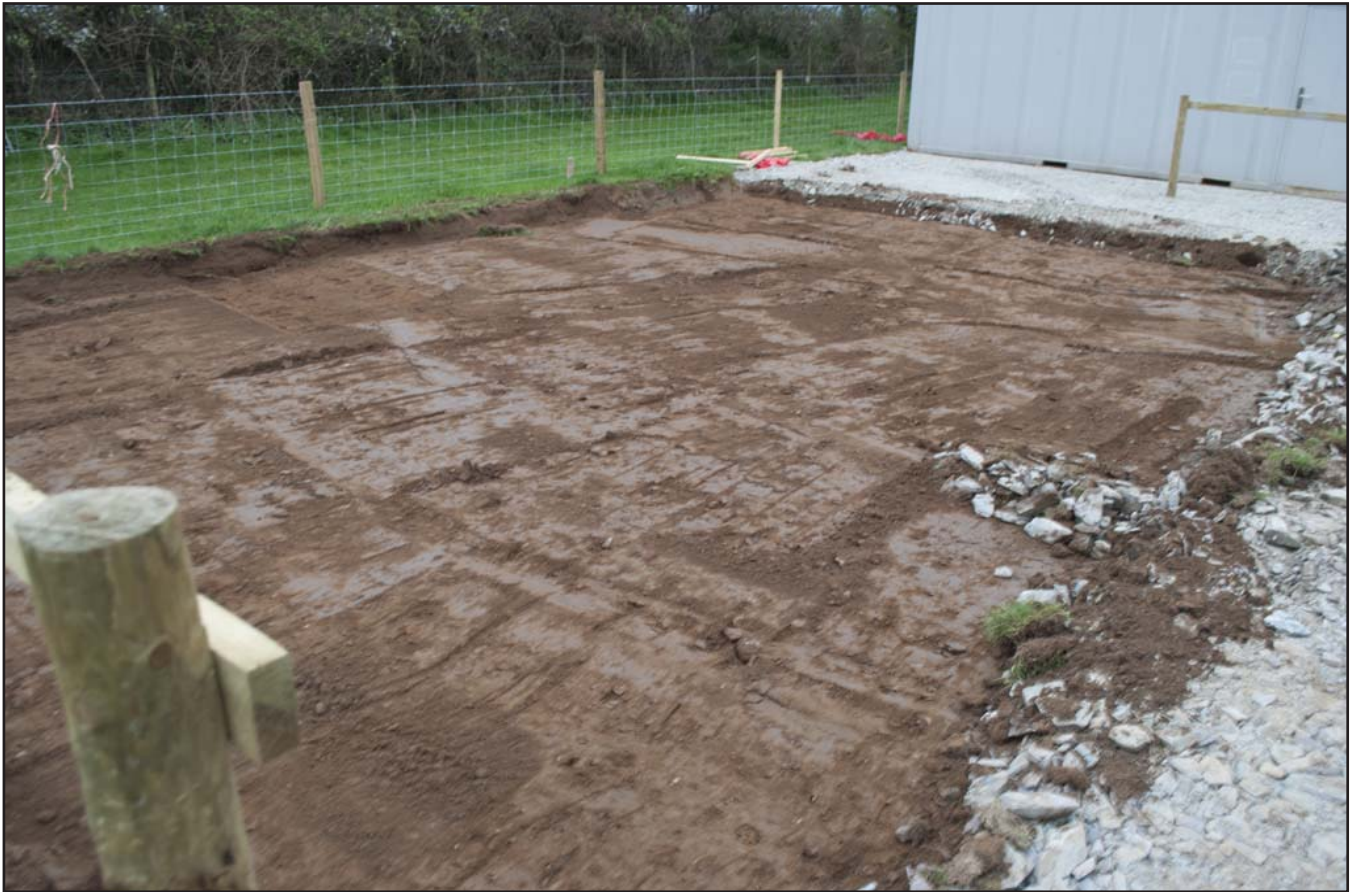
Plate 5: View of topsoil strip on the corner of the compound area - no possibility of seeing the archaeology; scale 1x1m; view from NE (archive reference: G2716_005).
