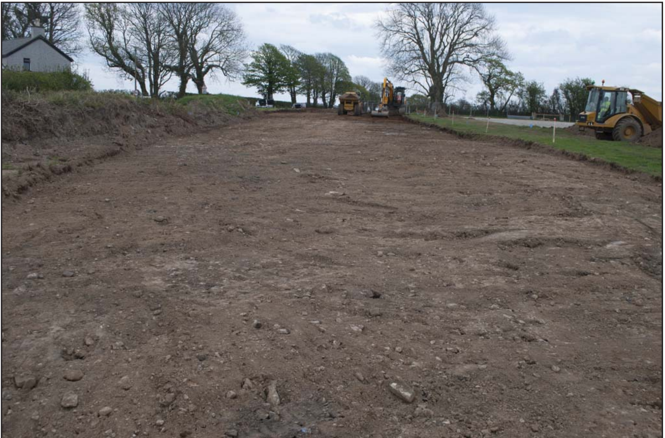
Plate 10: General view of the stripped area; scale not used; view from N (archive reference: G2716_010).
