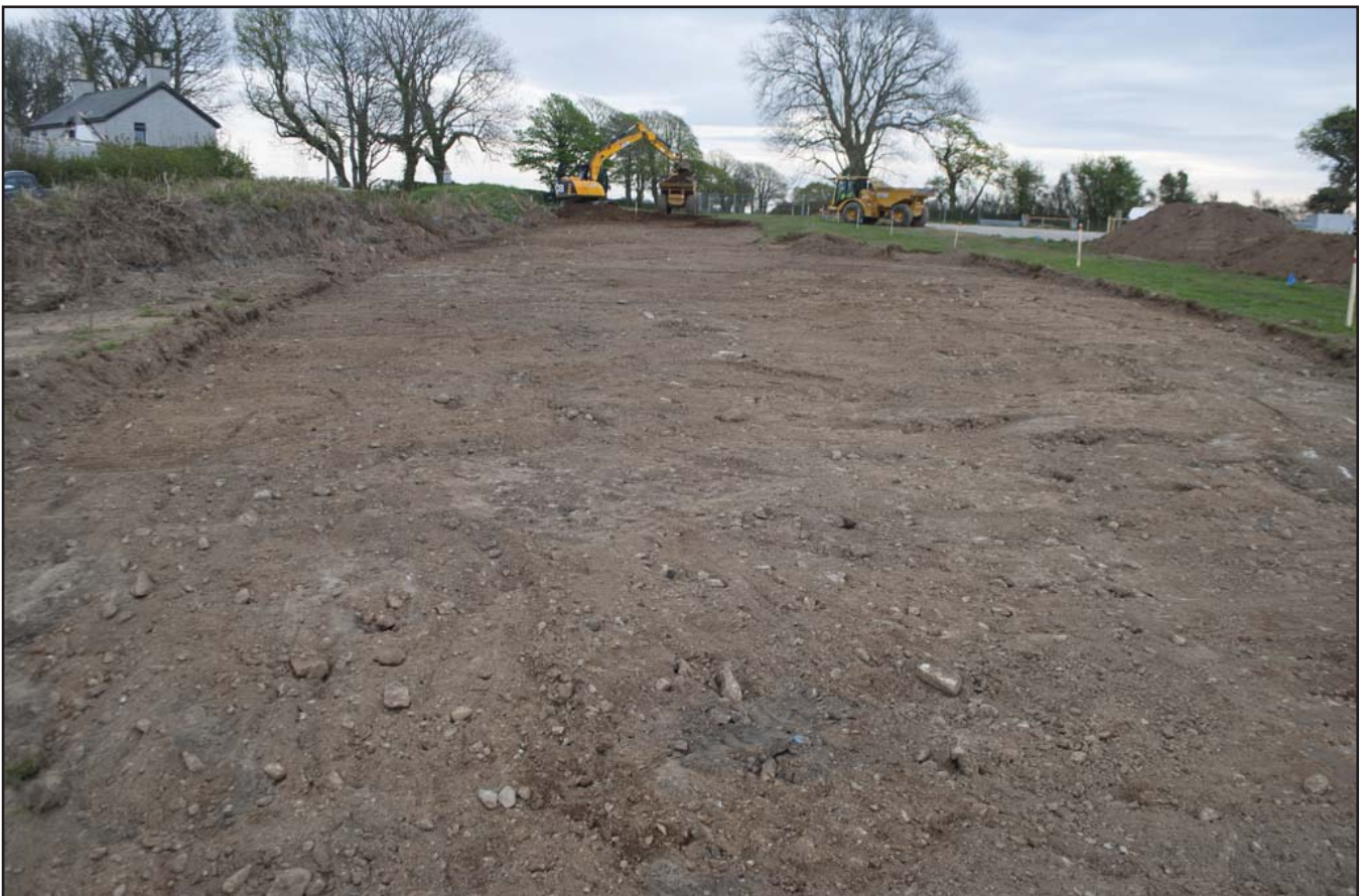
Plate 6: General view of the topsoil strip; scale 1x1m; view from N (archive reference: G2716_007).
