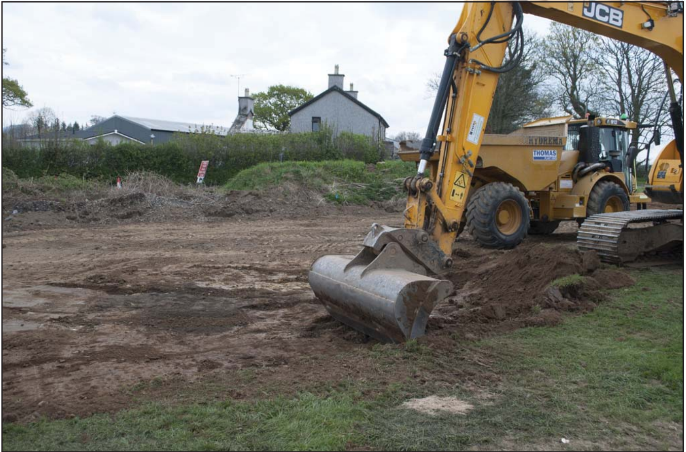
Plate 9: General working shot showing topsoil stripping; scale not used; view from NW (archive reference: G2716_009).
