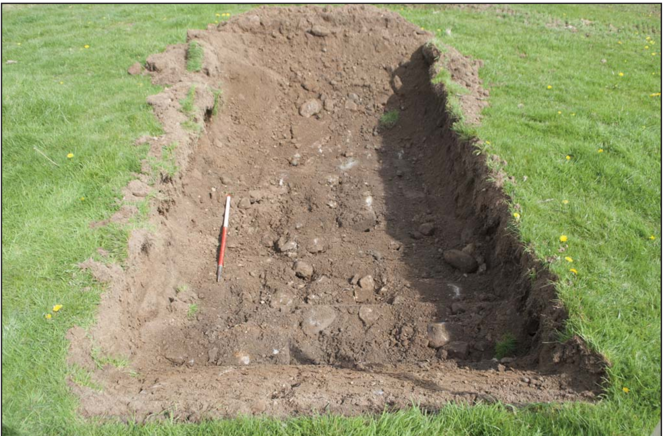
Plate 2: Topsoil removal over the mill race (PRN 90074; Feature 2); scale 1x1m; view from SW (archive reference: G2716_002).
